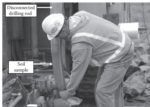
FIGURE 4.14 Extracting a sample from a Roto-sonic drilling rod. (Photo by Daniel T. Rogers.)
