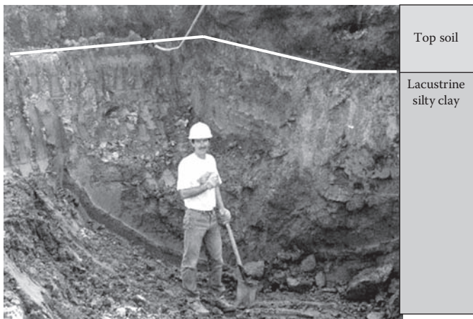
FIGURE 5.4 Excavation at a construction site exposing geologic strata. (Photo by Daniel T. Rogers.)
