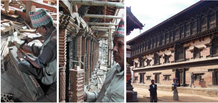
Fig. 5.10 55-Window Palace during and after renovation: ( left ) Craftsman carving lattice window, 2006; ( middle ) senior craftsman presenting carvings in upper storey during renovation phase, 2007; ( right ) after the renovation, 2011
