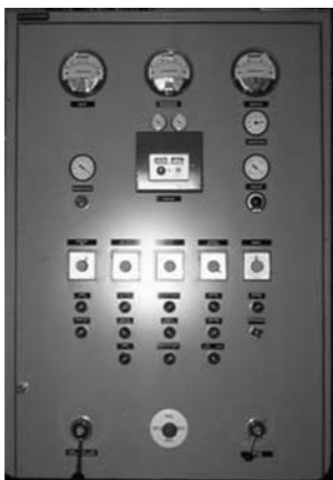
Figure 22 Pneumatic control panel. Source: Courtesy of The Glatt Group.
