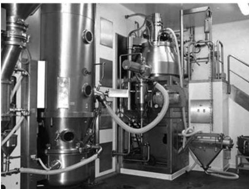
Figure 38 Loading of fluid bed from high shear mixer. Source: Courtesy of The Glatt Group.
