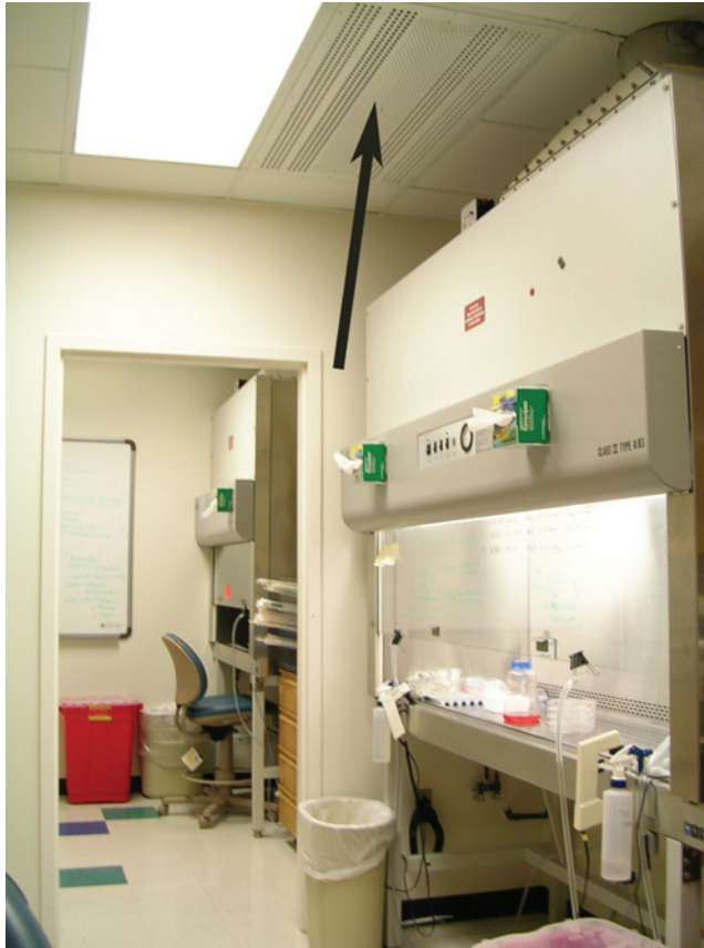
FIGURE 26.3 The air handling system of the cell culture rooms are HEPA-filtered (arrow) and maintain positive pressure with respect to adjacent non-cell culture areas.
