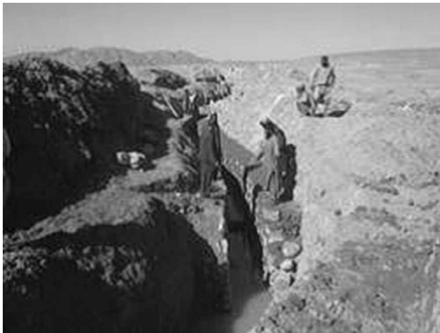
FIGURE 22.3 Karez canals require maintenance (Photo http://www.afghanistan.gc.ca ).
