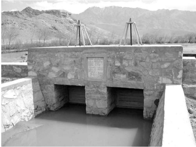
FIGURE 22.6 A typical gate fitted canal intake.
