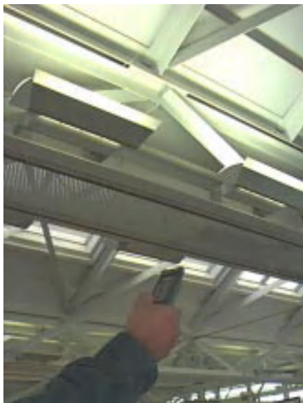
Figure 9: The ambient lighting system in the Intelligent Workplace incorporates user-controlled indirect luminaires that have T-8 fluorescent fixtures with electronic ballasts to support daylight-based dimming.
