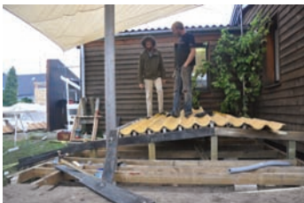
Figure 5.19 The front edge that descended into the water was constructed and then unconstructed and stored for the final phase of installation
