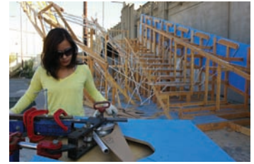
Figure 17.13 Pendulum Plane . A wood jig ensured accurate overall geometry of each piece during assembly. The jig held each piece in place to aid in welding each of the 16 units together. The design required the fabrication of two jigs, one a mirrored version of the other
