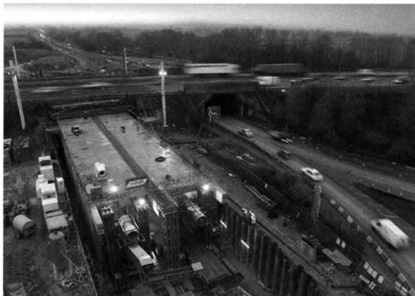
Figure 20, Rear view of the vehicular underbridge during installation, Junction 15A, M1 Motorway, Northampton.
