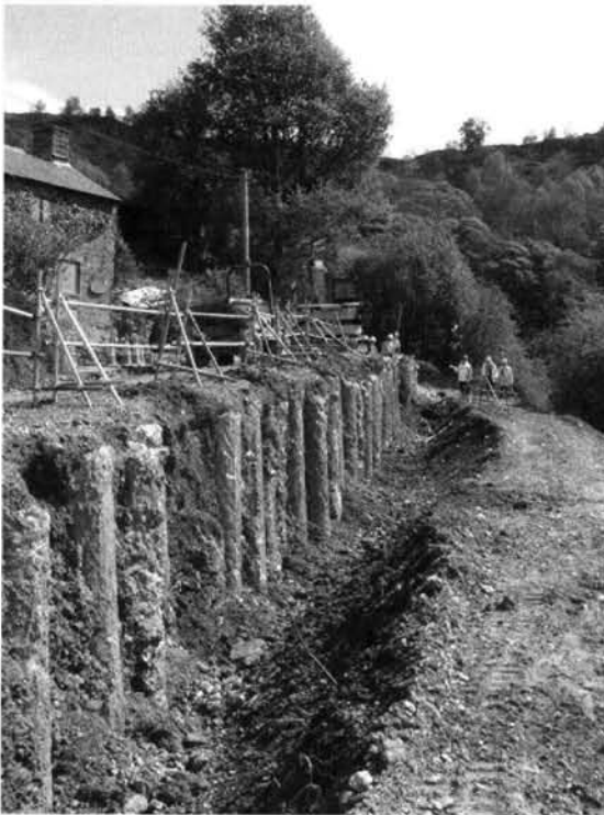
Figure 11, Deep seated failure and repair
