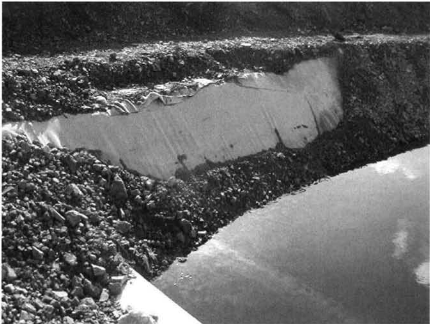
Figure 6, Slip of cover soil on steep barrier covered slope
