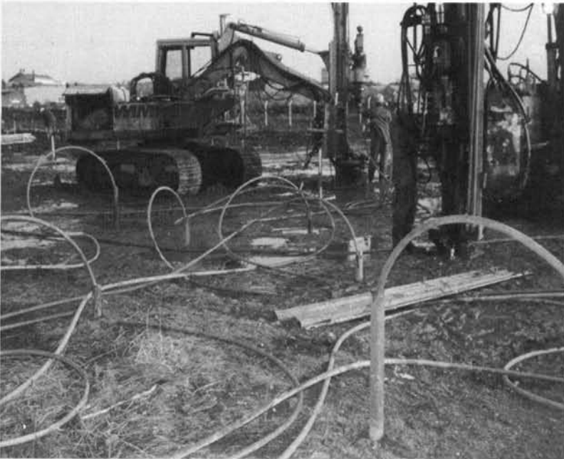
Figure 13, Mining subsidence and repair
