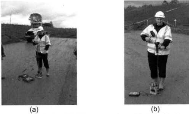
Plate 4, In-situ testing during HBFM construction with (a) Light Dynamic Plate, and (b) Cone Penetrometer
