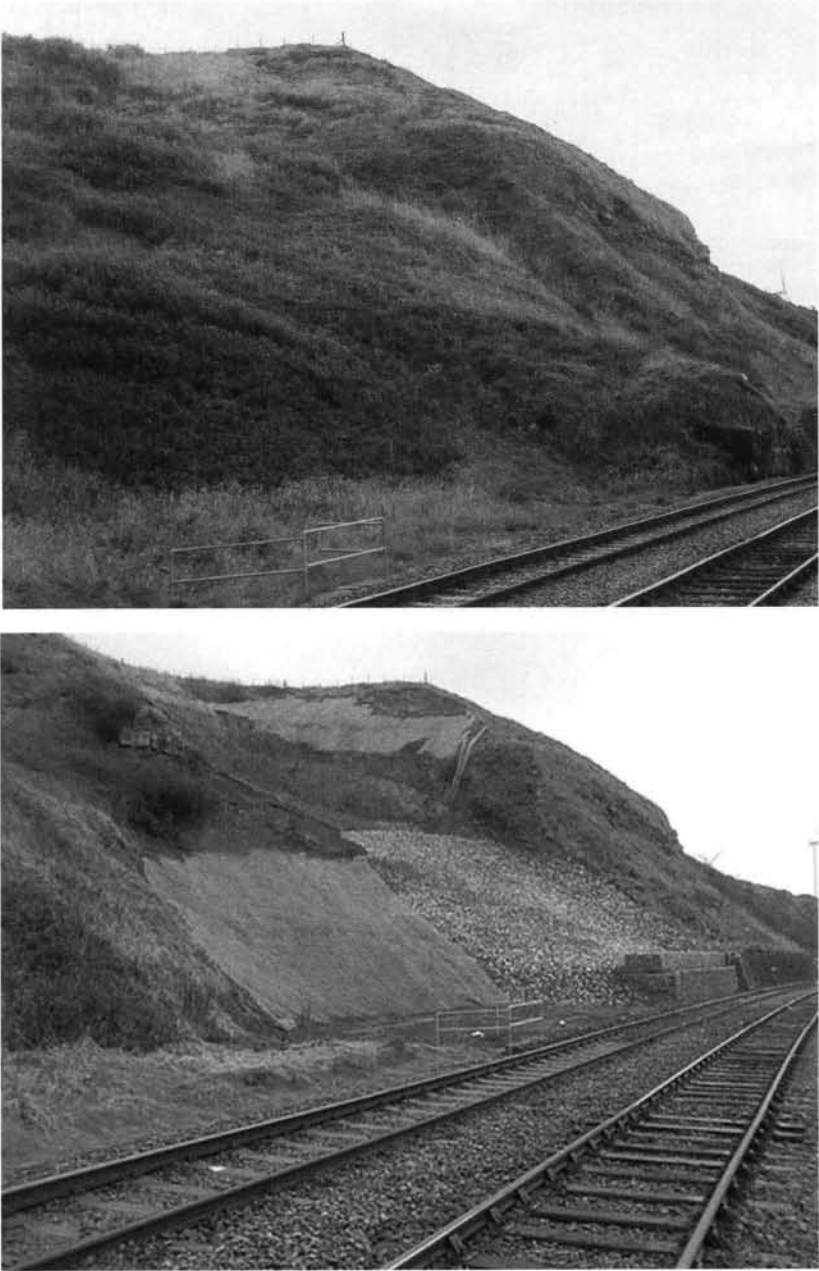
Figure 12, Debris flow failure and repair
