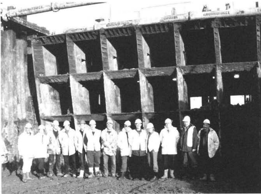
Figure 21, Cellular shield and team on completion of tunnelling, Junction 15A, M1 Motorway, Northampton
