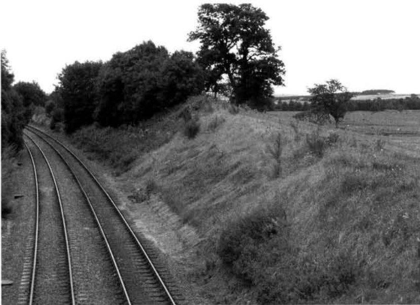
Figure 15, Animal damage and repair
