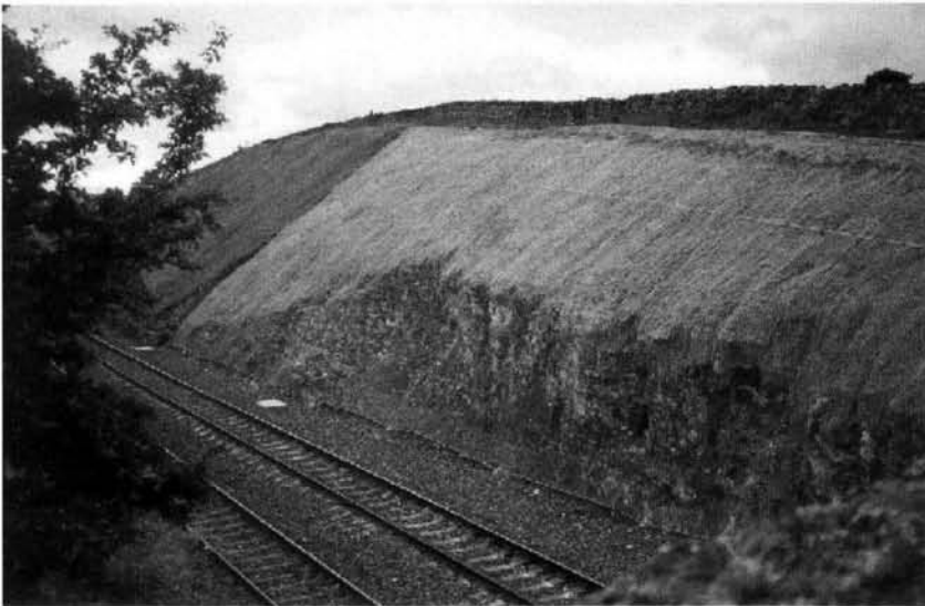
Figure 14, Rock fall failure and repair
