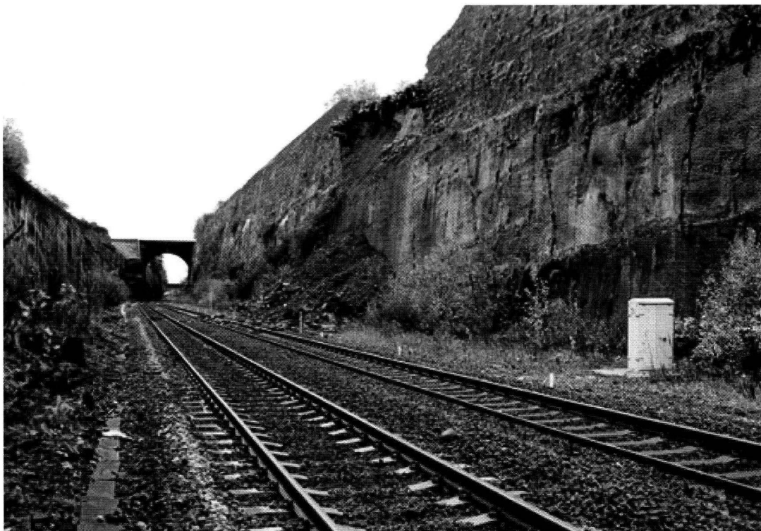
Figure 1, Example of earthwork asset at ultimate limit state
