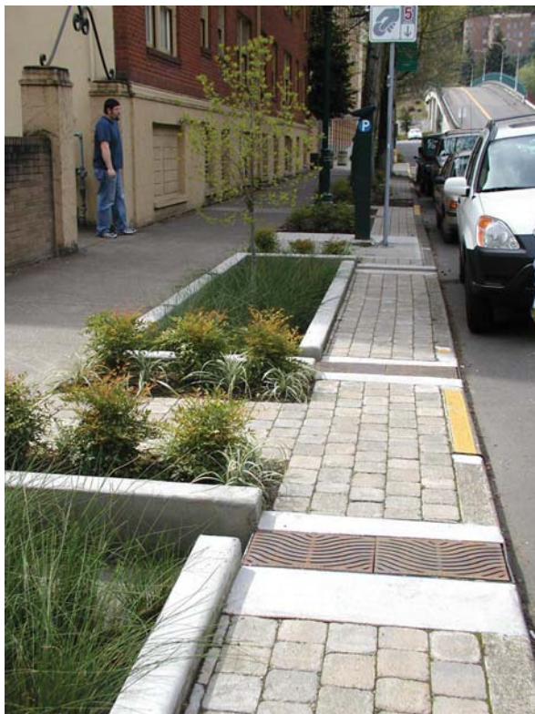
Fig. 8.7 Downtown street design in Portland, Oregon, that filters runoff water from traffic and parking lanes. Grates cover the channels that bring water from the street into the planting areas. Photo by K. Hill
