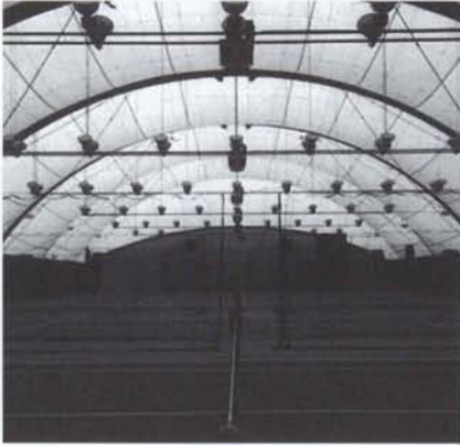
The parallel arches of the Hanover Park, Illinois, tennis facility (ABOVE RIGHT) rely on interior cross-bracing for stability (ABOVE LEFT).
