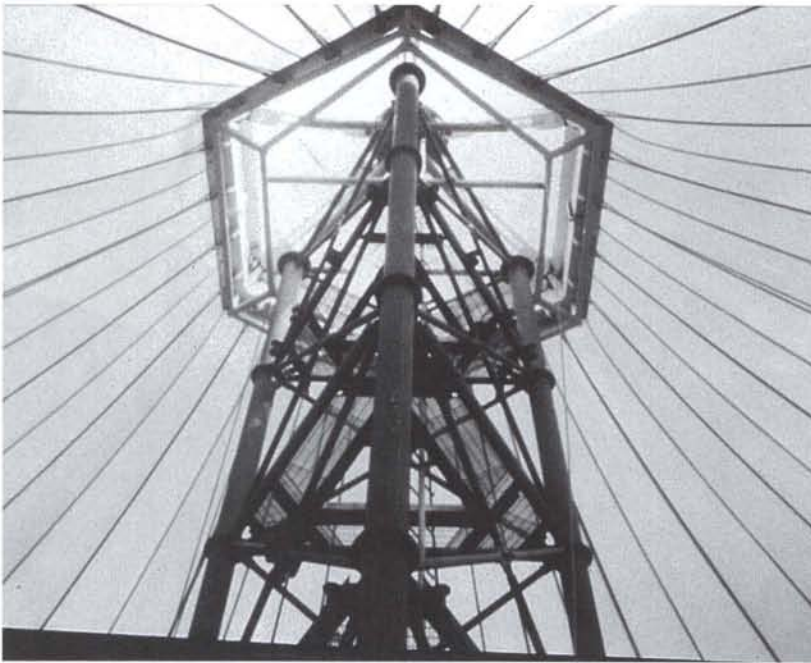
[LEFT] The characteristic upward sweep of seams in the cone roof of the Park City Mall in Lancaster, Pennsylvania, draws the eye up with it.
