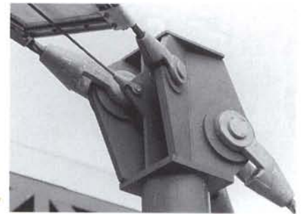
[ABOVE] Connections such as those at Tampa Airport Hanger No. 1 provide workmanlike and visually unambiguous terminations of both cables and fabric.
