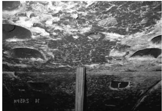
Figure 2. Fire damage to tunnel lining in Shanghai Metro tunnel fire.
