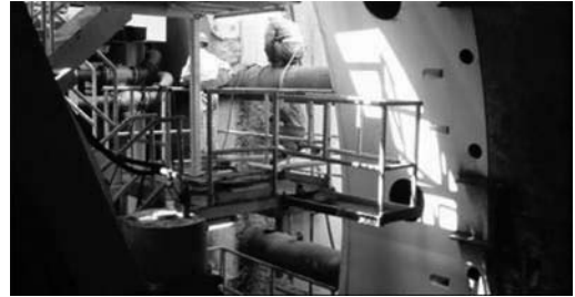
Figure 8. Installing the pipe struts between the concrete reaction structure and the steel thrust frame.
