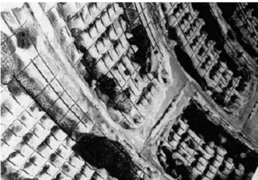
Figure 1. Fire damage to tunnel segments in Channel Tunnel fire (Kirkland 2002).
