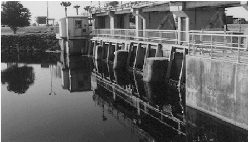
Figure 25. A typical water control gate (USACE 2003).
