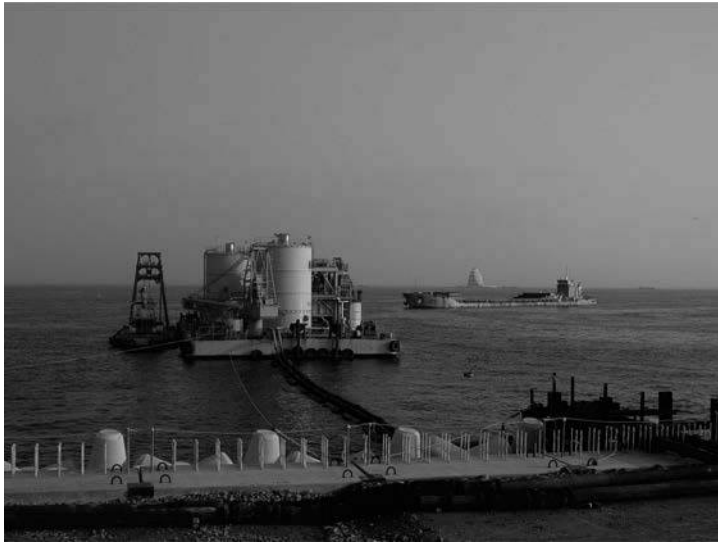
Figure 1.10 Pneumatic flow mixing method at the Tokyo Haneda International Airport construction project.
