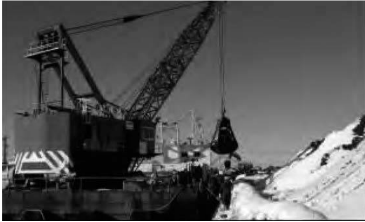
Figure 4.21 Placement of stabilized soil by a shell grab for backfill at Kushiro Port.
