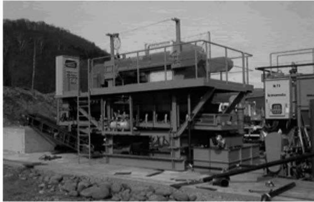
(a) High pressure compressor.
