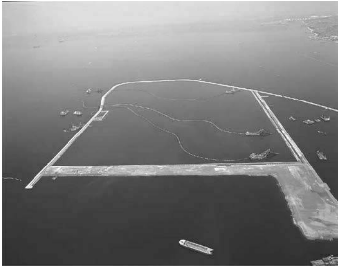
Figure 4.9 Pneumatic execution systems operating at the construction site of Central Japan International Airport.
