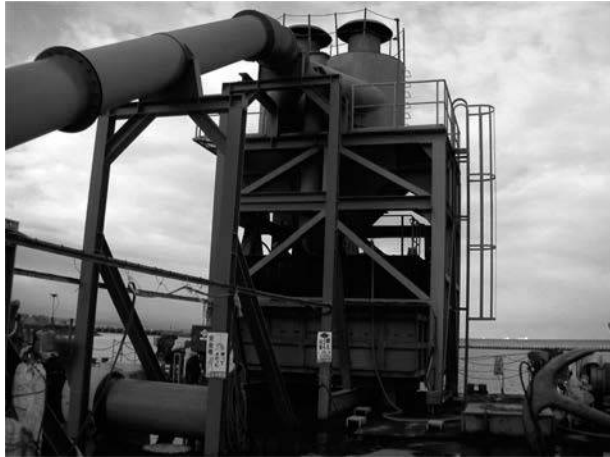
Figure 5.9 Air pressure release cyclone.
