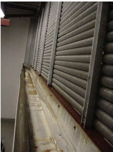
Figure 4.7 – Condensate Pan with Good Drainage
