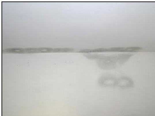
Fig. 3.3 – Water stains on wall and ceiling ( www.epa.gov )
