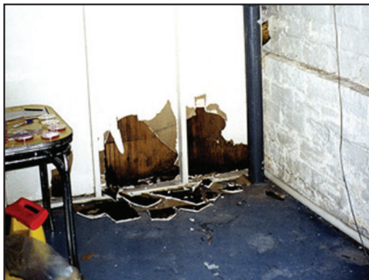
Fig. 3.2 – Front side of wall-board looks fine, but surfaces within the wall cavity are covered with mold ( www.epa.gov )
