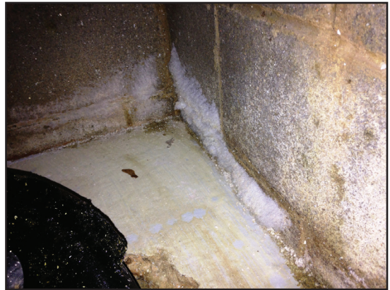
Fig. 3.5 – Efflorescence on Basement Cinder Block Walls
