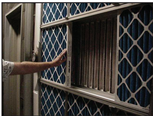
Figure 4.5 – Inspecting Filter Bank (pre-filter is removed here to inspect secondary bag filters)
