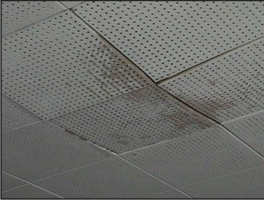
Fig. 3.4 – Acoustic ceiling tiles with water damage (www.epa.gov)
