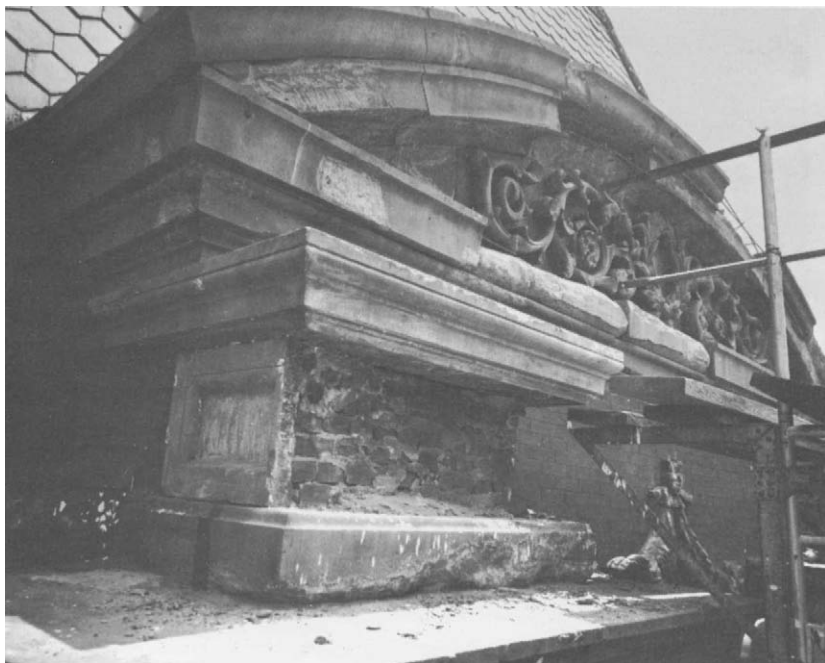
10. Restoration of a pediment of a corner pavilion, The Corcoran Gallery of Art, Washington, D.C.
