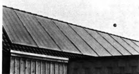
Roof solar collectors
