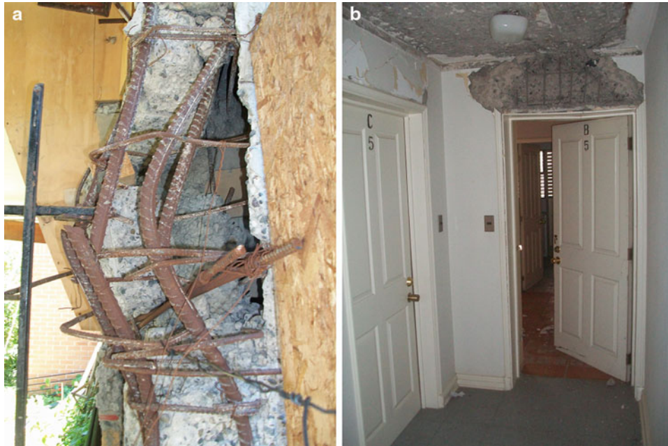
Fig. 39.9 (a) Buckling in longitudinal reinforcement bars first floor columns. (b) Lintel beam cracked
