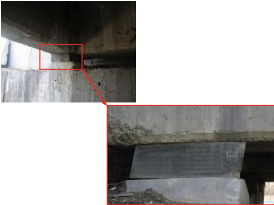
Fig. 18.7 Local damage in isolators
