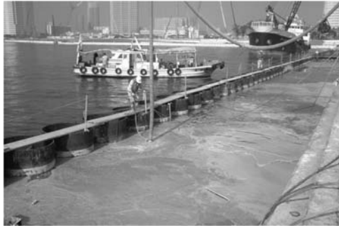
Figure 1.14 Application of Lightweight Geo-material for backfill at Kobe Port (by the courtesy of SGM Lightweight Treated Soil Method Association).
