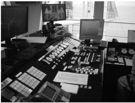
(a) Control desk for operating pumping units.
