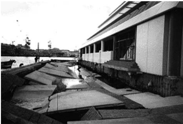
Figure 4.18(c) Damage of sea revetment near the building.
