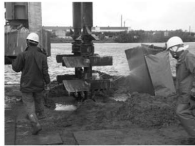
(b) Outlet for low pressure injection.
