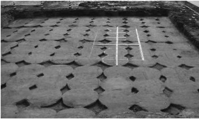
Figure 5.35 Top view of stabilized soil columns by CDM-Lemni 2/3 method (Cement Deep Mixing Method Association, 2005).
