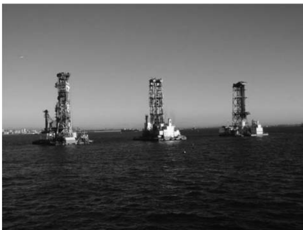
Figure 4.19(d) DMM vessels in operation (by courtesy of the Tokyo/Haneda International Airport Construction Office).
