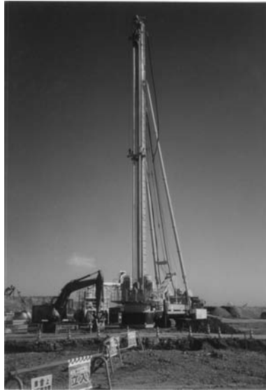
Figure 5.3 DJM machine in operation (by the courtesy of Dry Jet Mixing Association).
