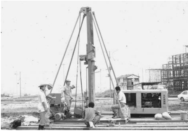
Figure 1.2 First field test with small on-land machine in the 1970s (by the courtesy of Port and Airport Research Institute).
