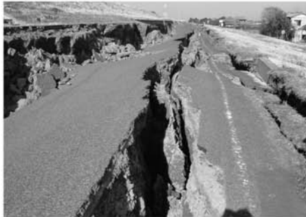
(c) Damage at River embankment without improvement.
