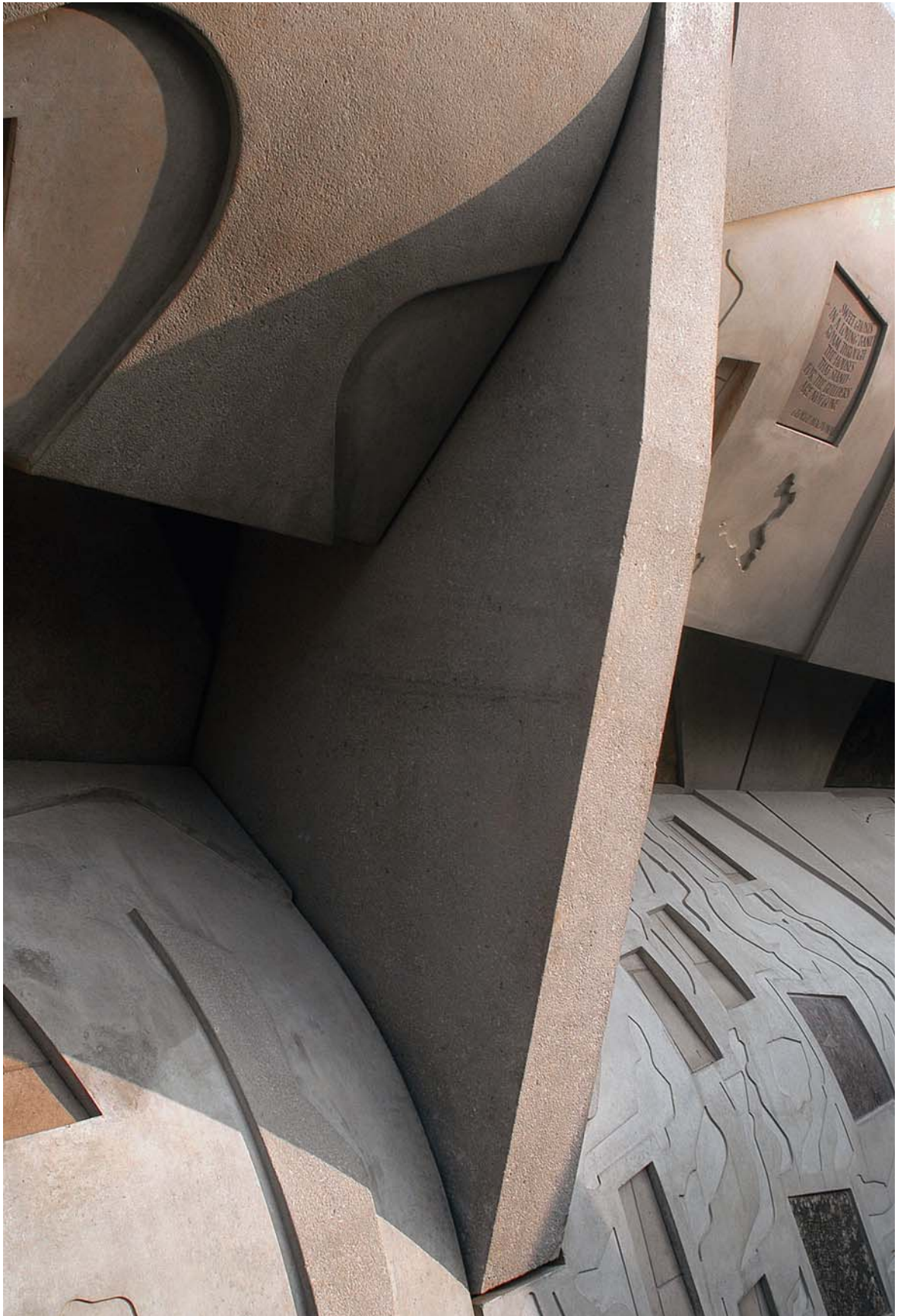
Canongate wall showing separation of upper and lower curvature
