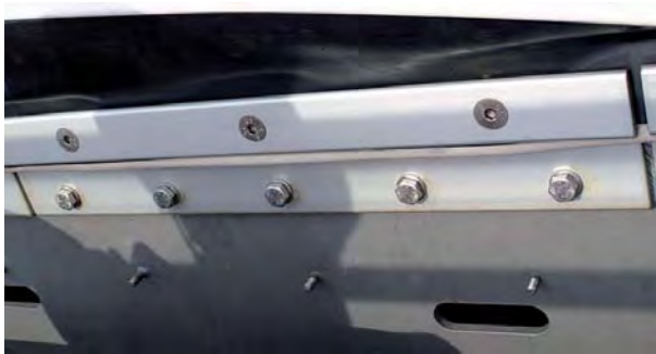
Fig. 139: Clamping plate edge and corner detail for the roofing of the Main Station in Dresden, Germany
