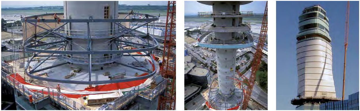
Fig. 229: left, middle: Erection of the first two steel rings; right: Completed membrane surface
