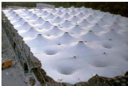
Fig. 247: Erection of the vehicle park roof at the Munich Waste Disposal Office
