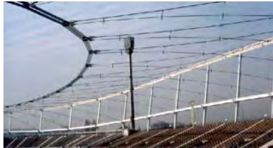
Fig. 239: left: Primary structure with rope trusses; middle: Lifting the rope structure; right: Erection of the compression ring
