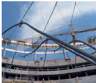
Fig. 301: left: Lifting the spanning ropes at the Waldstadion in Frankfurt/M., Germany; right: Lifting the ropes at the Stadium in Wolfsburg
