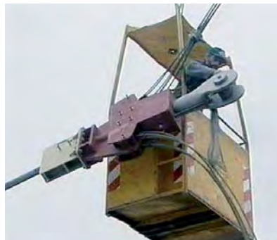
Fig. 300: left: Lifting a rope complete with strand tensioning equipment; right: Lifting a stay rope with rigging rope
