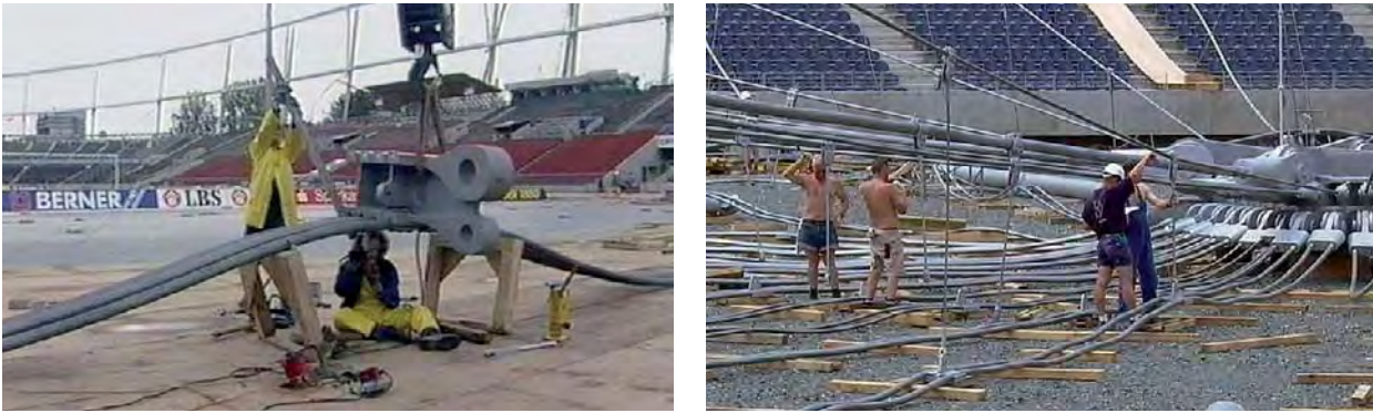
Fig. 292: left : Preassembly of the ring cable at the Gottlieb Daimler stadium; right : Preassembly of the hanger ropes at the Waldstadion, Frankfurt/M., Germany
