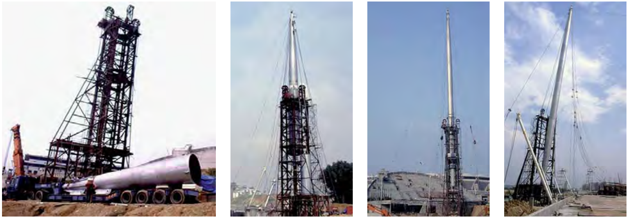
Fig. 225: Segmental erection from underneath for the swimming pool membrane roof in Kuala Lumpur, Malaysia
