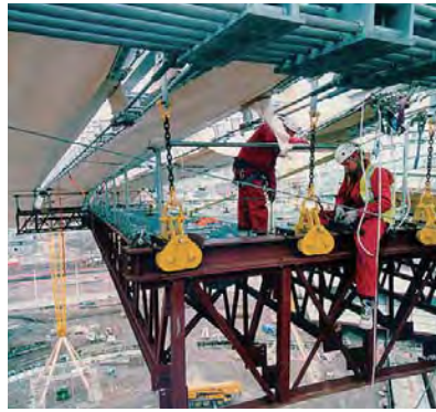
Fig. 197: Hanging scaffolding for the erection of the Millennium Dome in London, England
