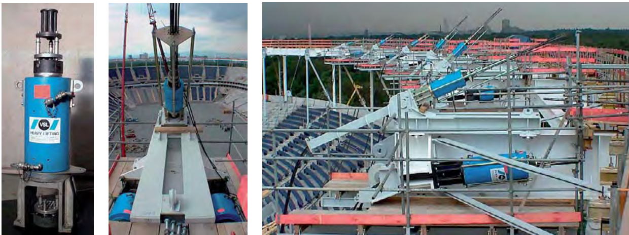
Fig. 176: VSL strand tensoning device and the application for the installation of the cable stays in the construction of the Waldstadion in Frankfurt/M., Germany
