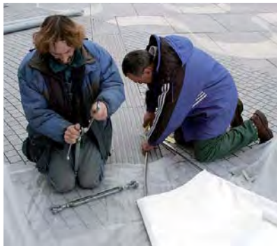
Fig. 297: Mounting the corner fittings and inserting the edge rope of a four-point awning
