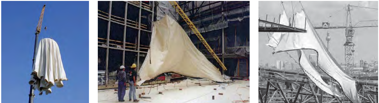
Fig. 309: left: Lifting a high point surface; middle, right: Lifting the segments for the Forum roof at the Sony Center in Berlin, Germany
