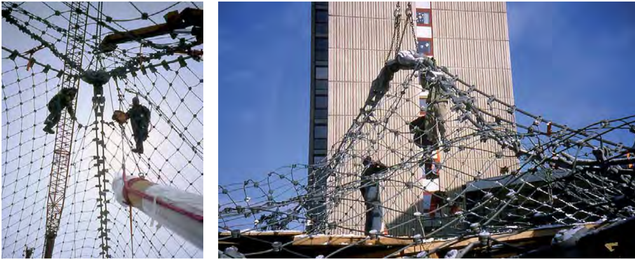
Fig. 303: left: "Threading in" the columns, right: Lifting the rope net for the roofing of the Rhön Clinic in Bad Neustadt, Germany
