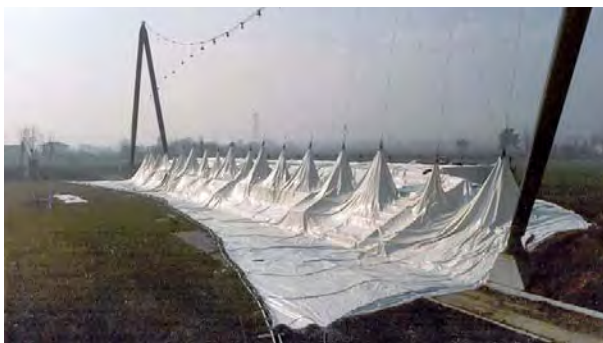
Fig. 257: Erection of a hanging high point surface by pulling up the hanger rope system
