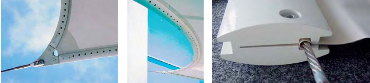
Fig. 141: left: Corner connection and edge detail to the roof over the entrance to the Federal Chancellor's Office in Berlin, Germany; right: Detail photo of clamping profile
