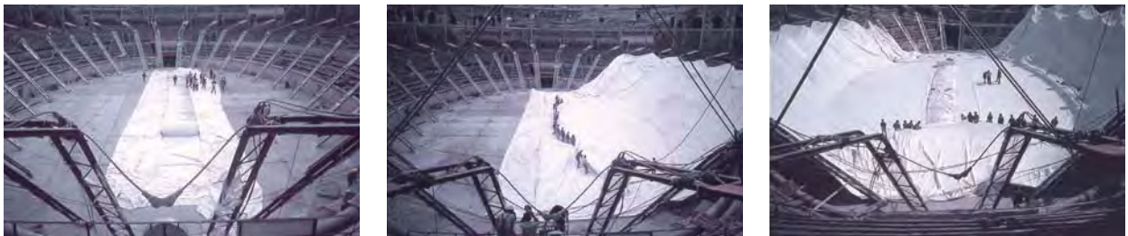
Fig. 155: Laying out the lower and upper membranes for the roofing of the Arena in Nimes, France
