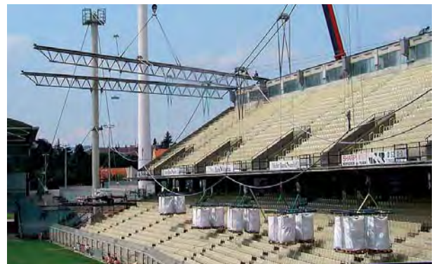
Fig. 203: top: Ballasting a wire rope construction for glass panels with sandbags at the nodes; bottom: Ballasting two carrier ropes with water containers during the erection of the roof over the Gerhard Hanappi Stadion in Vienna, Austria
