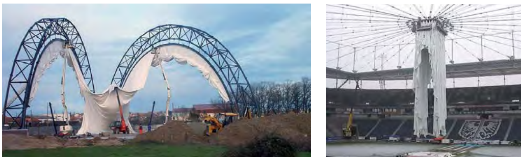
Fig. 311: left: Lifting a membrane premounted to arches; right: Lifting a transformable membrane surface
