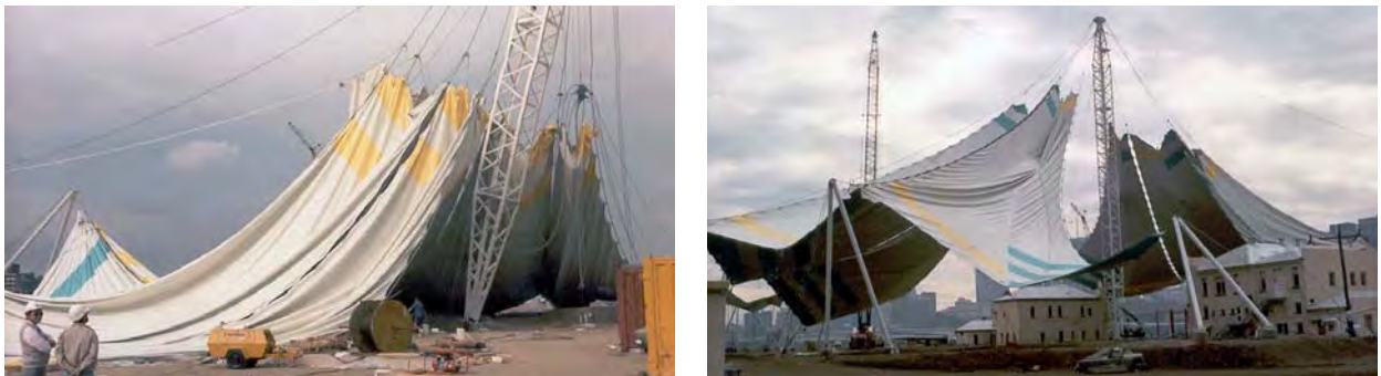
Fig. 310: Pulling in the 11,000 m 2 partial area for the membrane roof over the EXPO grounds in Brisbane, Australia
