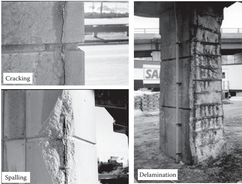
Figure 9.2 (See color insert.) Cracking, spalling, and delamination of concrete cover due to corrosion of embedded reinforcement.
