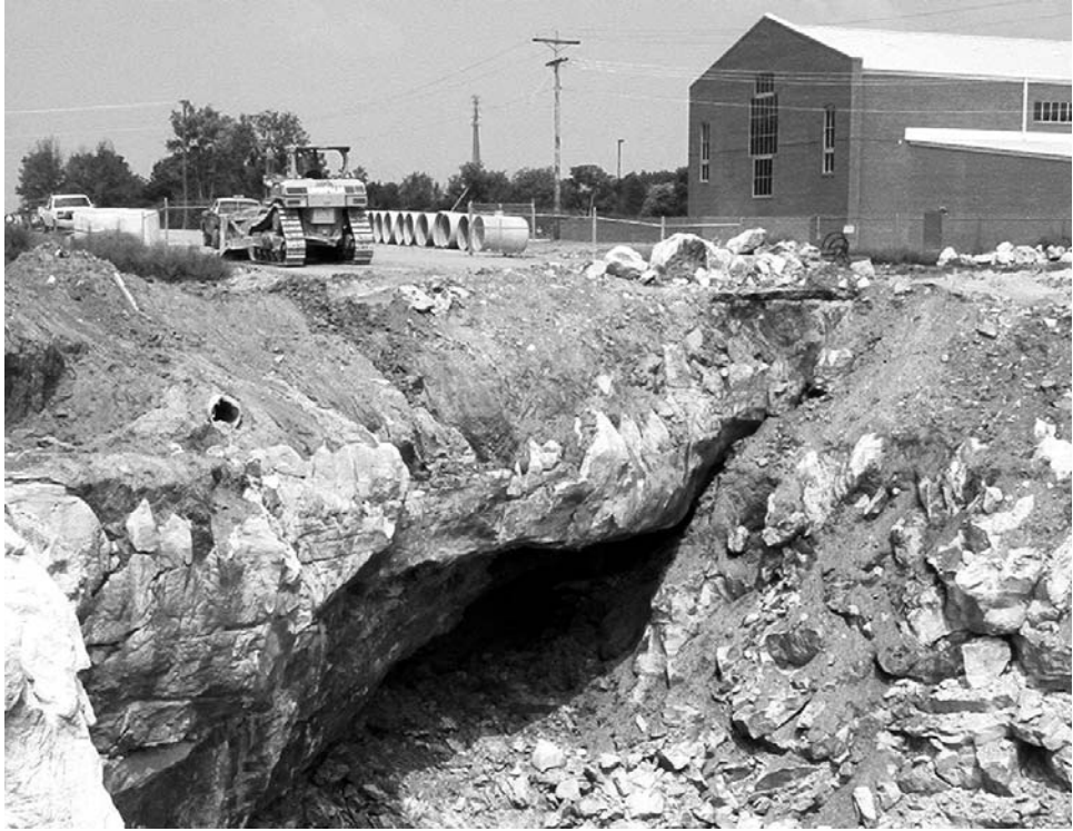
Figure 7.1. Fractured rock around the margin of the new collapse sinkhole that destroyed Dishman Lane in Bowling Green, Kentucky, in 2002.
