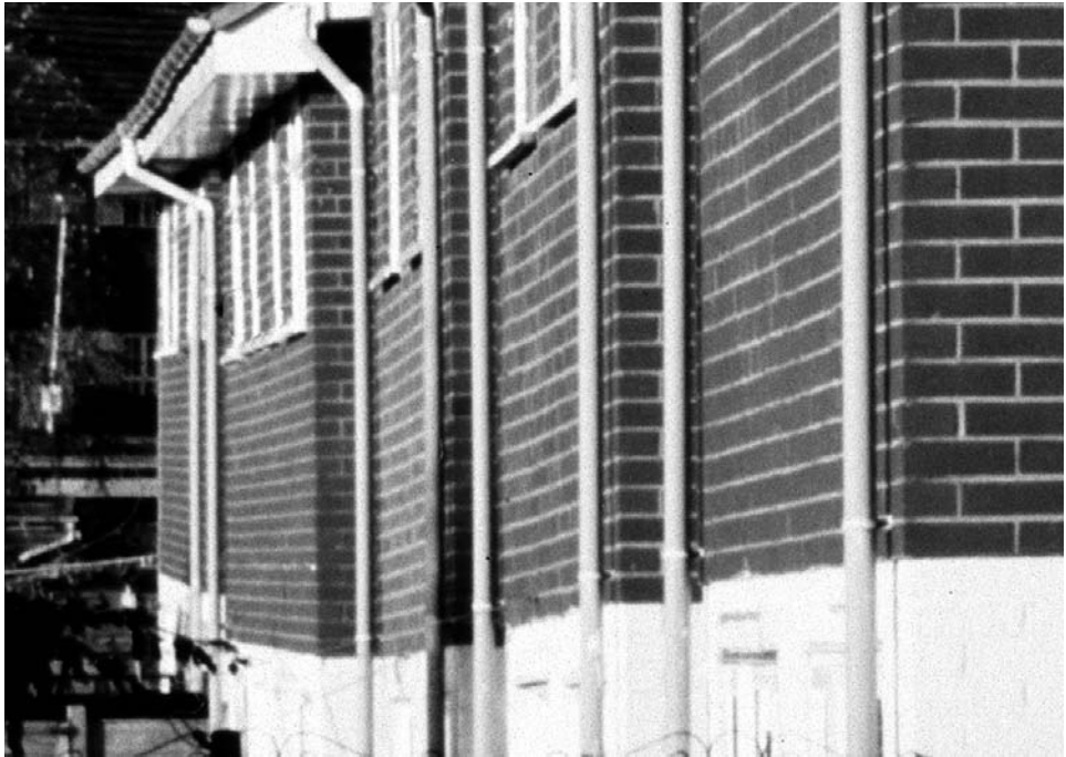
Figure 2.8. Houses in Sandbach subsided and tilted due to dissolution and removal of salt from the rockhead zone beneath 20 m of drift cover, in the Cheshire Plain, U.K. TW.
