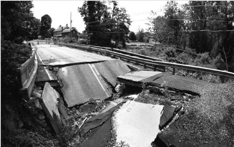
Figure 8.2.2. The bridge that carried Tatamy Road over Bushkill Creek, destroyed by an expanding and ever-changing cluster of sinkholes. TW.
