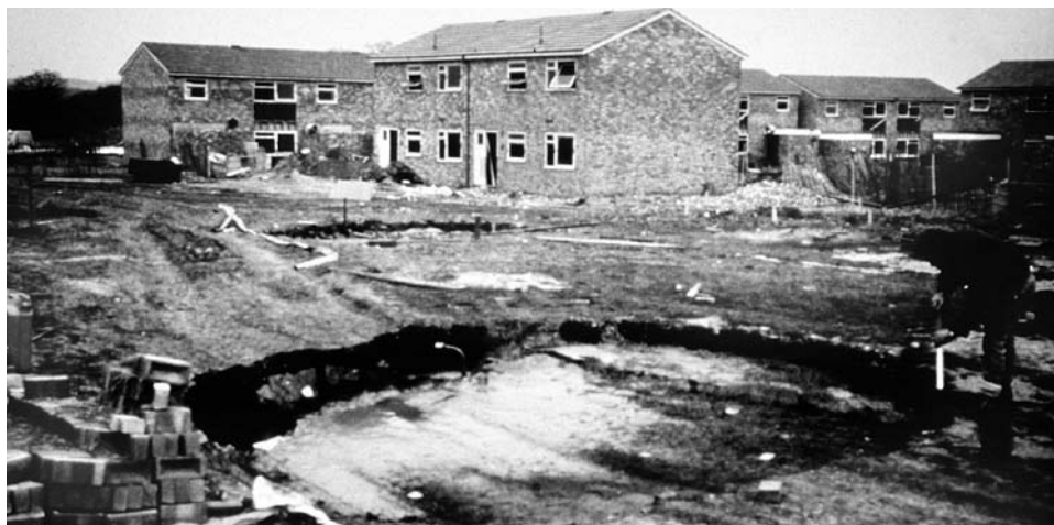
Figure 5.15. Subsidence of about 300 mm over a chalk pipe whose fill was disturbed by construction activity on a site in the English Chiltern Hills.
