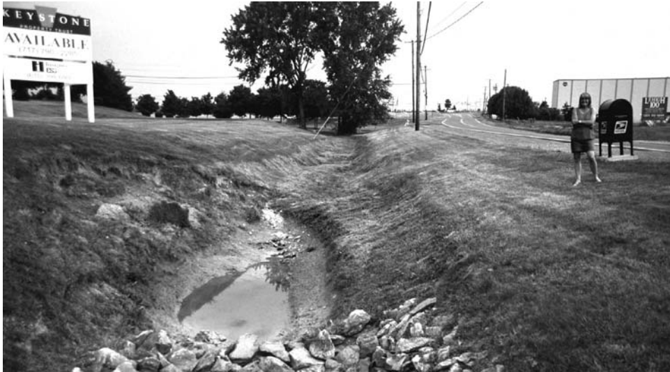
Figure 8.1. Early stages of a sinkhole developing in the untreated soil floor of a ditch beside a Pennsylvanian highway; it is temporarily choked with clay, while the riprap in the foreground was placed to prevent erosion at a culvert outlet.
