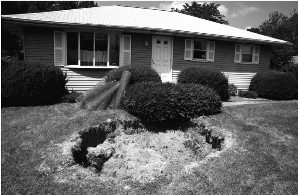
Figure 4.8. A dropout sinkhole in the front lawn of a house in Pennsylvania; the hole was originally 5 m deep but was filled with soil to prevent the sides flaring out, and the soil fill had compacted and settled by 0.7 m by the time this photo was taken. TW.
