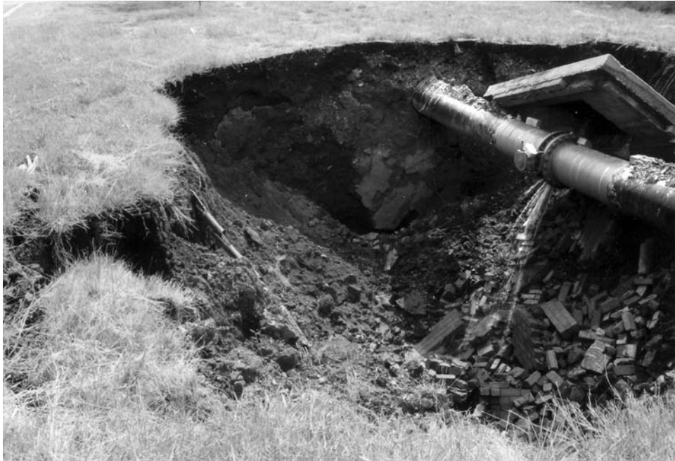
Figure 1.12. A small suffosion sinkhole that has opened up beneath a leaking pipeline in the soil-covered dolomite karst south of Pretoria, South Africa.
