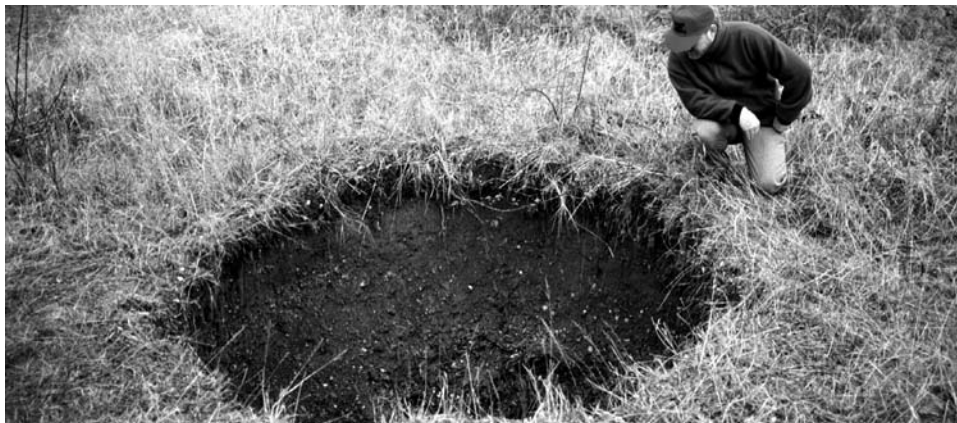
Figure 8.2. One of the cluster of subsidence sinkholes induced by a broken water main on the English chalk downs; there was no surface flow, but the dropouts developed above suffosion points in the soil over bedrock fissures.
