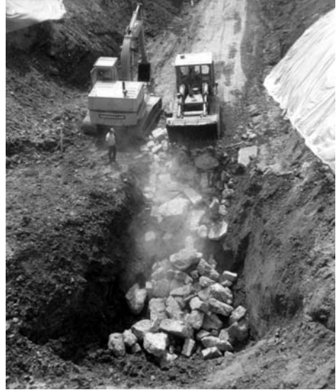
Figure 11.8. Chunk rock being placed at the lowest exposed point in the Macungie sinkhole. Photo: Percy Dougherty.
