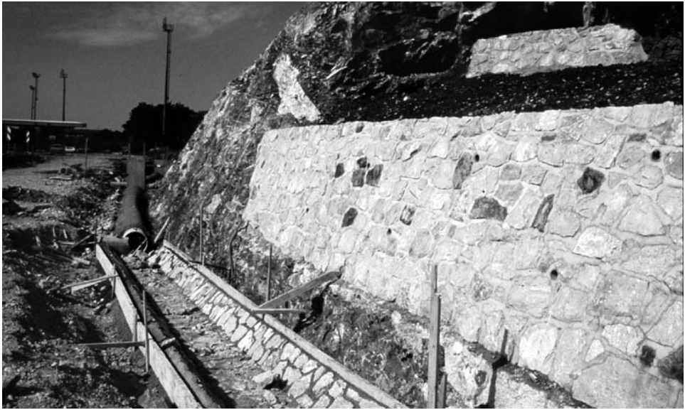
Figure 13.3.5. Construction of an impermeable roadbed through a cutting where a breached cave has been walled off, along a motorway to Italy.
