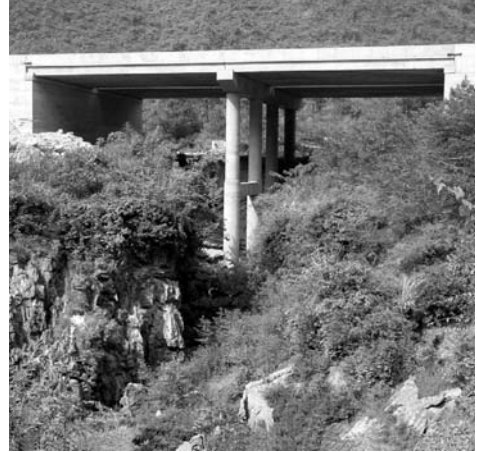
Figure 13.5.7. Piers stand on piles founded on sound bedrock to carry the Shui-Nan Highway over a section of difficult karst ground. Photo: Mingtang Lei.
