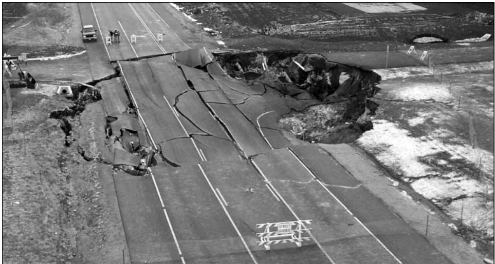
Figure 13.2.1. Aerial view of the collapse sinkhole in Dishman Lane, Bowling Green, seen looking towards the south-east
