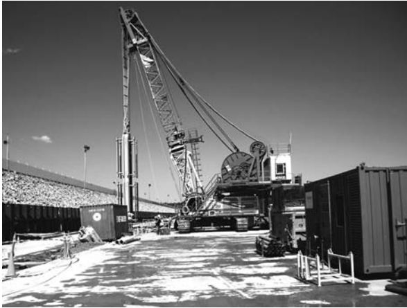
Photo 4.7 Hydromill operation at Wolf Creek Dam, Kentucky. (Courtesy of TREVIICOS Soletanche JV USACE.)
