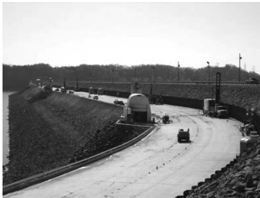
Photo 2.9 Multiple drilling and grouting operations at Wolf Creek Dam, Kentucky. (Courtesy of Advanced Construction Techniques, Ltd.)
