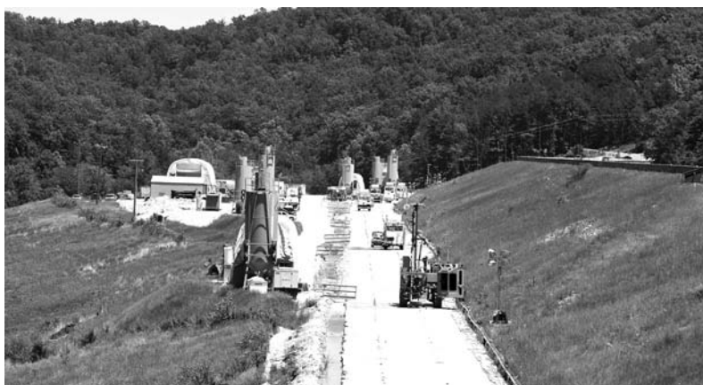
Photo 2.5 Drilling and grouting operations at Clearwater Dam. (Courtesy of Advanced Construction Techniques, Ltd.)
