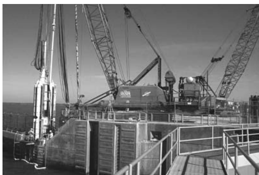
Photo 4.21 Hydromill cutting the lock walls standing on the concrete dam, W. F. George Dam, Alabama. (M. Siepi, personal communication, 2011.)
