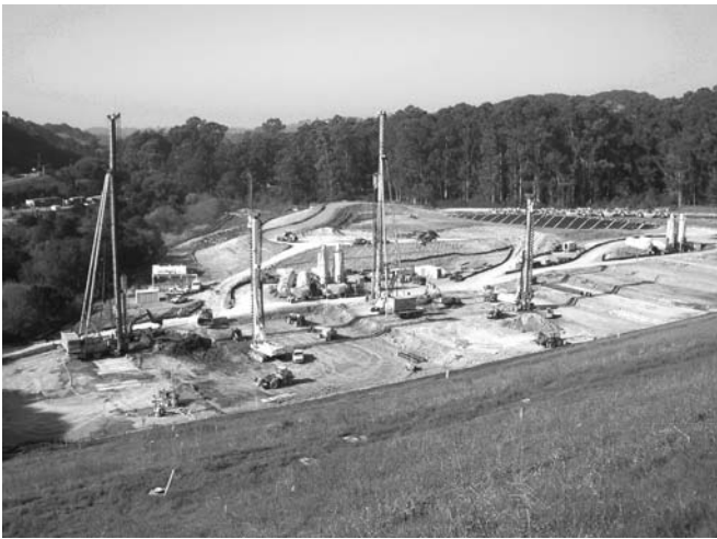
Photo 3.9 Predrilling and DMM treatment at San Pablo Dam, California. (Courtesy of Yujin Nishimura, Raito, Inc.)
