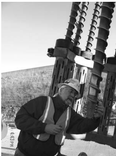
Photo 2.1 Inner auger used to clean out drilled casing. (Courtesy of Advanced Construction Techniques, Ltd.)
