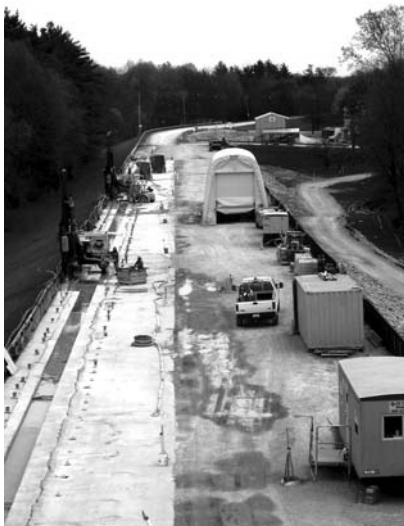
Photo 5.1 View of the remediation works at Mississinewa Dam, Indiana. (Courtesy of ACT, Gannett Fleming, and the USACE.)
