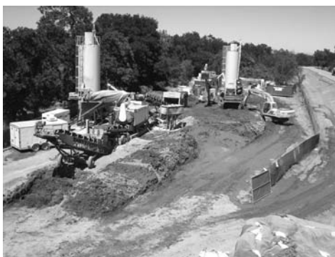
Photo 4.2 Pugmill mixing plant, Mayhew Levee, Sacramento, California.
