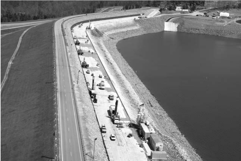
Photo 2.6 Wolf Creek Dam, Kentucky, embankment foundation grouting project. (Courtesy of Advanced Construction Techniques, Ltd.)
