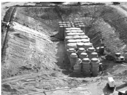
Photo 2.14 Aerial view of the test area from the west, Tuttle Creek Dam, Kansas. (From Mauro, M., and F. Santillan, “Large Scale Jet Grouting and Deep Mixing Test Program at Tuttle Creek Dam.” Proceedings of the 33rd Annual and 11th International Conference on Deep Foundations , 2008. With permission.)
