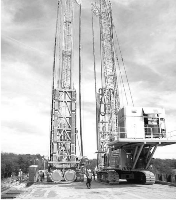
Photo 4.6 Hydromill being moved along the work platform at Mississinewa Dam, Indiana. (Courtesy of Bencor-Petrifond JV and USACE.)
