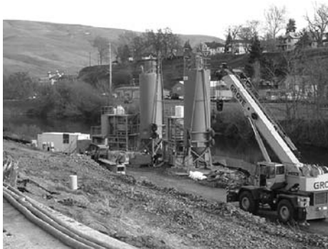
Photo 3.5 Batch plant on the seepage berm at the landside toe of Lewiston Levee, Idaho. (After Gibbons, Y. R., and G. J. Buechel, "Lewiston Levees DSM Wall Construction," 18th Annual Conference of the Association of State Dam Safety Officials, www.damsafety.org , Snowbird, Utah, 2001; Courtesy of Association of State Dam Safety Officials.)
