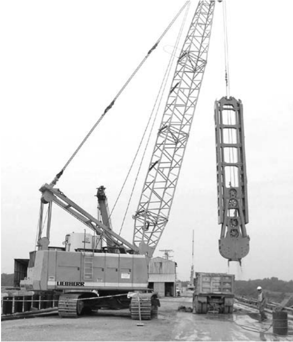
Photo 4.11 Heavy-duty cable-suspended and operated clamshell, Mississinewa Dam, Indiana. (Courtesy of Bencor-Petrifond JV and USACE.)
