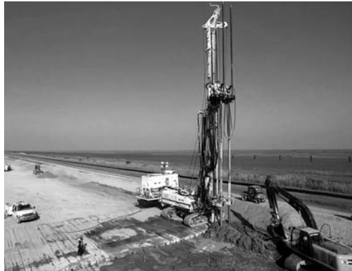
Photo 3.1 Twin Axis DMM machine (WJE system) installing soilcrete panels on a levee in New Orleans, Louisiana. (Courtesy of TREVIICOS Corp.)
