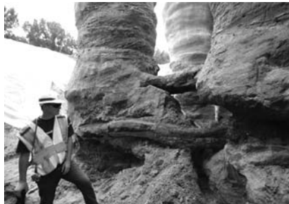
Photo 2.15 Effect of an obstruction in a double-fluid jet grout column, Tuttle Creek Dam, Kansas. (From Mauro, M., and F. Santillan, “Large Scale Jet Grouting and Deep Mixing Test Program at Tuttle Creek Dam.” Proceedings of the 33rd Annual and 11th International Conference on Deep Foundations , 2008. With permission.)
