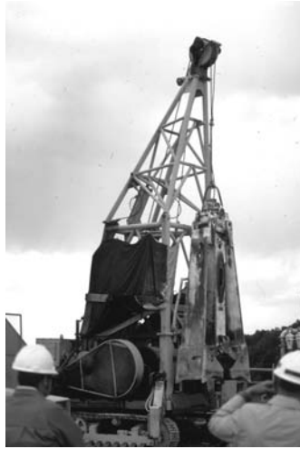
Photo 4.10 Cable-suspended grab in operation off a specially developed tracked rig, Wolf Creek Dam, 1975–79. (Courtesy of Arturo Ressi.)
