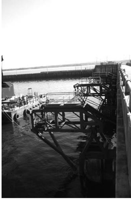
Photo 4.19 Template supports out from the buttresses of the dam, W. F. George Dam, Alabama. (M. Siepi, personal communication, 2011.)
