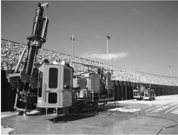
Photo 2.8 Drilling with down-the-hole rotary percussion water hammer, Wolf Creek Dam, Kentucky. (Courtesy of Advanced Construction Techniques, Ltd.)
