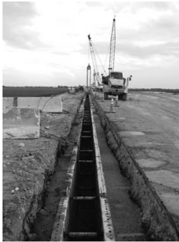
Photo 4.8 Guide wall installed prior to excavating a remedial cutoff wall. (Courtesy of Bencor.)
