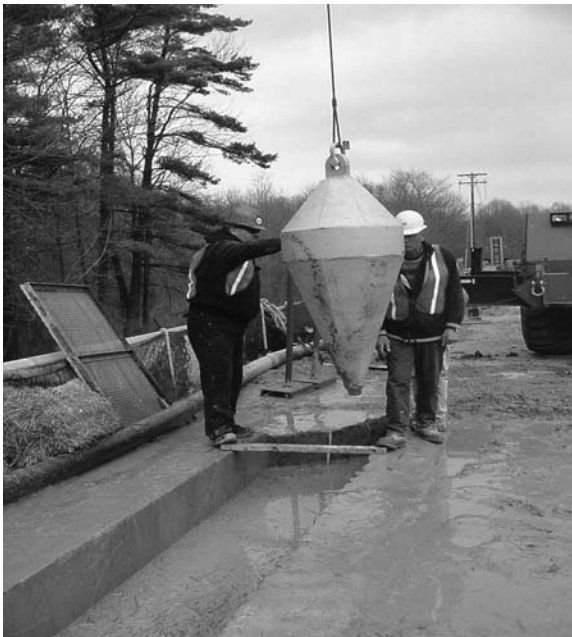
Photo 4.12 Traditional plumb-bob method as used in concert with modern methods to check panel deviation. (Courtesy of Bencor-Petrifond JV and USACE.)
