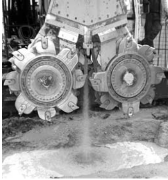
Photo 3.14 Slurry injected between the cutting and mixing wheels of the CSM head.
