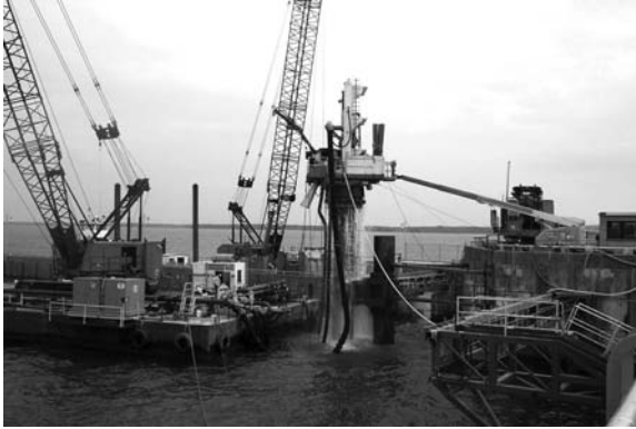
Photo 4.20 Top pile rig excavating with reverse-circulation method, W. F. George Dam, Alabama. (M. Siepi, personal communication, 2011.)
