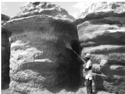
Photo 2.13 Exposed triple-fluid columns, Tuttle Creek Dam, Kansas. (From Mauro, M., and F. Santillan, “Large Scale Jet Grouting and Deep Mixing Test Program at Tuttle Creek Dam.” Proceedings of the 33rd Annual and 11th International Conference on Deep Foundations , 2008. With permission.)
