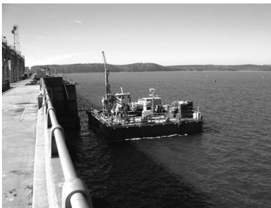
Photo 4.18 The exploratory and grouting campaign being conducted from a barge, W. F. George Dam, Alabama. (M. Siepi, personal communication, 2011.)
