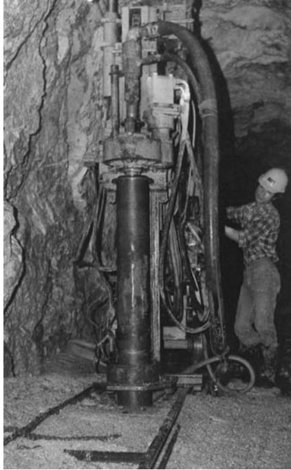
Photo 4.15 Drilling with 300-mm DTH hammer in the galleries, Khao Laem Dam, Thailand. (From Rodio, Khao Laem Multipurpose Project—C3—Concrete Diaphragm Wall—Construction Method Analysis, Internal Report, 1980. With permission.)
