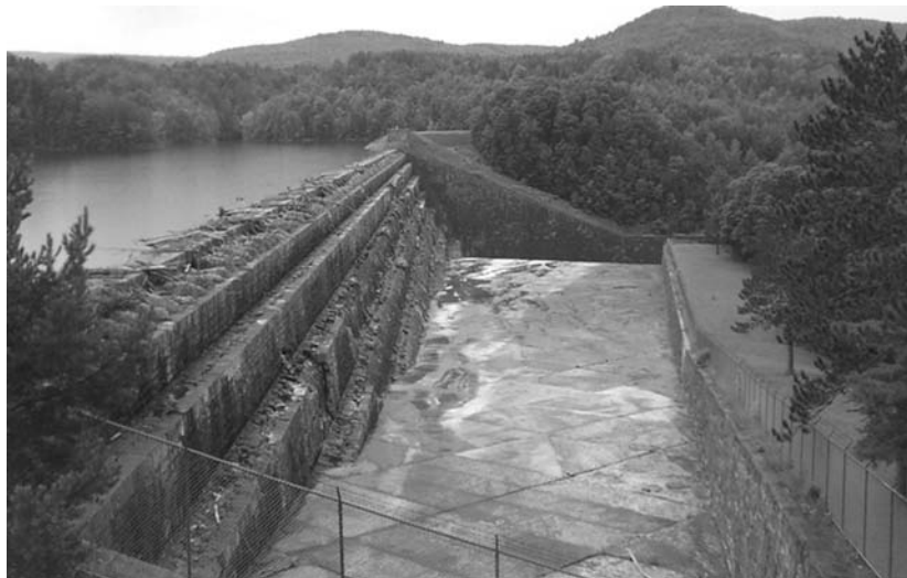
Photo 6.3 Gilboa Dam, New York, in summer 2003. (Modified from Zicko, K. E., D. A. Bruce, and R. A. Kline, Jr., “The Stabilization of Gilboa Dam, New York, Using High Capacity Rock Anchors: Addressing Service Performance Issues,” Paper presented at Institution of Civil Engineers, Ground Anchorages and Anchored Structures in Service, London, England, 2007.)
