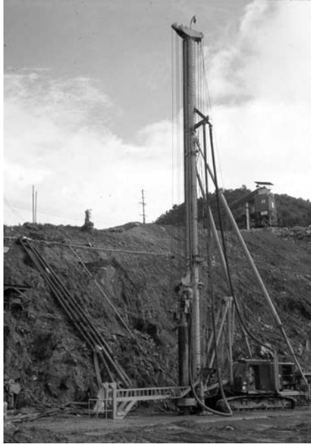
Photo 4.14 The secant pile rig showing the rod-loading system, Khao Laem Dam, Thailand. (From Rodio, Khao Laem Multipurpose Project—C3—Concrete Diaphragm Wall—Construction Method Analysis, Internal Report, 1980. With permission.)
