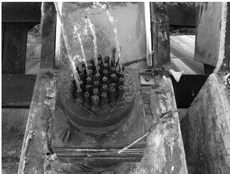
Photo 6.4 Typical corroded anchor head in 2008 at John Day Dam, Washington. (Note water spraying out of strands.) (From Heslin, G., D. A. Bruce, G. S. Littlejohn, and T. Westover, "Performance of Aging Post-Tensioned Rock Anchors in Dams," ASDSO Northeast Regional Conference, State College, PA, 2009. With permission.)
