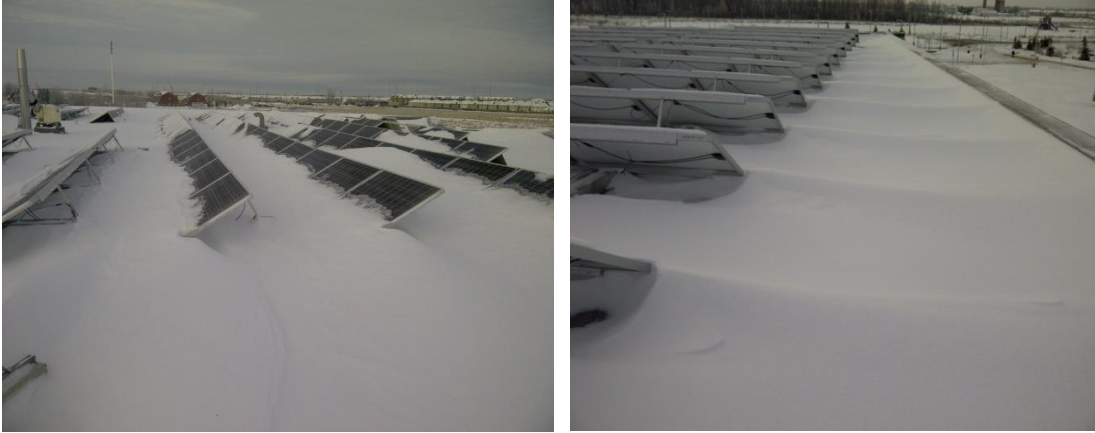
Fig. 1-3. Typical Tilted–Open Solar Panels (Photos courtesy of SLK Solar Corporation)
