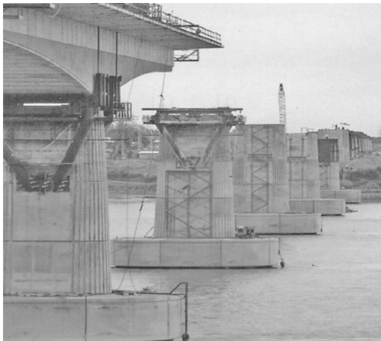
Figure 11.6 The Mekong River Bridge during construction, with pier 12 ready for the installation of two banks of three 450 kN capacity STUs
