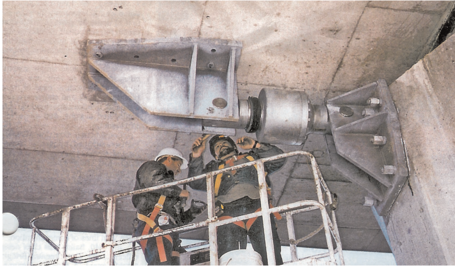
Figure 5.10 An STU being installed at the expansion joint of a pier on the Arthur Laing Bridge ( Bridge Design and Engineering , February 1997, p. 51). © D.S. TechStar, Inc.
