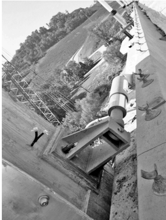
Figure 7.11 One of the eight 1300 kN STUs installed at the two towers of the Maysville Bridge
