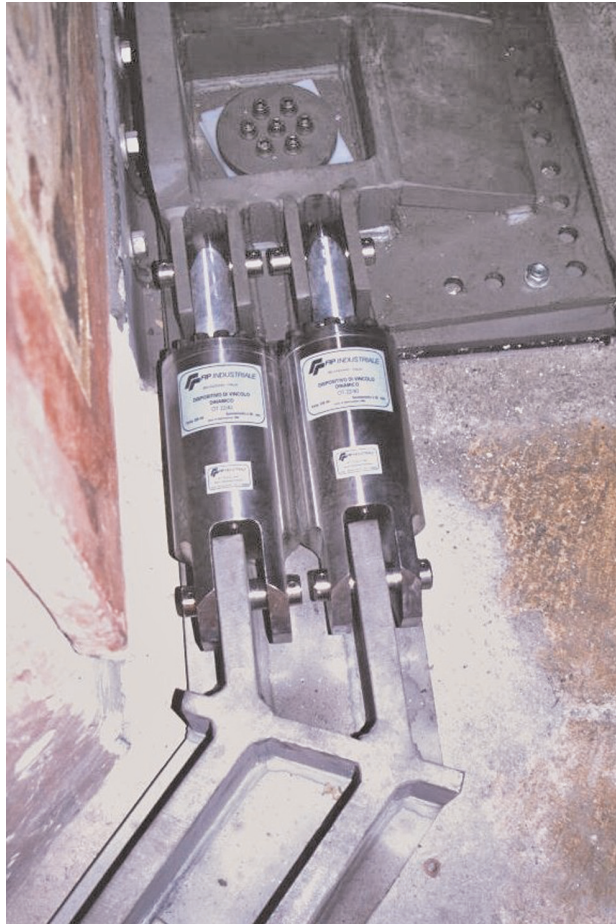
Figure 8.14 Two STUs connecting the steel girders in the upper basilica of San Francesco. Reproduced courtesy of FIP Industriale SpA
