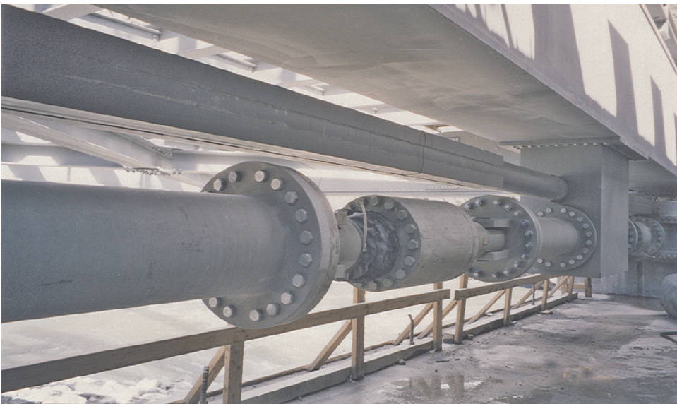
Figure 4.8 Two STUs per abutment installed transversely at the abutment of the Goff Bridge
