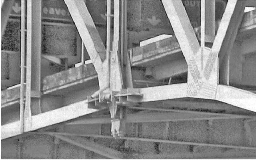
Figure 17.17 An STU at panel L13 of the Marquam Bridge. Image courtesy of the Oregon Department of Transportation
