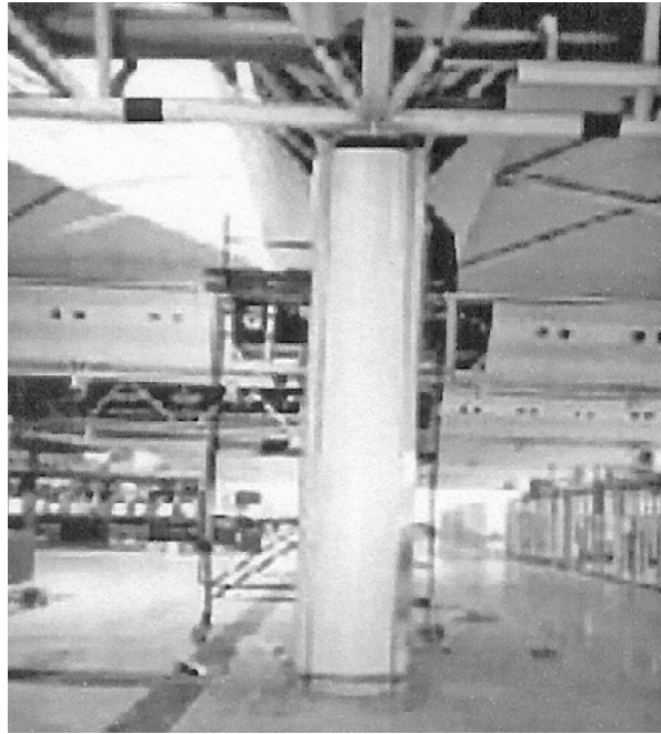
Figure 8.10 A typical third-storey column carrying the roof trusses over a friction pendulum bearing. © Michael Constantinou, Andrew S. Whittaker and Emmanuel Velivasakis, University at Buffalo
