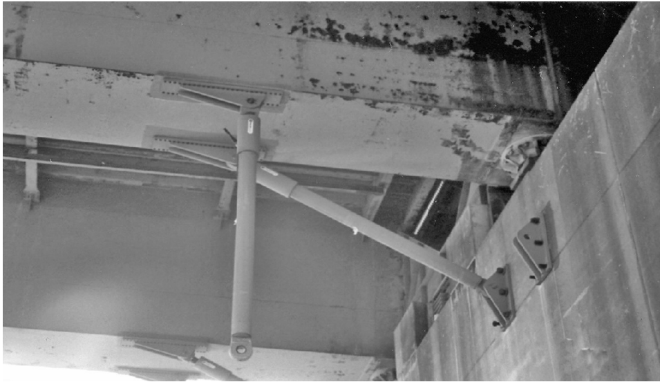
Figure 5.7 The STUs installed on the Poplar Street Bridge
