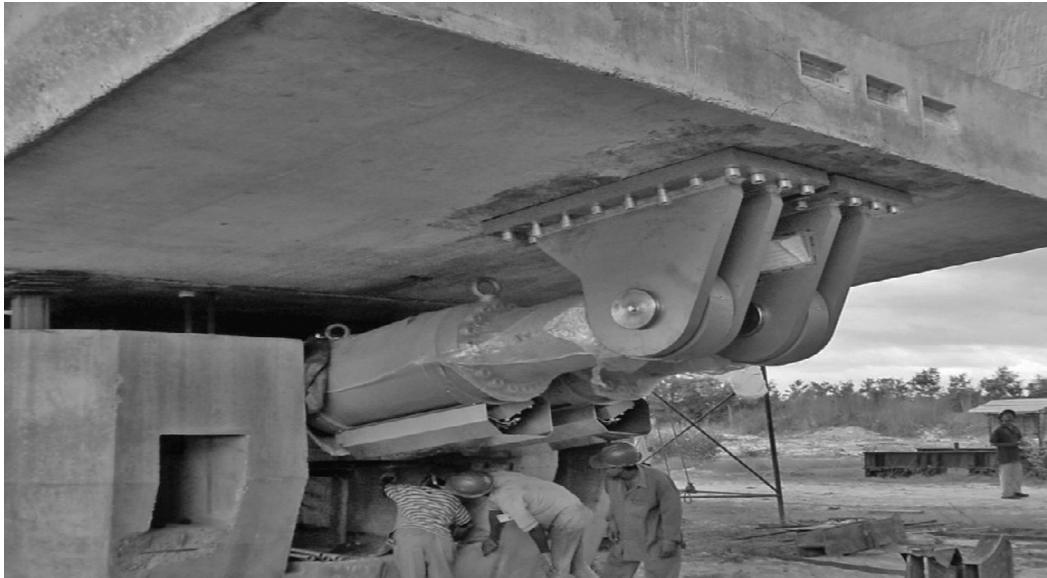
Figure 4.6 STUs being installed on one of the piers of the Paksey Bridge (Hongbing et al. , 2004). © D.S. TechStar, Inc.
