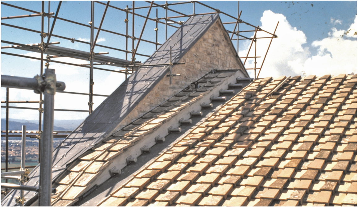
Figure 8.16 Shape-memory alloy devices connecting the roof of the upper basilica of San Francesco. Reproduced courtesy of FIP Industriale SpA
