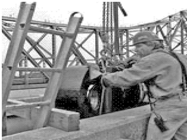
Figure 11.10 The STU is lowered down into the recess in the bottom chord to be attached to the fabricated brackets
