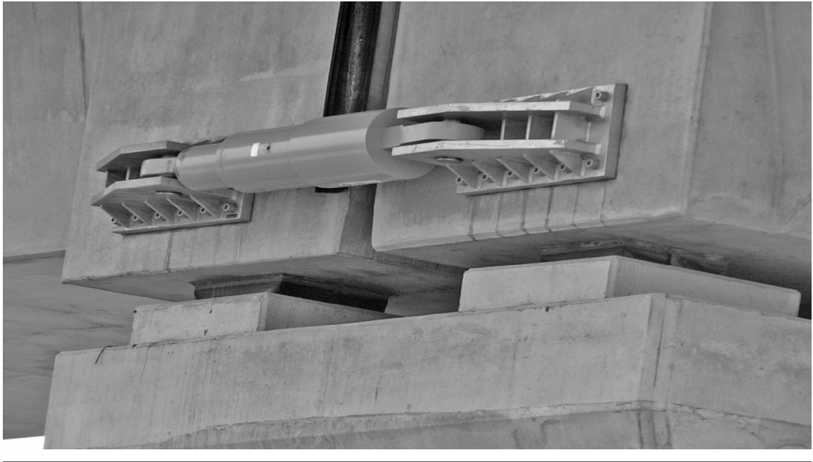
Figure 6.3 A typical 3900 kN STU installed at the expansion joint of the simply supported viaduct
