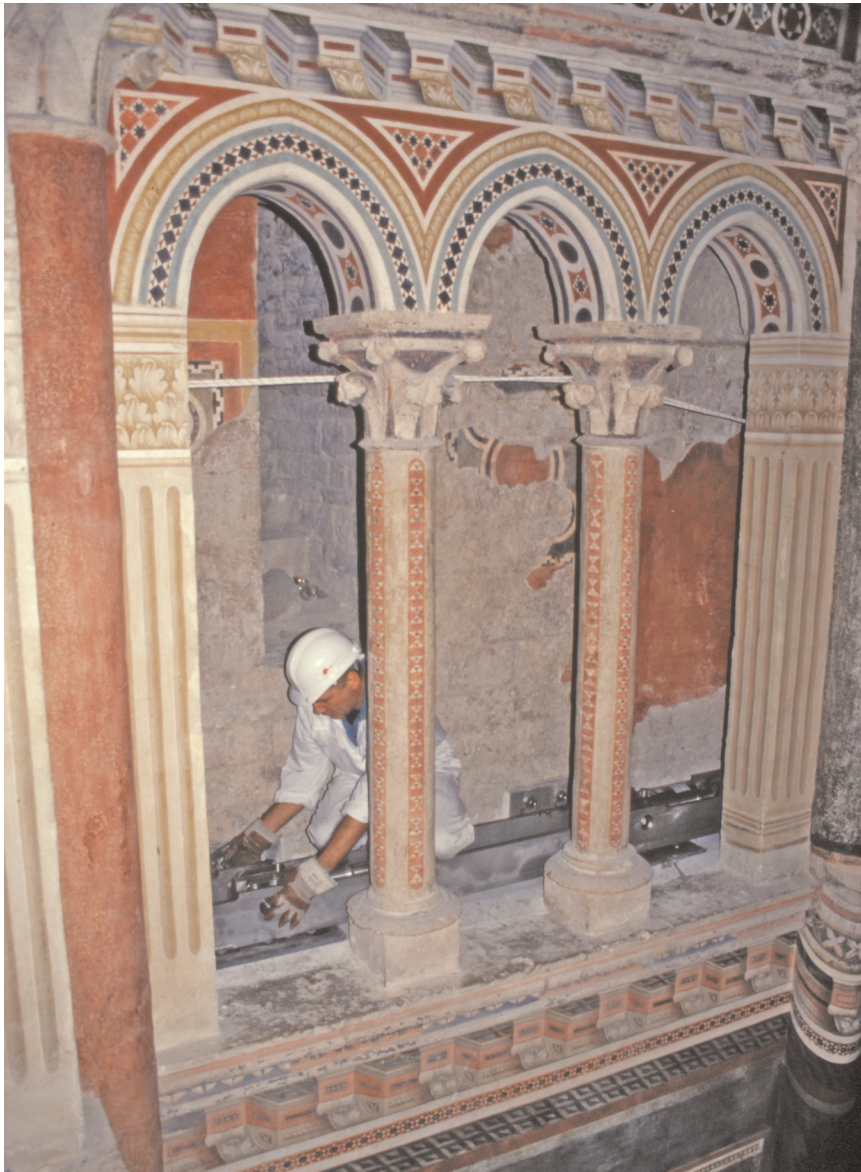
Figure 8.12 The damaged Giotto frescoes in the upper basilica of San Francesco
