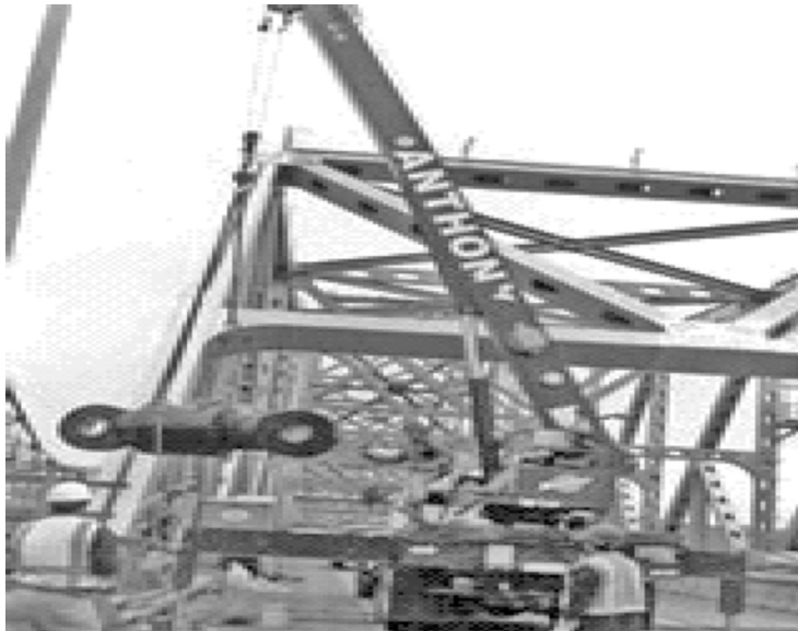
Figure 11.9 The STU is lifted using eye bolts threaded into tapped holes in the end caps of each cylinder
