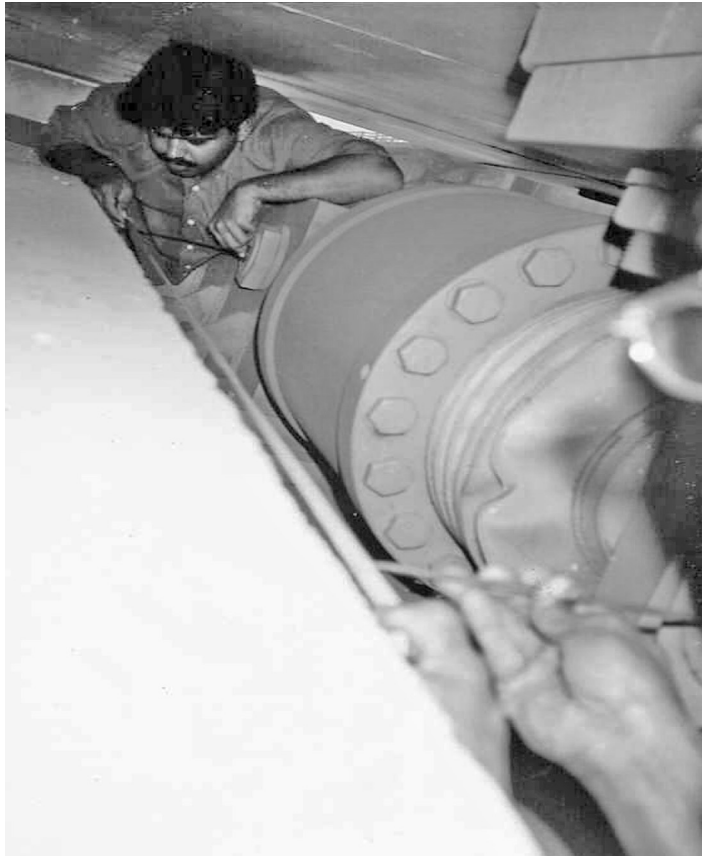
Figure 14.1 Measuring the pin-to-pin distance of an STU on the Second Bassein Creek Bridge
