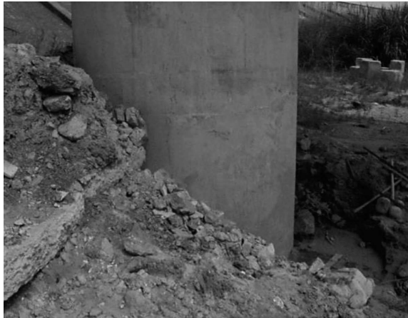
Figure 12.6 Lateral spreading past a bridge pier at the new Taichung bridge, Taiwan.
