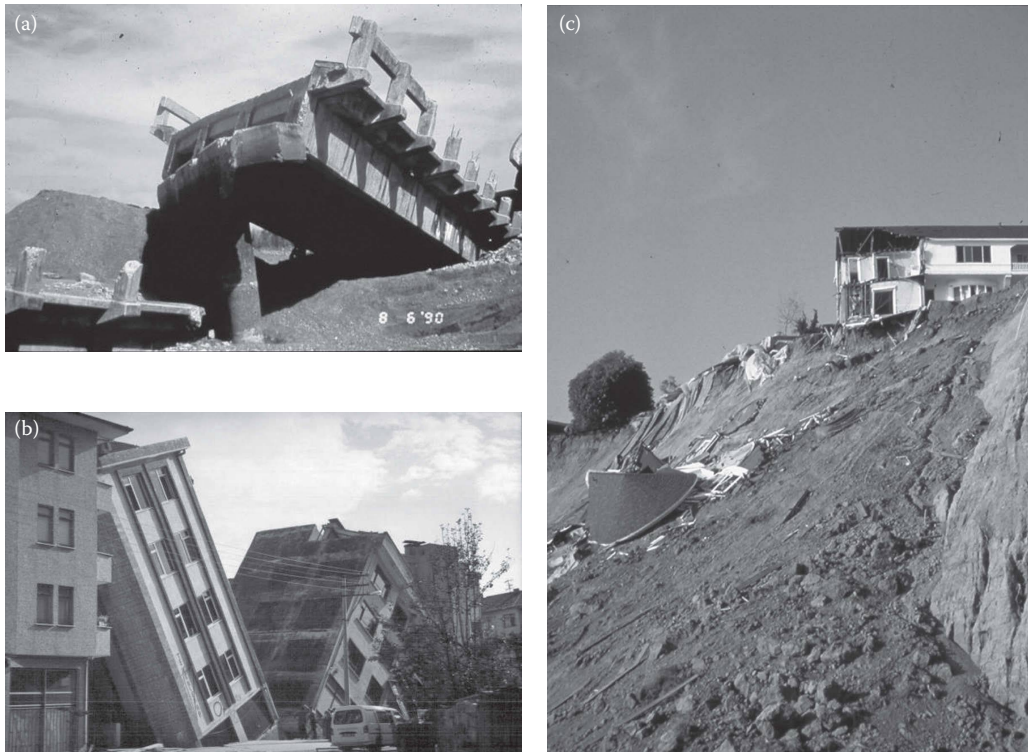
Figure 11.2 Examples of poorly sited structures. (a) Fault Rupture – Luzon, Philippines 1990. (b) Liquefaction – Adapazari, Turkey 1999. (c) Slope Instability – Pacific Palisades, Los Angeles, 1994.
