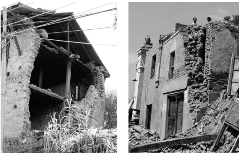
Figure 9.1 Examples of collapse due to poor connectivity of perpendicular walls and lack of horizontal ties at floor levels to ensure box behaviour.
