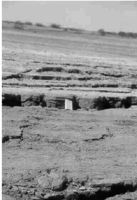
Figure 12.9 Lateral spreading of the downstream slope of an earth dam in Gujarat, India.
