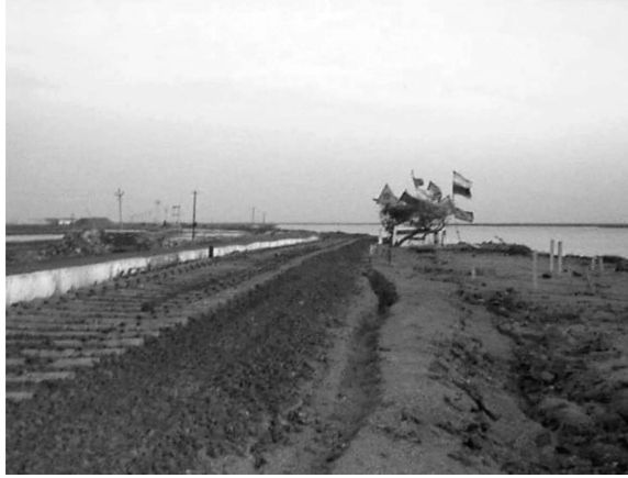
Figure 12.8 Lateral spreading next to a railway track at the Navalakhi port in Gujarat, India.
