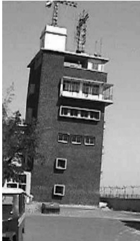
Figure 12.2 Rotation of a tall masonry building on pile foundations during the Bhuj earthquake.
