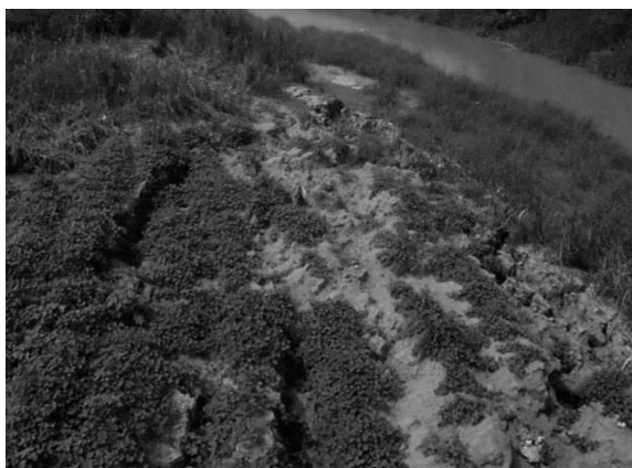
Figure 12.7 Lateral spreading of slopes of a river bank in Taichung, Taiwan.
