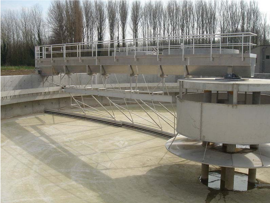
An empty sedimentation tank at the treatment plant in Merchtem, Belgium.
