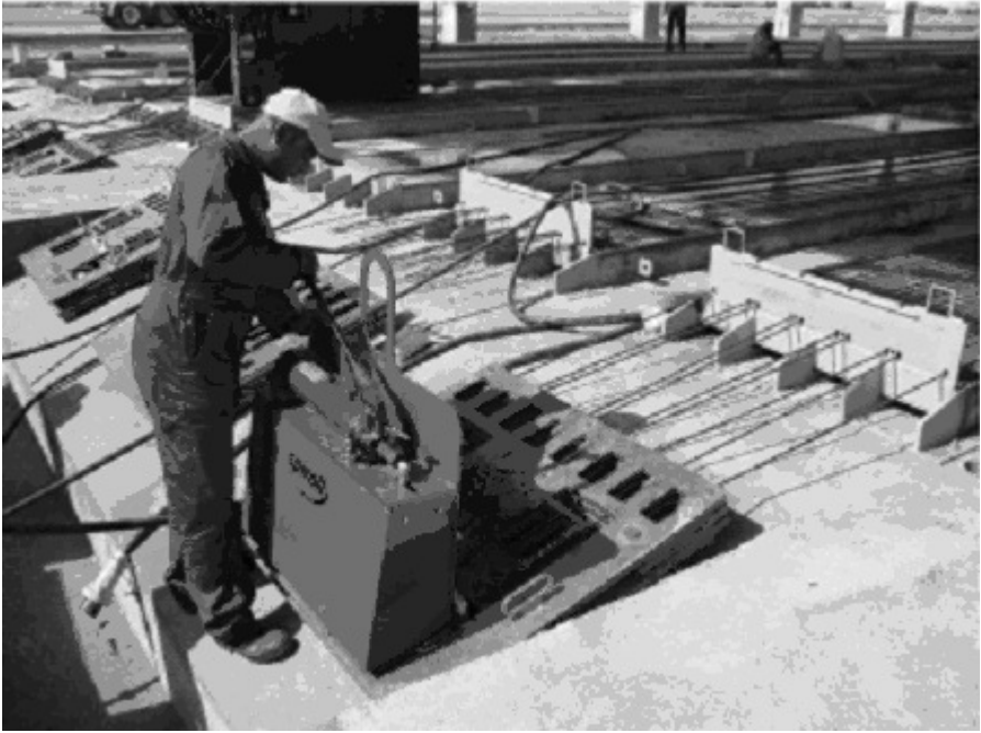
Fig. 2.2a Photograph of a pre-tensioning bed
