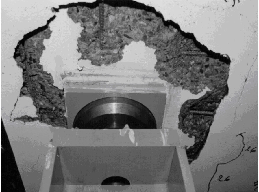
Fig. 13.1b Punching shear failure in a slab at a support
