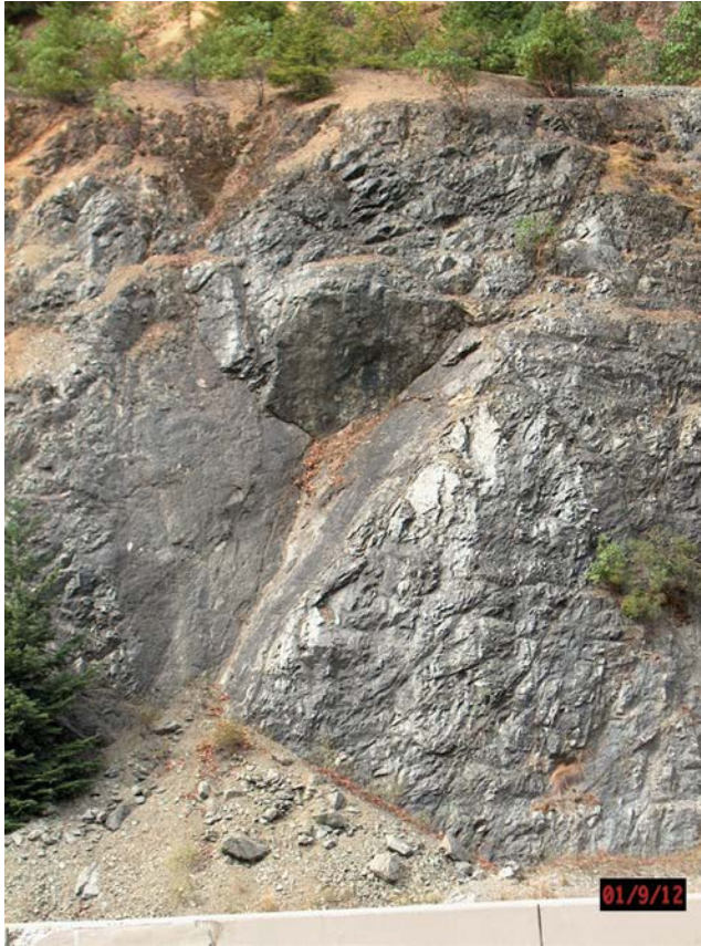
Figure 8.1 Typical wedge failure involving sliding on two persistent joints with line of intersection of joints daylighting at toe of rock face, and an upper plane that formed a tension crack (strong, volcanic rock on Interstate 5, near Grants Pass, Oregon).
