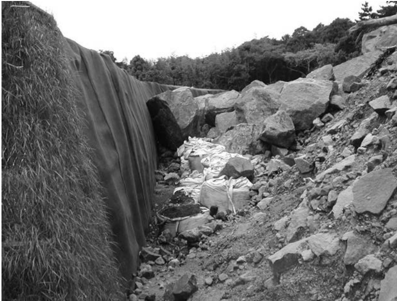
Figure 11.1 Rock fall induced by magnitude 6.4 earthquake on Niijima Island in Japan contained by an MSE wall (Protec Engineering, 2002).
