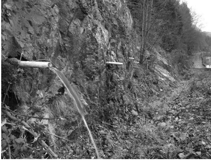
Figure 6.1 Horizontal drain holes, lined with perforated plastic pipes, in rock face; flow only occurs in holes that intersect water-bearing discontinuities (Sea to Sky Highway, British Columbia, Canada). (Image by J. K. McDonnell.)
