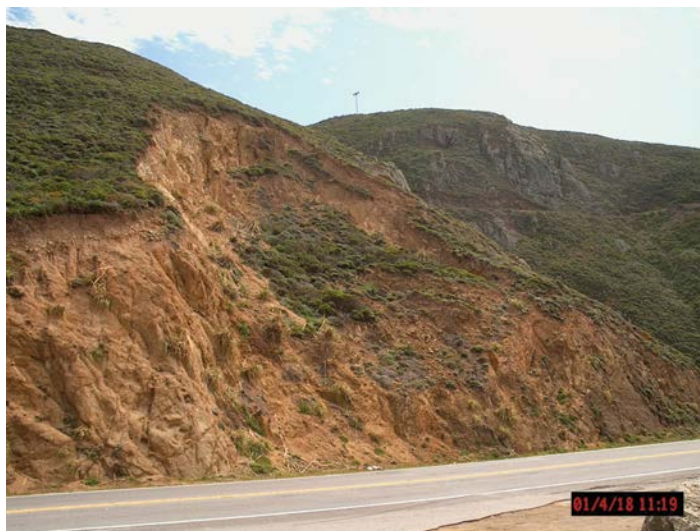
Figure 9.1 Circular failure in highly weathered, granitic rock (Highway 1, near Devil's Slide, Pacifica, California).
