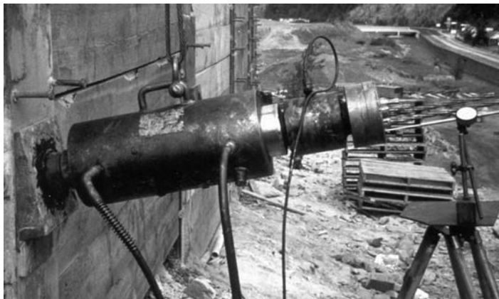
Figure 14.12 Test set-up for a tensioned multi-strand cable anchor comprising hydraulic jack load, and dial gauge on independent mount to measure anchor elongation. (Photograph by W. Capaul.)
