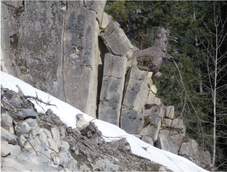
Figure 10.1 Toppling blocks in columnar basalt showing typical tension cracks with widths greater at the top and narrowing near the base (Sea to Sky Highway near Whistler, British Columbia, Canada).
