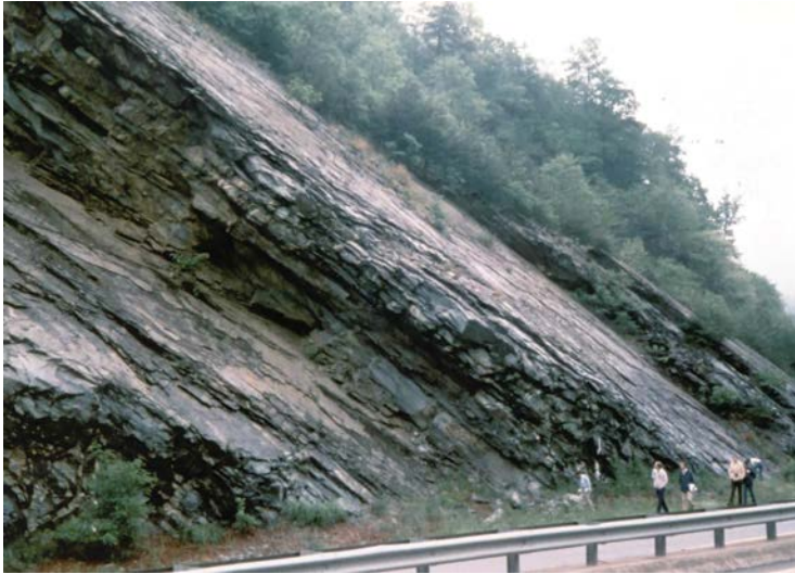
Figure 7.1 Plane failure on smooth, persistent bedding planes in shale (Interstate 40, near Newport, Tennessee).
