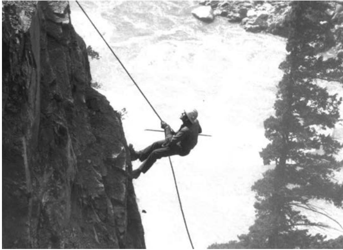
Figure 14.20 High-scaler suspended on rope and belt while removing loose rock on steep rock slope (Thompson River Canyon, British Columbia, Canada) (Transportation Research Board, 1996).
