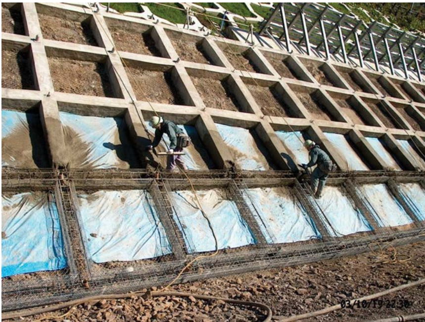
Figure 14.17 Construction of reinforced concrete grillage to support cut slope in weathered rock (near Niigata, Japan).
