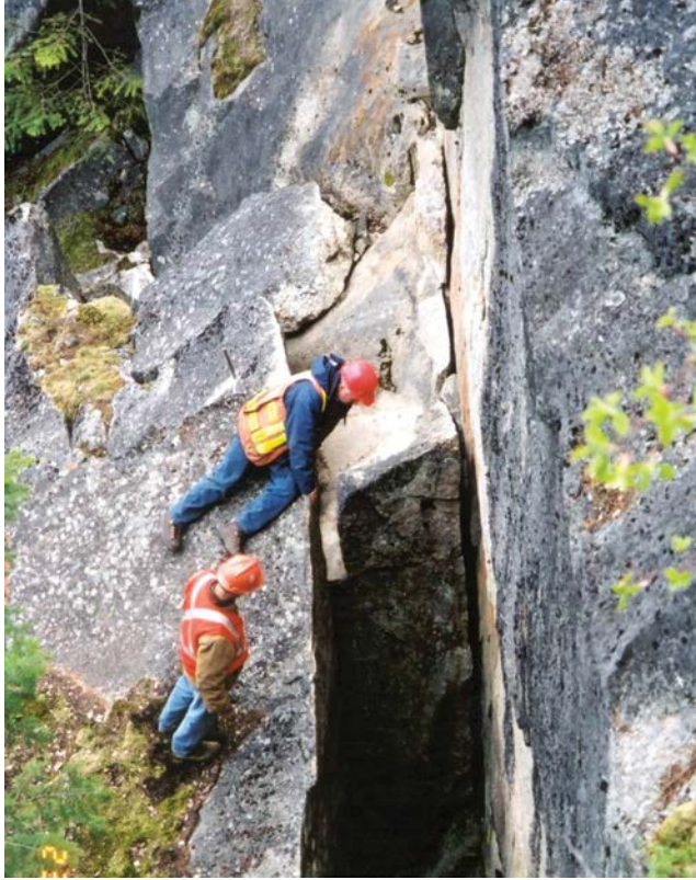
Figure 7.7 A tension crack behind a sliding rock mass in which significant horizontal displacement has occurred (above: Kooteney Lake, British Columbia).
