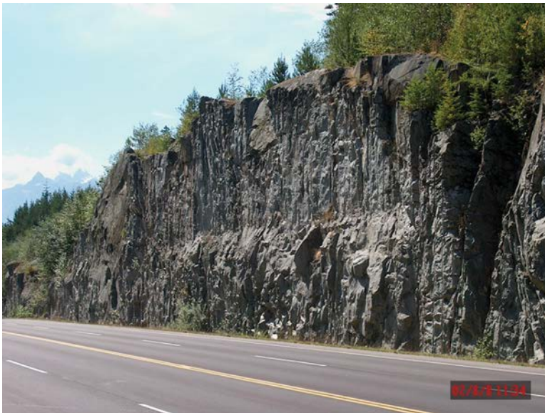
Figure 13.10 Example of controlled blasting, with drill 'offset' at mid-height for rock cut on highway project (strong granite, Sea to Sky Highway, British Columbia, Canada).
