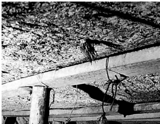
Figure 4 Development of the lower third of the seam revealing the pre-installed wooden dowel reinforcement of the septum. Source: O'Beirne, 1982
