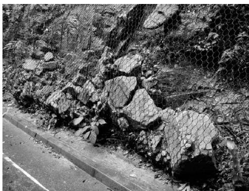
Figure 10 Minor rockfalls contained by rock mesh avoiding impact on the adjoining carriageway.
