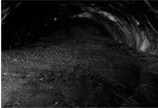
Figure 3 Flow of clay matrix along with highly disintegrated and weathered rock mass from tunnel face at Ch. 2077m (Rao & Sharma, 2014).
