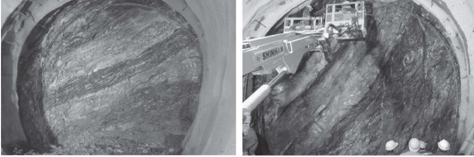
Figure 11 Coal-bearing layer at the face (left) and installation of lattice girder (right) in Sol-an Tunnel.
