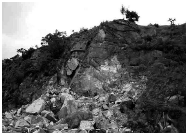
Figure 17 The 2008 Tsing Yi Road rockslide.
