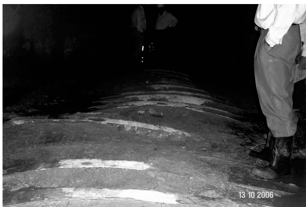
Figure 5 Floor heaving in a railway tunnel in J&K, India.
