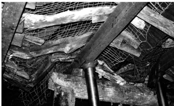
Figure 9 Mesh supporting the roof of the lower slice in the maingate/face-end area of a multi-slice longwall.
