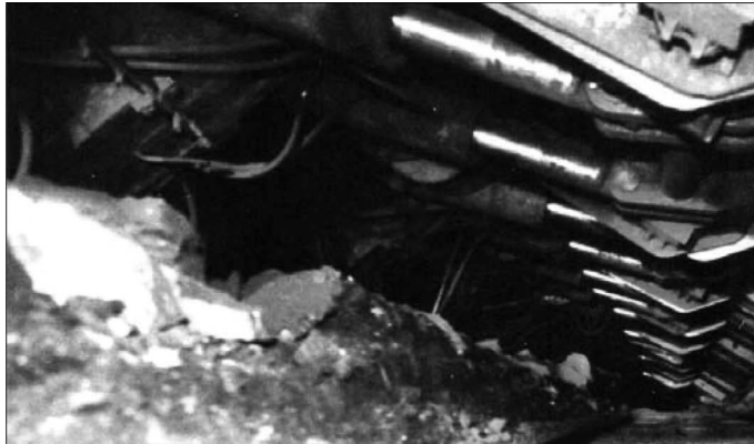
Figure 20 Rear AFC area of an operating LTCC face.
