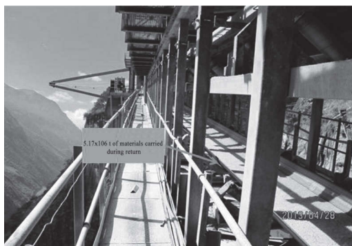
Figure 18 Transportation of materials during return of belt conveyor.
