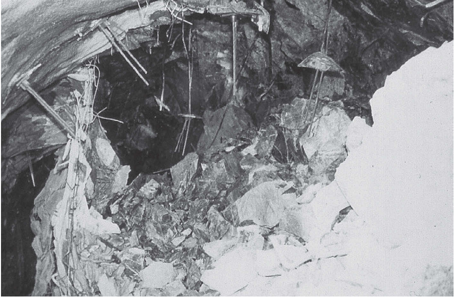
Figure 2 Exposed, protruding cables after a rockburst (Stacey & Rojas, 2013).
