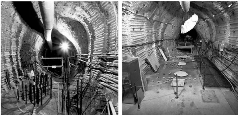
Figure 11 The Heated Failure Tests at the 420 Level: installation of instrumentation borehole casing in invert of widened MBE test tunnel (left), and completed experiment construction (right).
