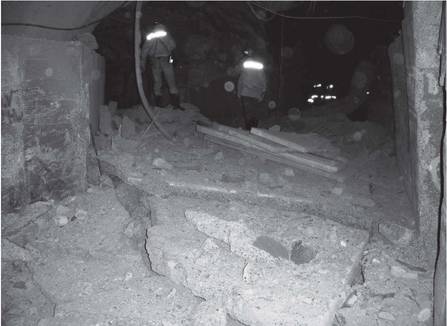
Figure 3 Floor heave of nearly 2m caused by a rockburst (Stacey & Rojas, 2013).
