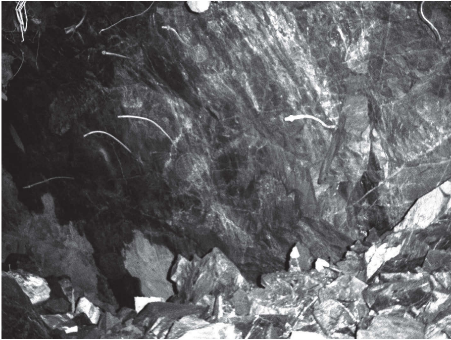
Figure 7 Rockbolt inclinations indicating upwards direction of ejection (Stacey & Rojas, 2013).
