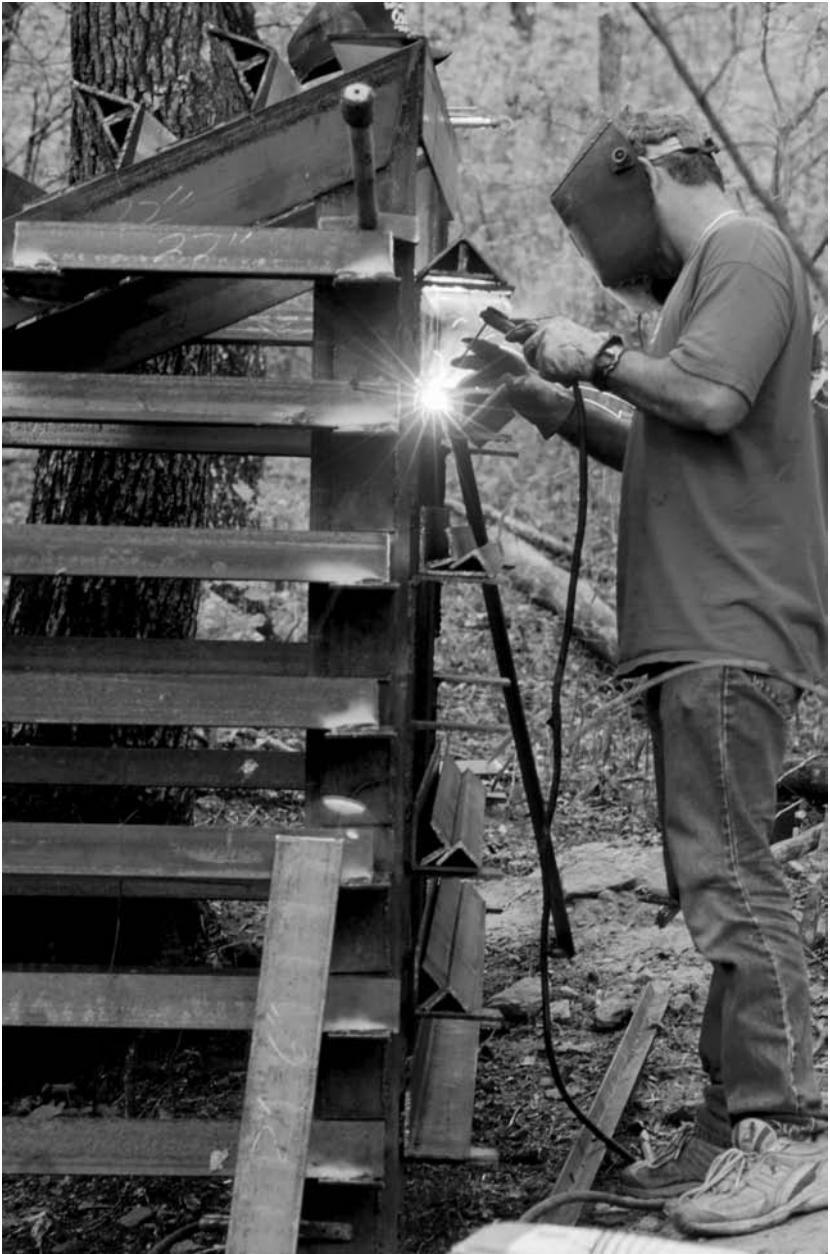
Figure 5.6 Building a bat gate above a sink opening. Photo by Danté Fenolio. (See Plate 21.)
