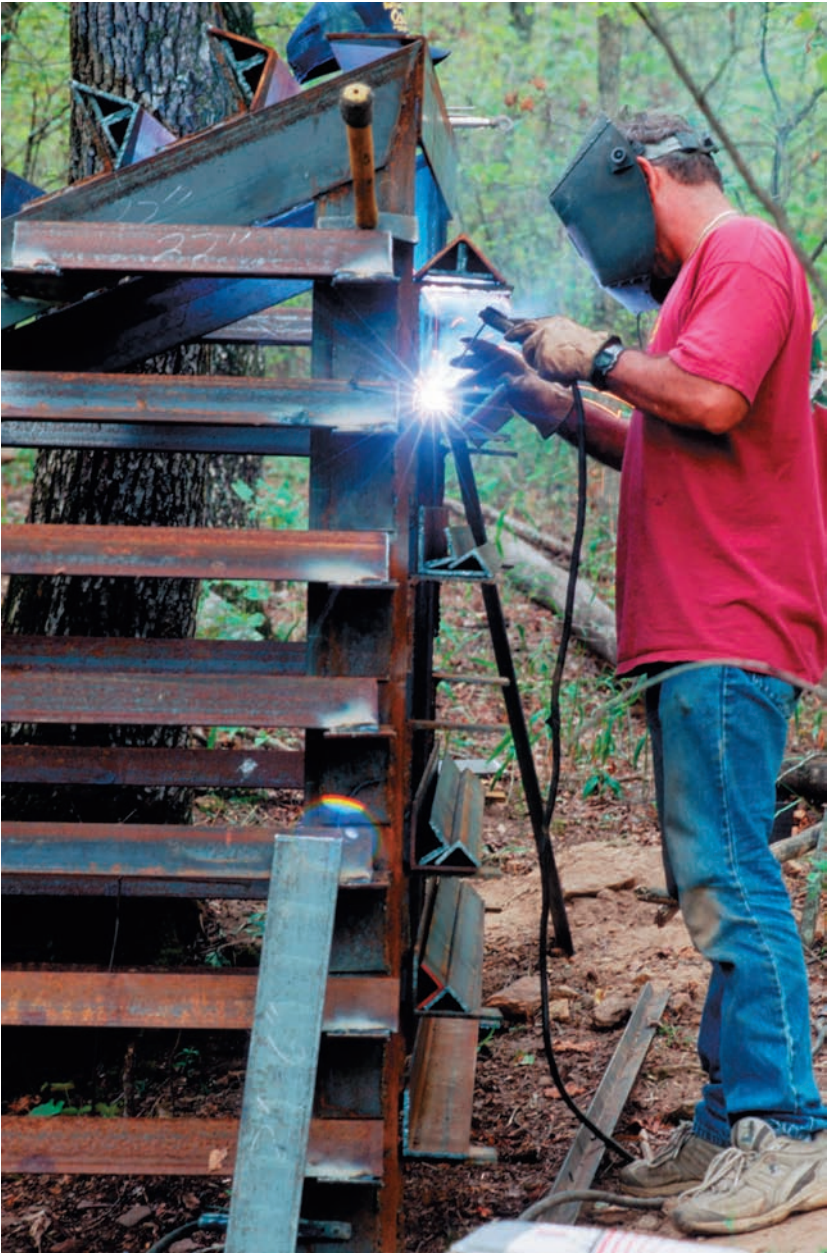
Plate 21 Building a bat gate above a sink opening. Photo by Danté Fenolio.
