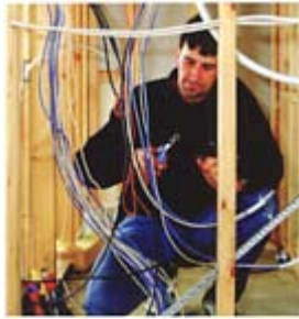
Above: Mawson Lakes homes are fully wired with an extensive digital communications infrastructure
