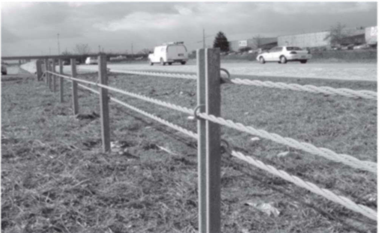
Figure 6.6 U.S. High-Tension Cable System
