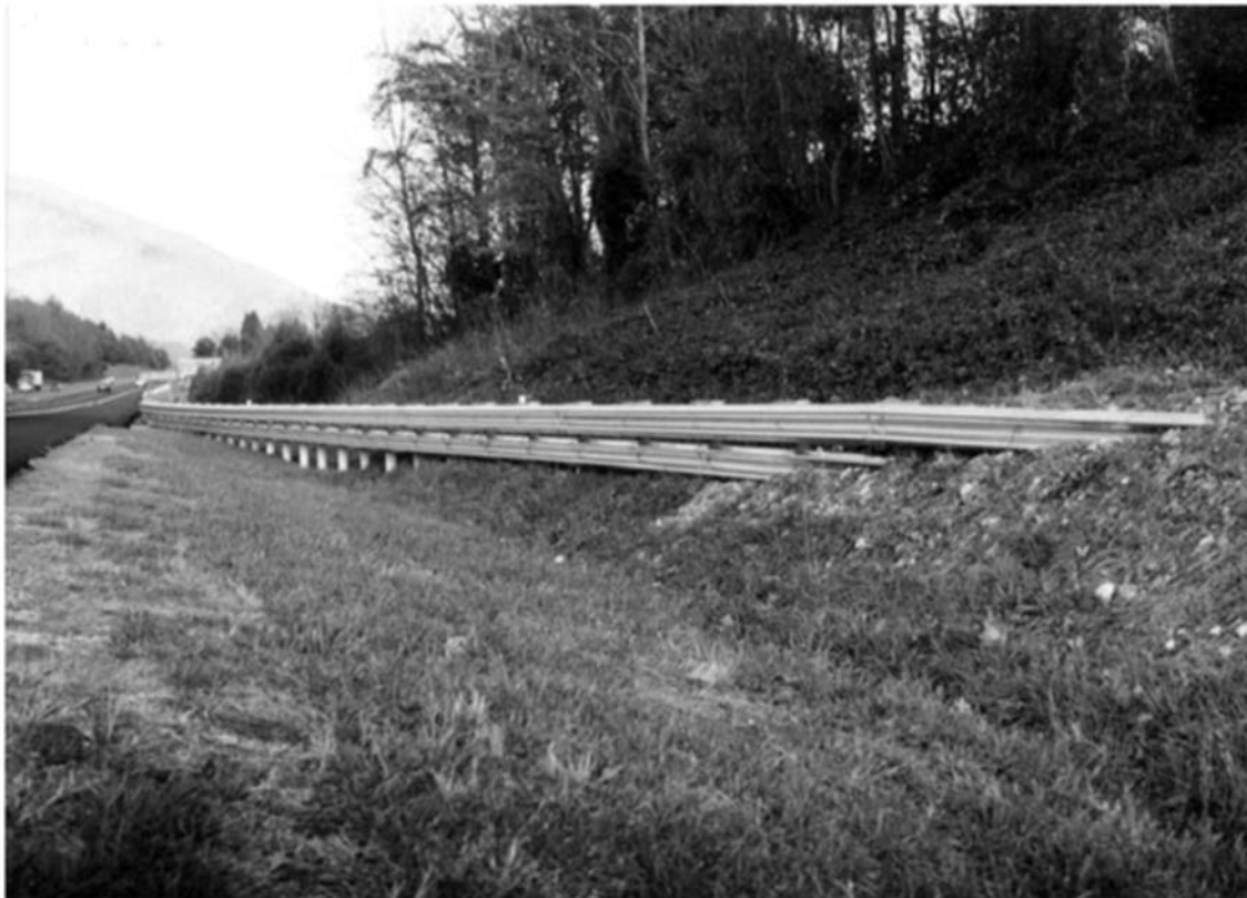
FIGURE 8.6 W-beam guardrail anchored in backslope
