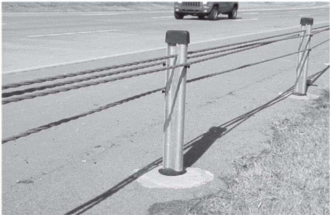
Figure 6.4 Brifen Wire Rope Safety Fence
