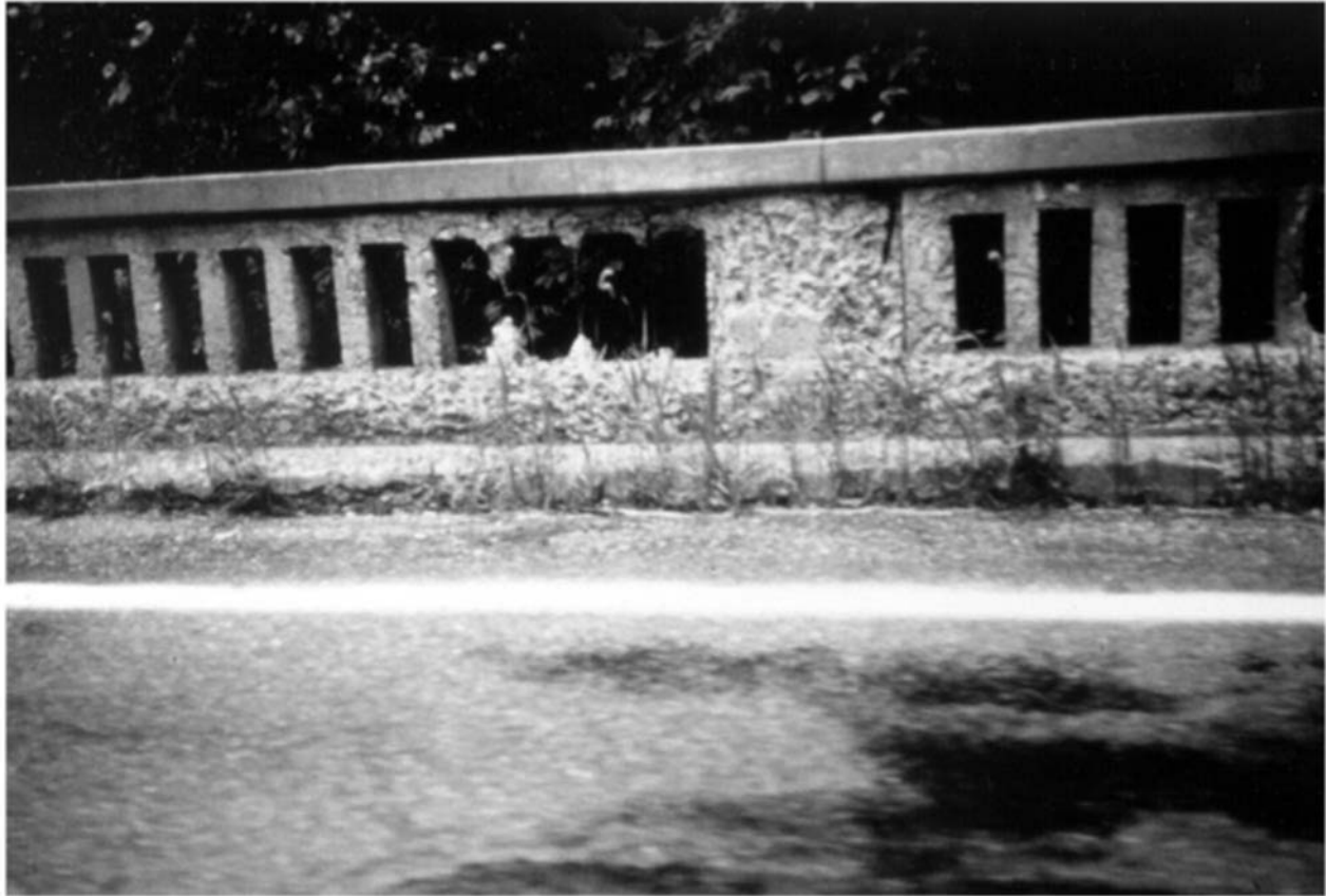
FIGURE 7.9 Inadequate railing strength
