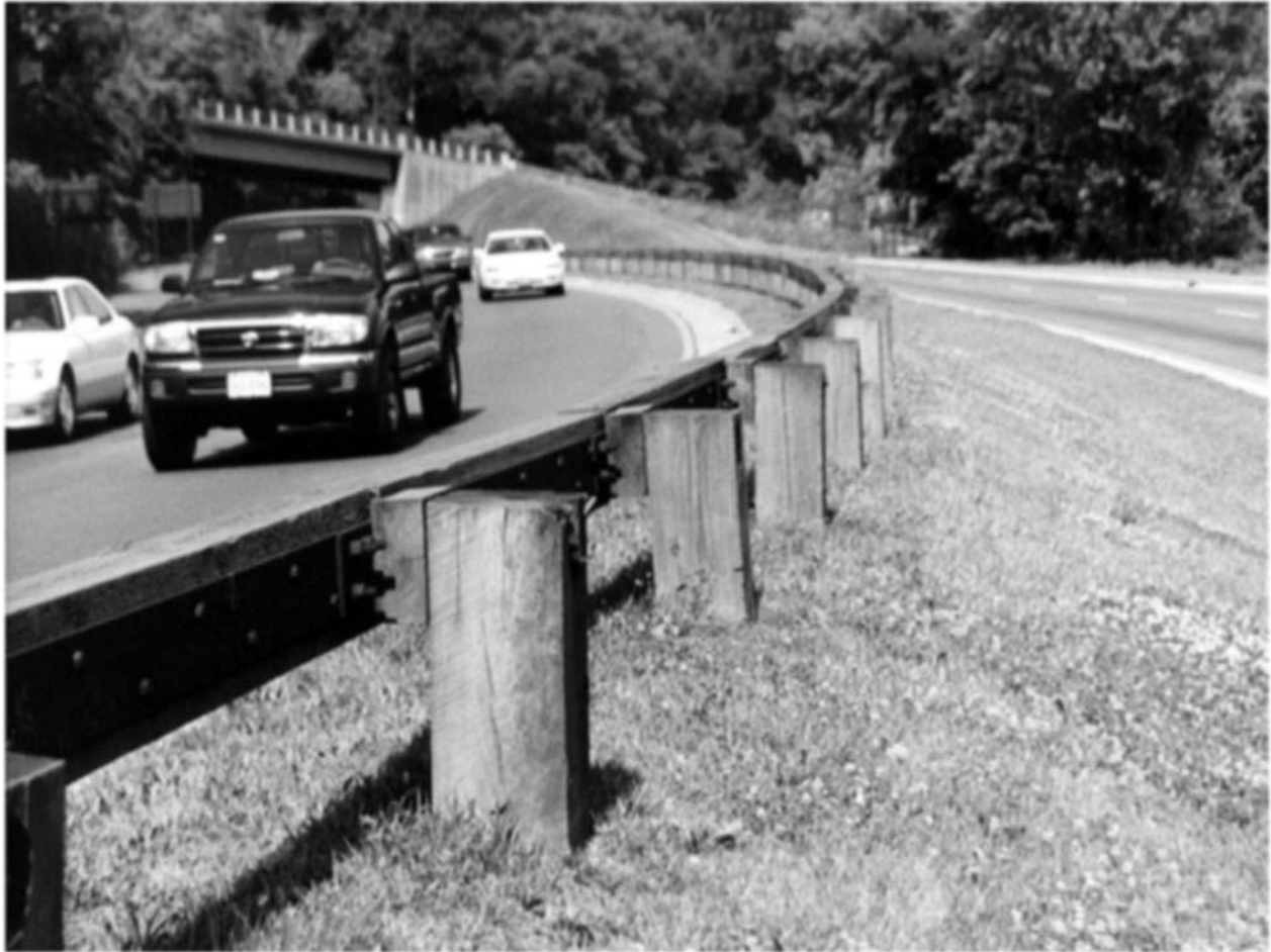
FIGURE 5.14 Steel-backed timber guardrail
