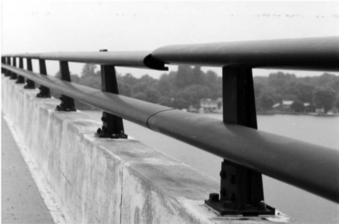
FIGURE 7.10 Lack of continuity in railing
