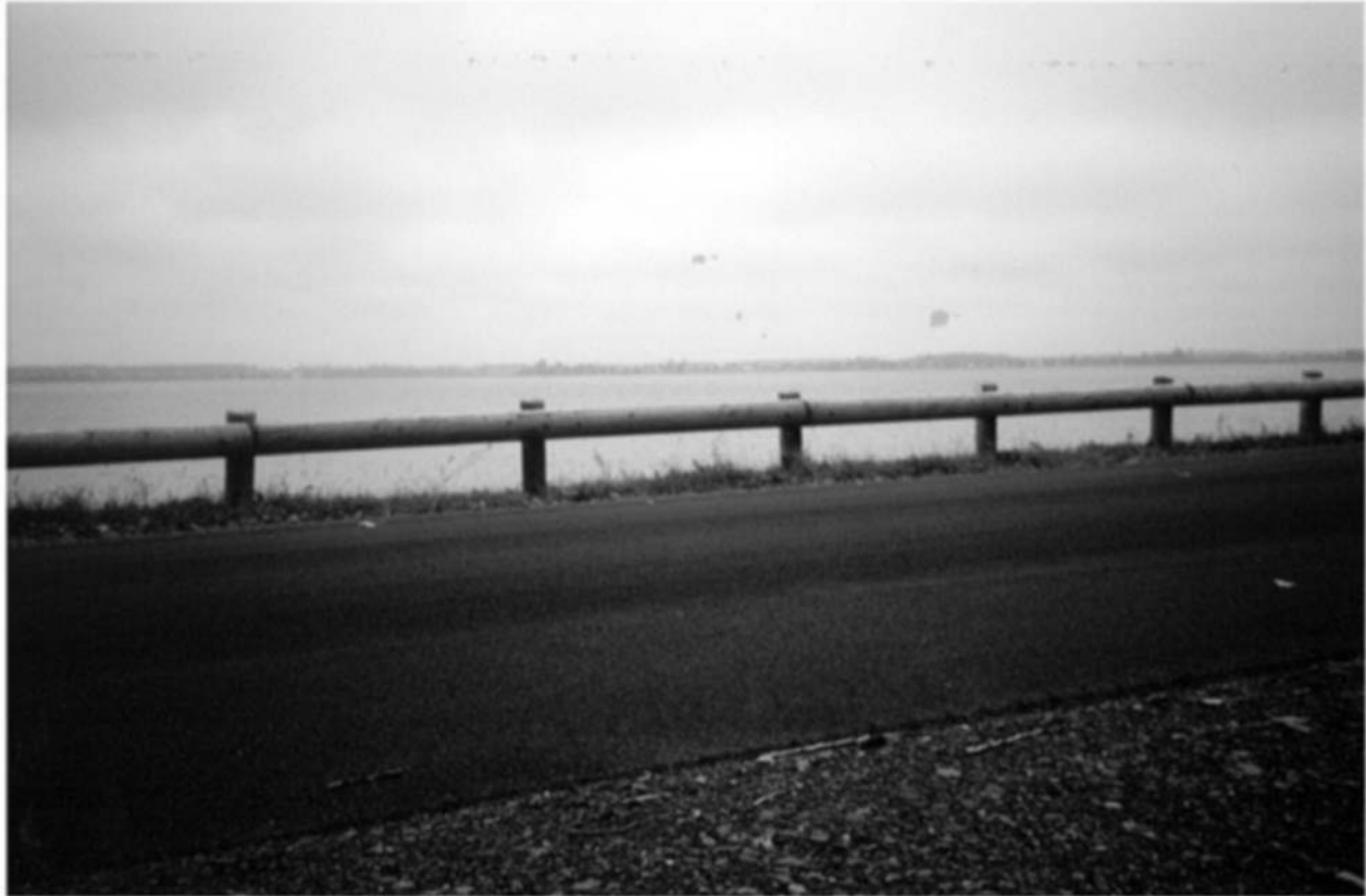
FIGURE 5.7 Ironwood aesthetic guardrail
