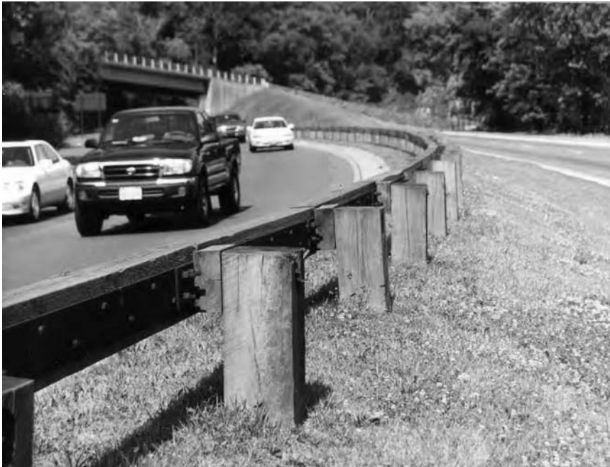
Figure 5-18. Backed Timber Guardrail
