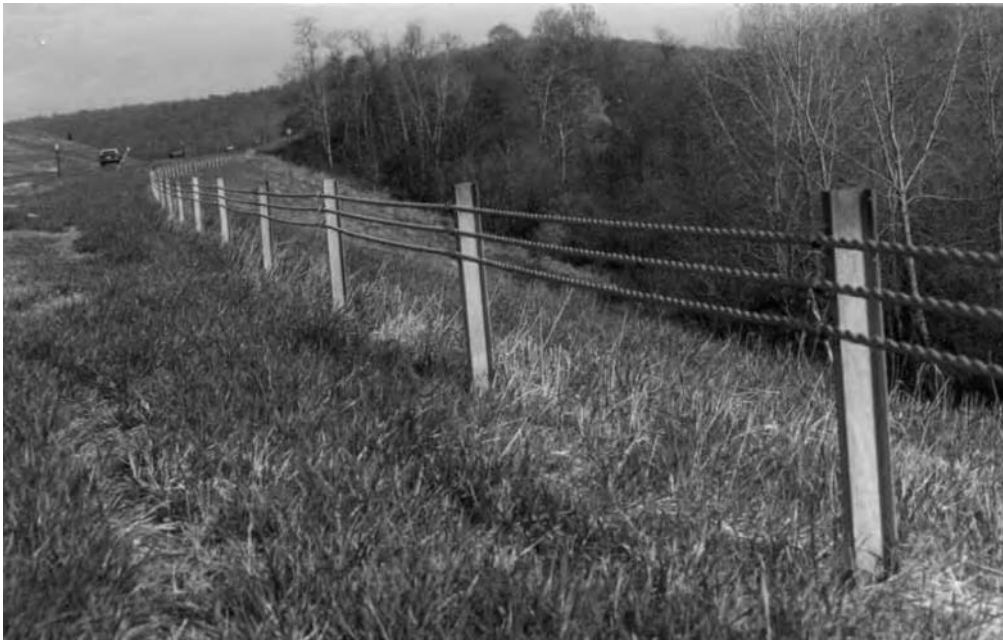
Figure 5-5. Three-Strand Cable Barrier
