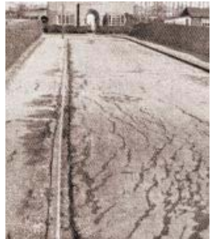
Figure 1.33 Shrinkage cracks in a road and pavement on London Clay indicating desiccation by trees
