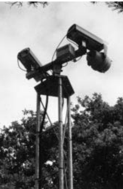
Figure 5.39 Column mounted CCTV equipment
