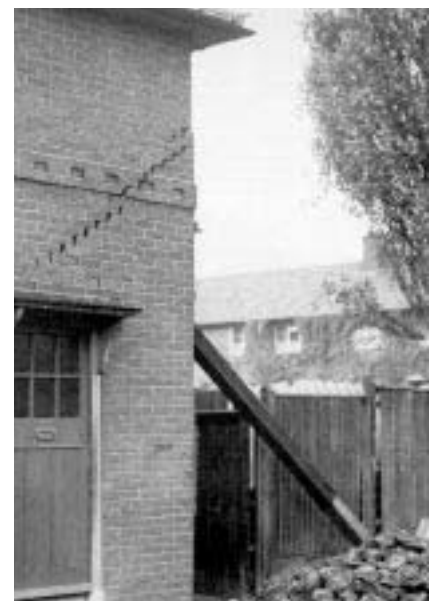
Figure 1.30 A cracked corner of a house near a Lombardy poplar tree
