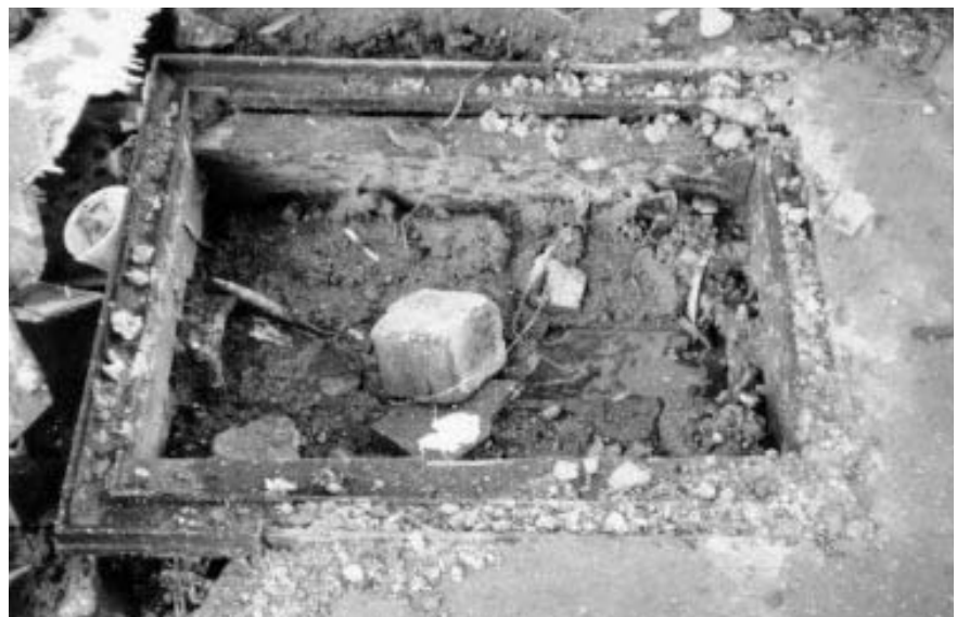
Figure 4.18 Builders' rubble entering an uncovered manhole during refurbishment work
