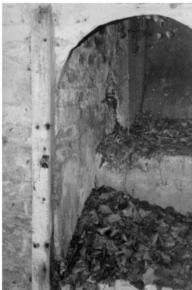
Figure 3.2 A coal cellar (with accumulated leaves) from the nineteenth century which has remained derelict for many years
