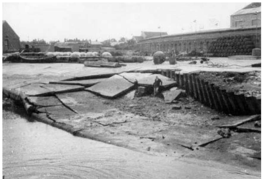
Figure 5.7 Failure of a sheet pile wall
