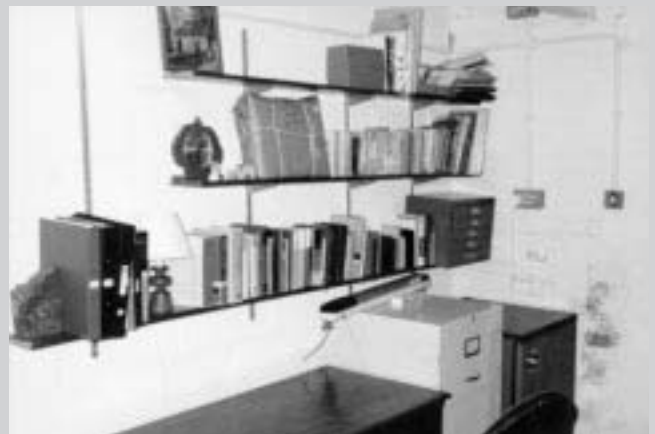
Figure 3.34 Items stored in a basement adjacent to that illustrated in Figure 3.33. Sufficient heat was emitted from the small freezer to keep the moisture levels below dewpoint
