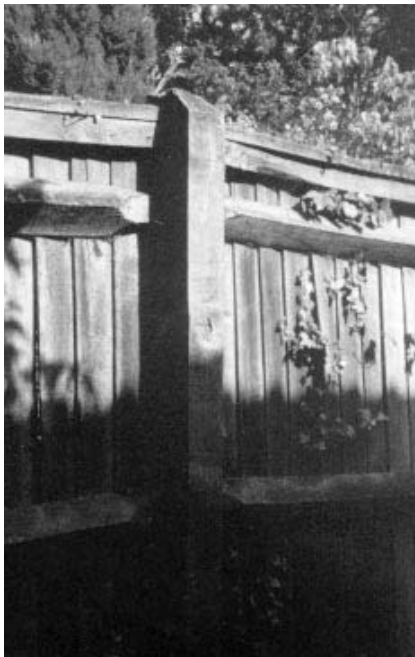
Figure 5.30 Non-preservative treated oak fence to BS 1722 after 20 years life
