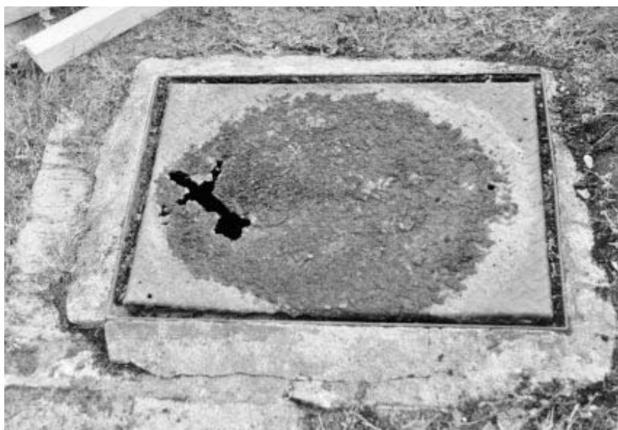
Figure 4.17 A 20 year old steel manhole cover which has suffered serious corrosion
