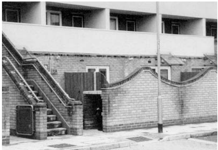
Figure 5.20 An urban brick boundary wall in stretcher bond. The design of the coping makes it inevitable that rainwater run-off will disfigure the front face
