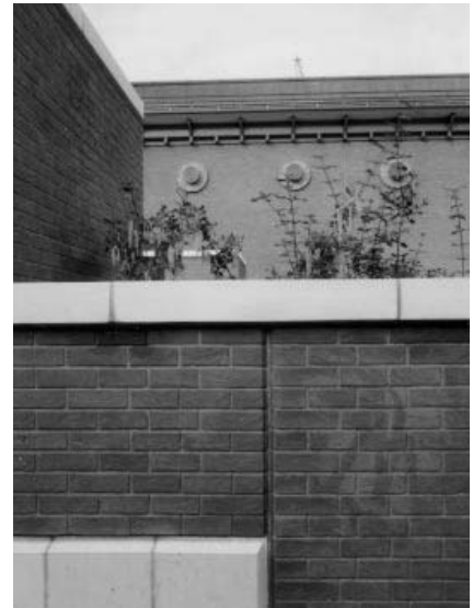
Figure 5.19 A boundary wall of a prestige building. Although the coping is substantial in size, it does not respect the movement joint beneath, with risk of subsequent distress
