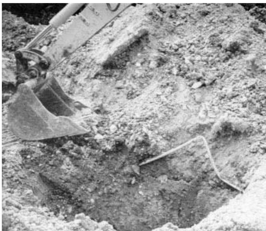
Figure 4.1 A lead water main caught by an excavator bucket while digging a soakaway. The water main did not leak – perhaps because one of the few advantages of lead being its ductility
