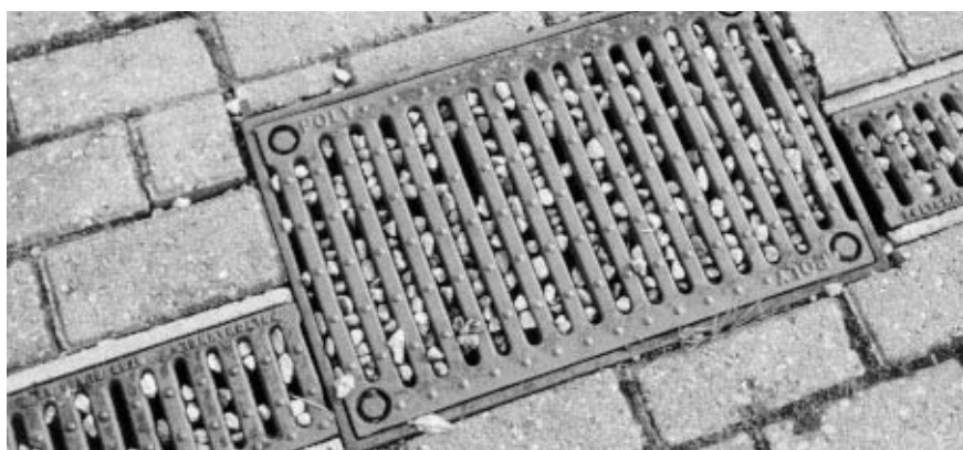
Figure 4.24 An elementary error. Pea shingle from an adjacent area has more-or-less completely blocked these drainage grilles
