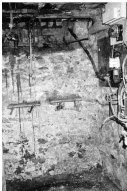
Figure 3.27 Services in the cellars of older properties are frequently maintained in hazardous and damaging conditions
