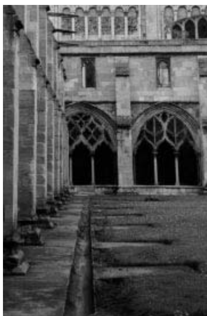
Figure 4.21 An open drain taking the discharge from the gargoyles in the cloisters at Norwich Cathedral
