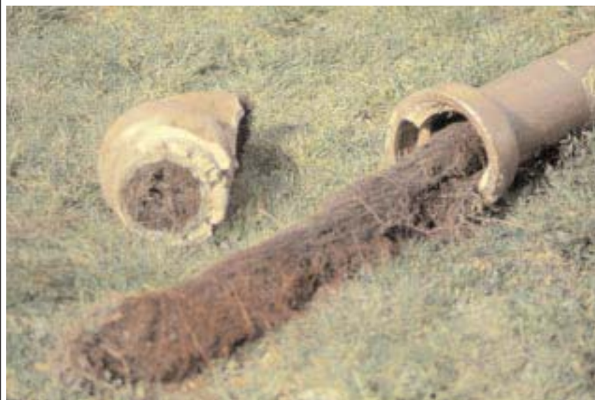
Figure 4.26 Tree roots entering this clayware drain through joints have completely filled it (Photograph by permission of John Bricknell)
