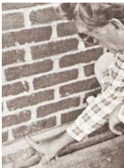
Figure 1.18 Undersailing of brickwork below the DPC caused by expansion in the floor slab. The amount of movement is shown as about half a finger's length
