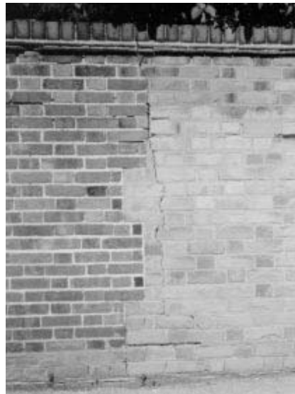
Figure 5.18 A brick which is insufficiently durable for a freestanding wall is block bonded into an adjacent stretch of wall in another type of brick, but there is no movement joint. The wall has therefore created its own movement joint in the form of a crack
