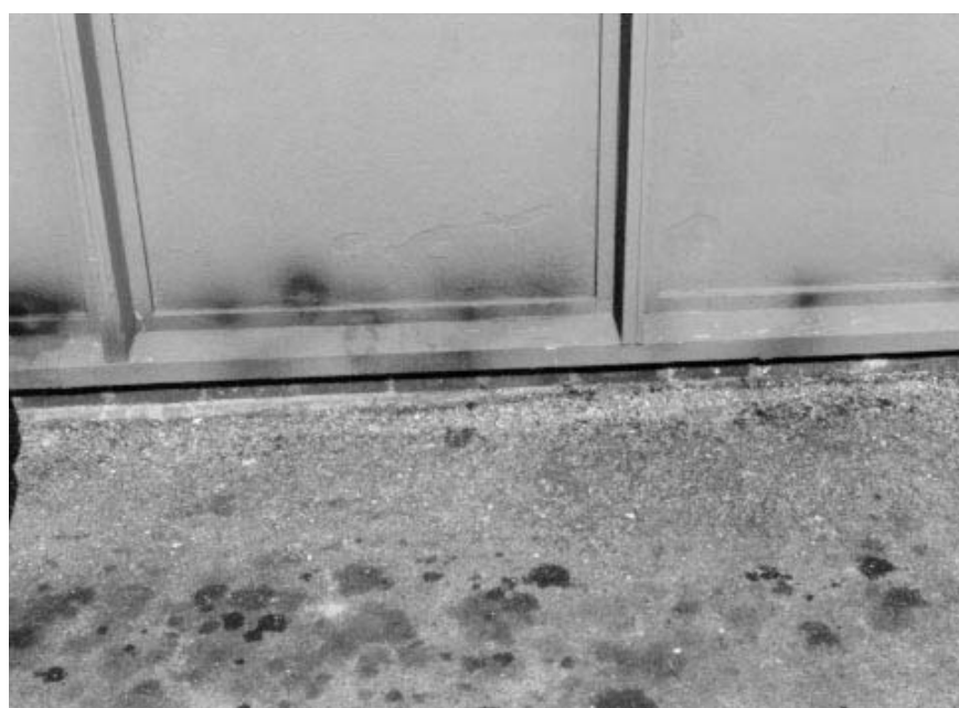
Figure 6.5 Cars parked too close to a building leave exhaust marks on the fabric. Oil which has dripped from parked vehicles onto paved surfaces permanently damages those surfaces (at worst) or disfigures them (at best)
