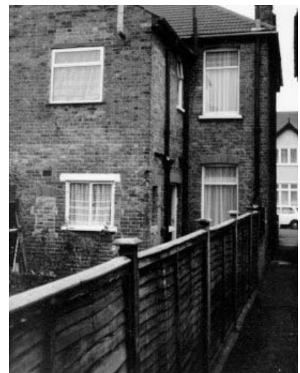
Figure 5.24 Lapped wood fencing panels. In this situation, lining a public footpath, the panels will probably not survive more than a few years
