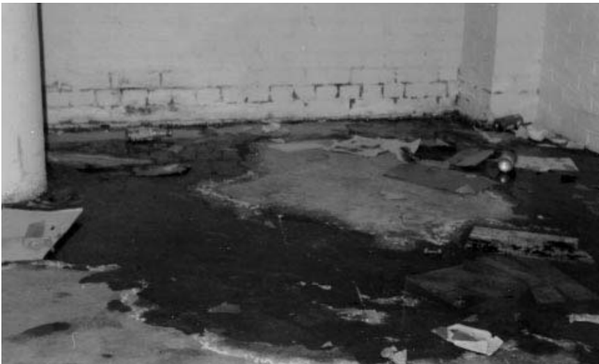
Figure 3.11 Flooding in a basement. The lower courses of brickwork are also saturated
