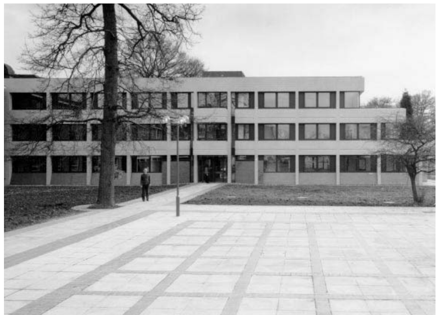
Figure 6.11 Fired clay pavers interspersed with concrete flags . Many of the pavers subsequently failed as a result of frost action during a 10 year service life
