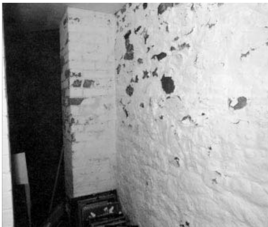
Figure 3.10 Salts from dampness in the structure is one of the problems to be faced in converting a basement to living accommodation
