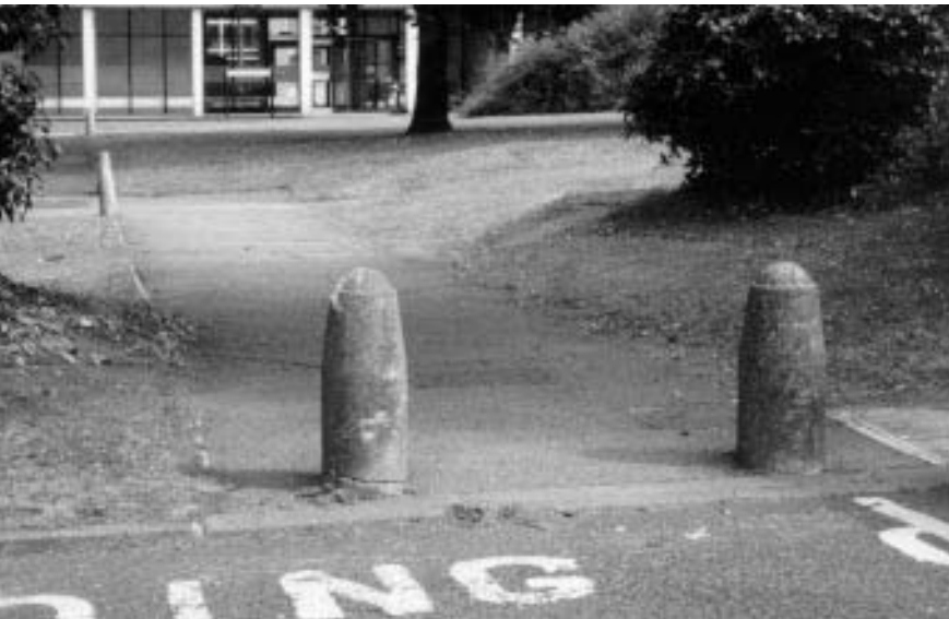
Figure 6.12 The scars and damage to the concrete bollard on the left show just how necessary protection can be
