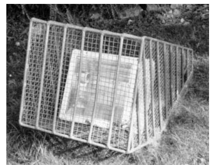
Figure 5.36 One of the ground mounted floodlights for the church tower shown in Figure 5.35
