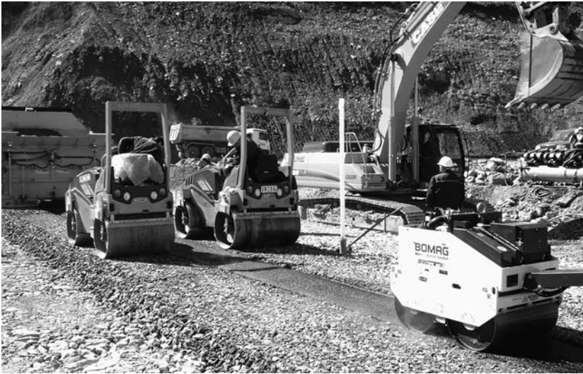
Figure 14.28 Knezhevo dam, compaction of the just placed transition and asphaltic concrete layers.
