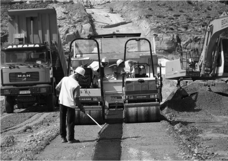
Figure 14.15 Synchronized compaction of the transition layers of both sides of the asphaltic core.
