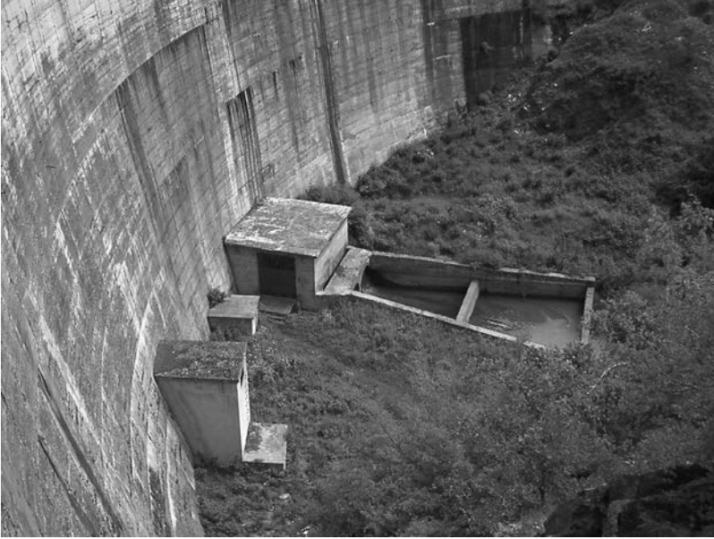
Figure 28.3 The terminal part of the bottom outlet of the Gratche dam (Macedonia).
