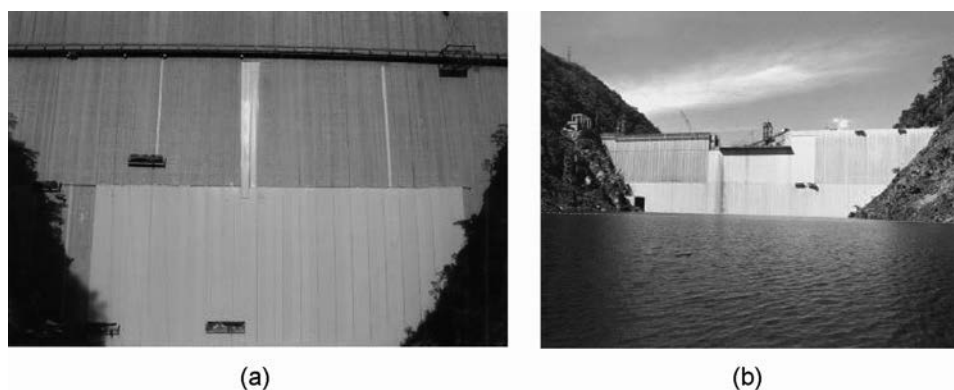
Figure 18.23 Miel I dam. (a) PVC installation almost completed in lower section, and starting in the section above, where placement of the support geocomposite on the contraction joints is being performed from the travelling platform; (b) the PVC geocomposite, already installed in the lower sections allowed impounding the reservoir, while RCC placement and waterproofing works were ongoing above (Vaschetti and Scuero, 2009).
