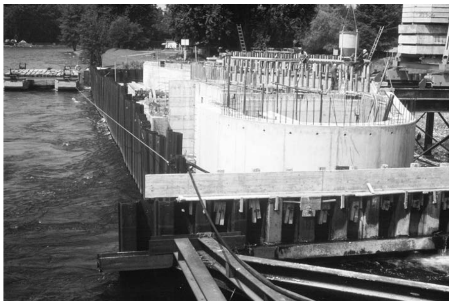
Figure 30.3 Construction of parting wall on the river Aar, in the vicinity of Zürich, under the protection of a steel sheet piling partition.
