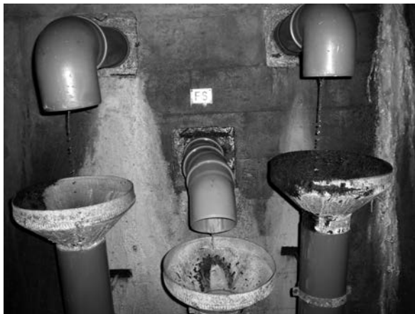
Figure 14.36 One of the seepage measuring points in the gallery of Finstertal dam (photograph taken in September 2010).
