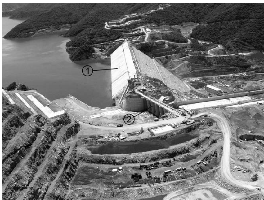
Figure 12.43 El Cajón dam at final construction stage. (1) Upstream dam face; (2) controlled spillway.
