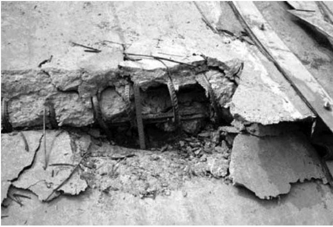
Figure 9.28 An illustration of the damage to a reinforced concrete slab of the Zipingpu dam in horizontal direction.
