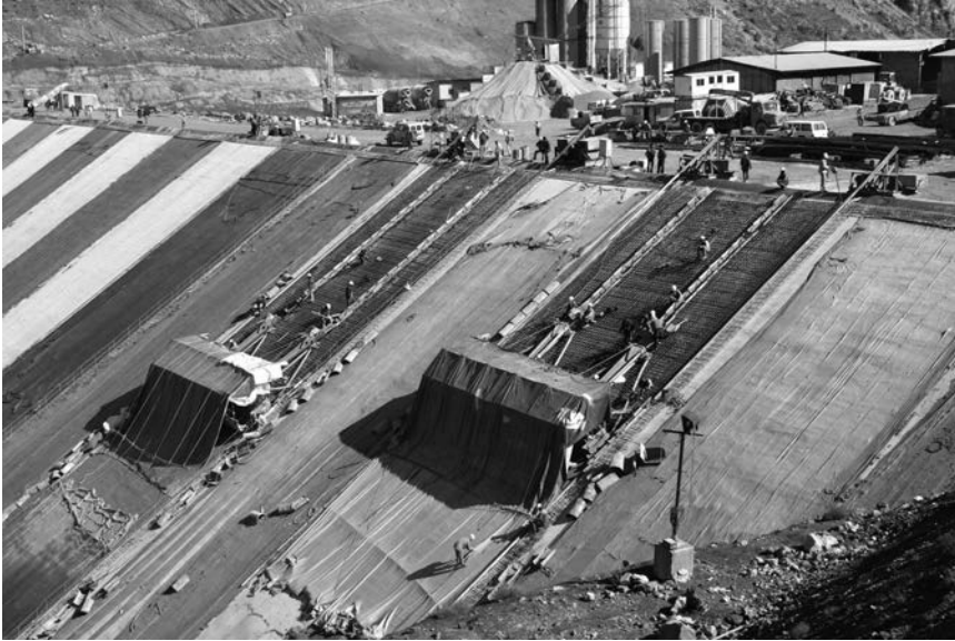
Figure 12.26 Siah Bishe Lower dam (Iran, H = 128 m), during the final stage of facing slabs construction, in 2009 (courtesy Mr. Lotfali Modarres).
