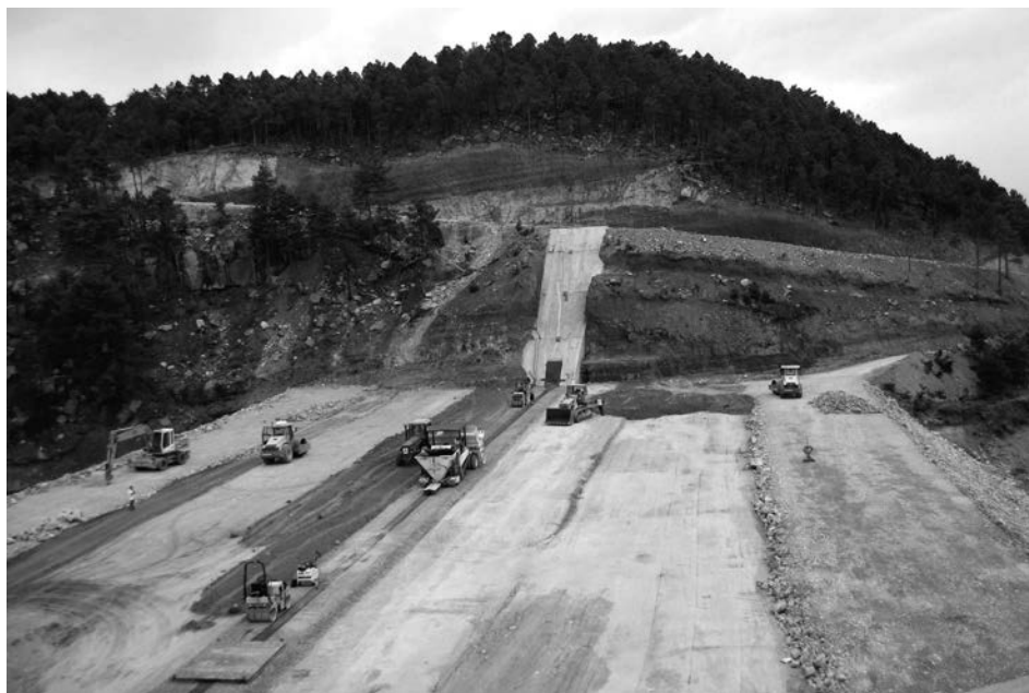
Figure 14.14 General view of the dam construction site, Mora de Rubielos dam, Spain, 2005.
