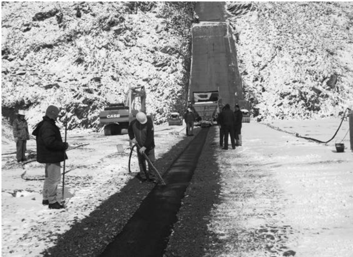
Figure 14.29 Knezhevo dam, light snow is not a serious obstacle for the placement of asphaltic concrete layers as long as the air temperature is not lower than 5°C.
