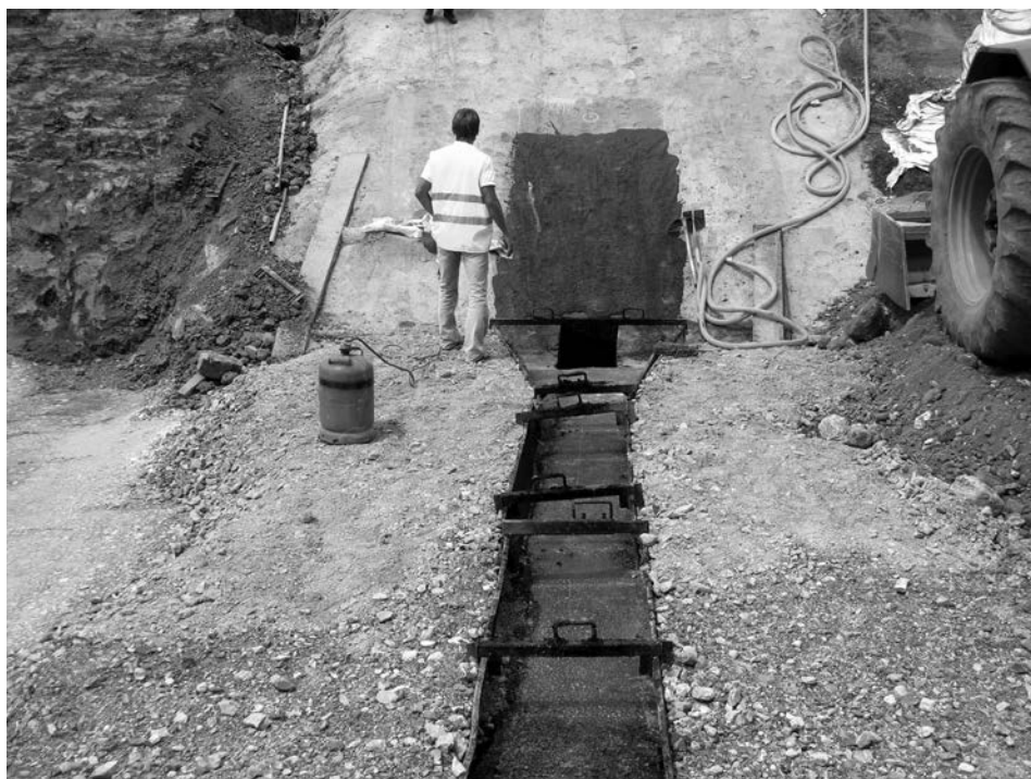
Figure 14.17 Framework prepared for hand-placement of the asphaltic concrete in the end of the core (near an abutment), inaccessible for the placement machine.
