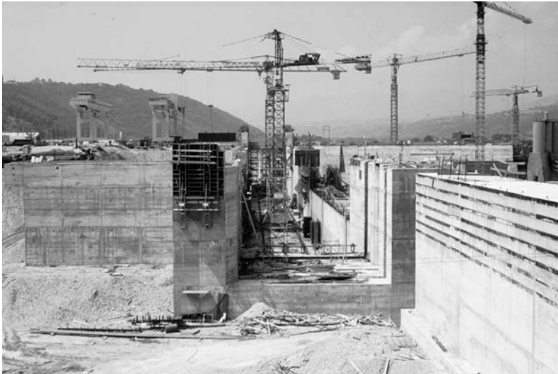
Figure 29.4 The ship navigation lock at one concrete gravity dam on River Rhone (France), under construction (1979).
