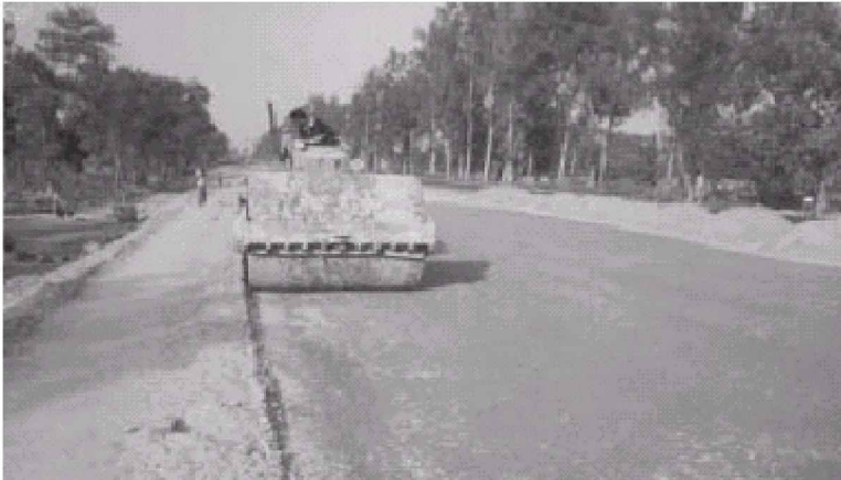
Figure 13.13 WMM work in progress at km 67 of NH-25 (Courtesy: NHAI and ICT Ltd., Kanpur).
