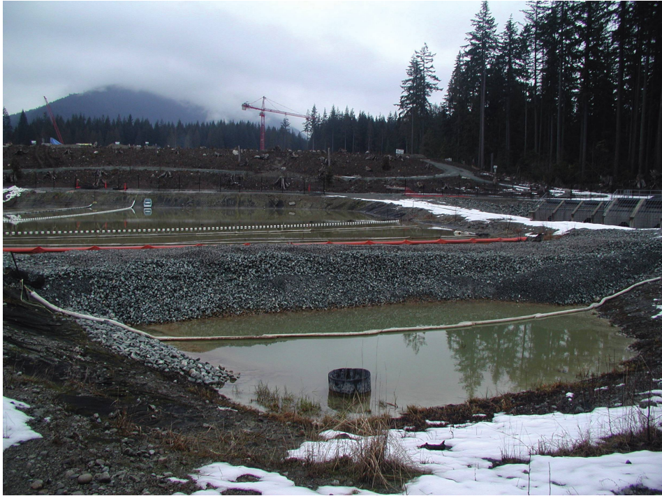
Figure 11.3 Construction water treatment ponds.
