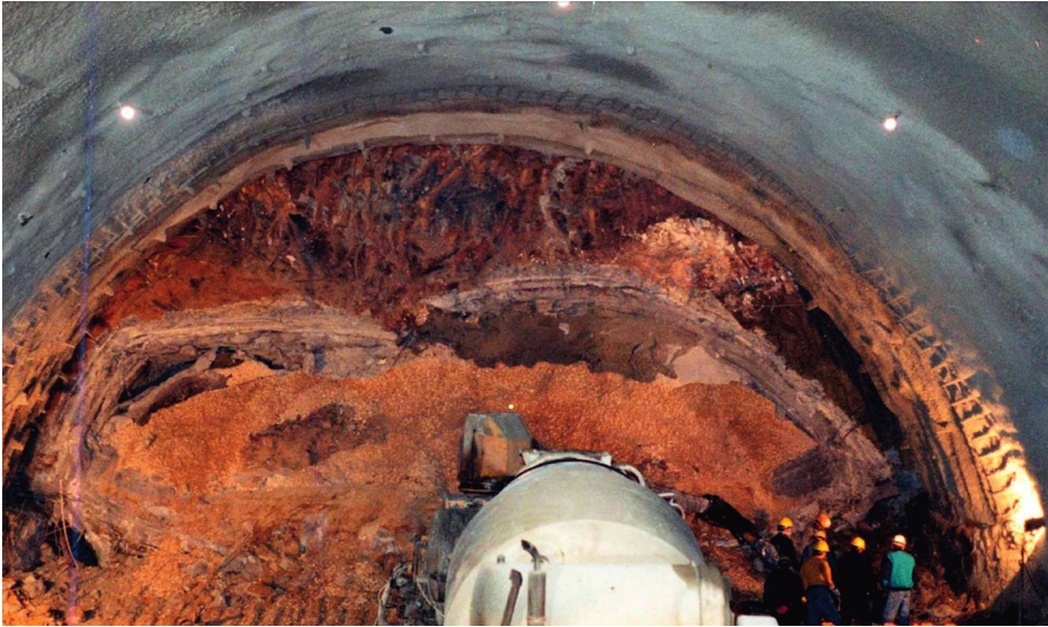
Figure 19.4 Severe deformation and damage of large tunnel.
