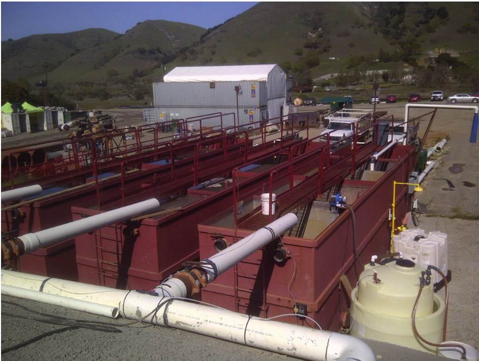
Figure 11.2 Construction water treatment system.
