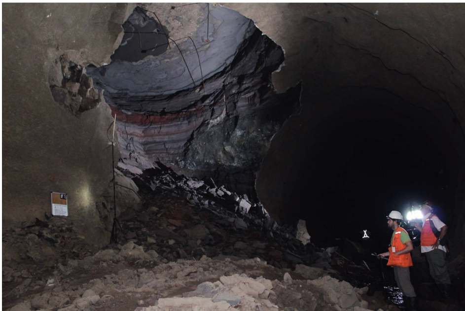
Figure 5.8 Tunnel collapse of expansive volcanic rock after 9 years of saturation.
