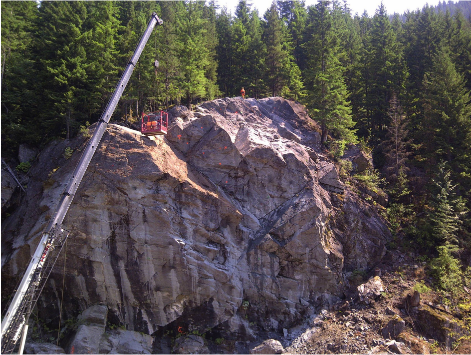
Figure 9.1 Installation of long rock bolts at tunnel portal for stabilization of large wedge.
