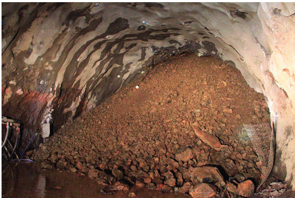
Figure 7.11 Unstable materials at major geological fault zone.
