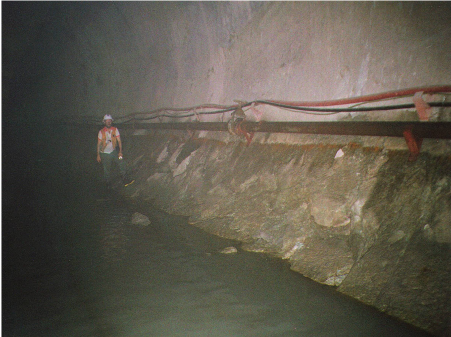
Figure 5.6 Deterioration of andesite during construction.
