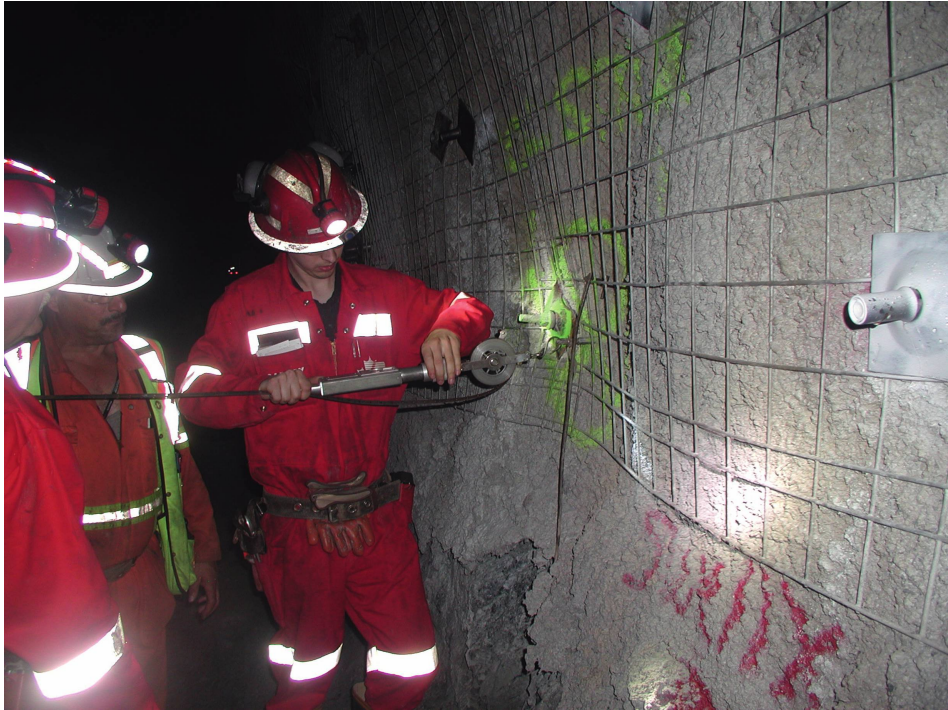
Figure 11.7 Geotechnical instrumentation – tape extensometer.
