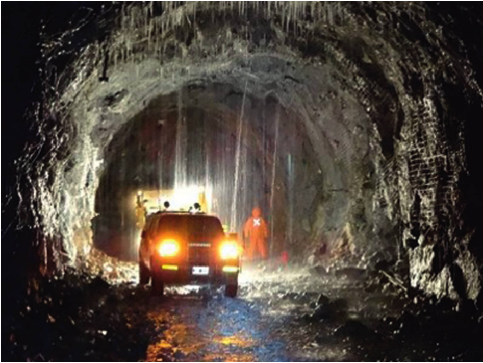
Figure 19.16 Highly acidic groundwater inflows.
