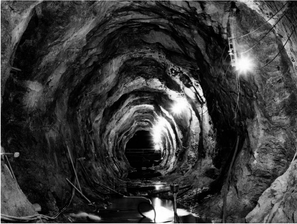
Figure 8.1 Large overbreak along historical tunnel.
