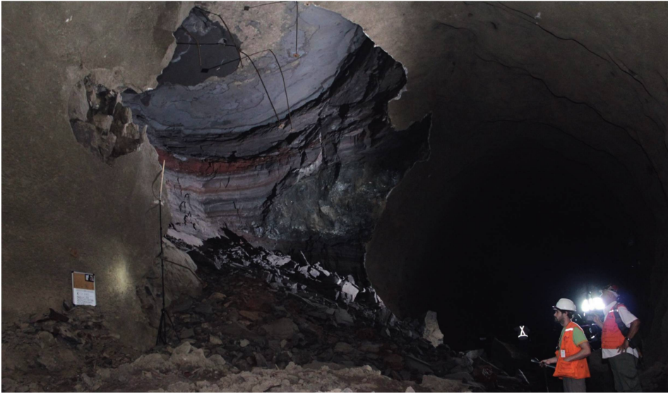
Figure 19.12 Tunnel sidewall collapse of non-durable volcanic rock.
