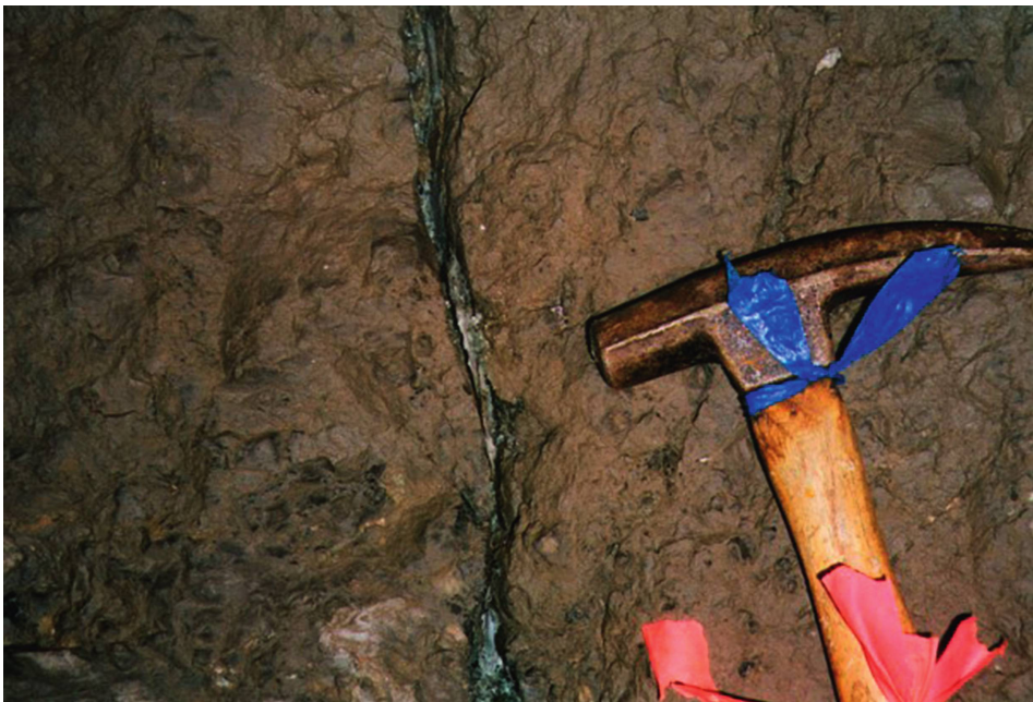
Figure 5.7 Dissolution of anhydrite filled fracture during construction.
