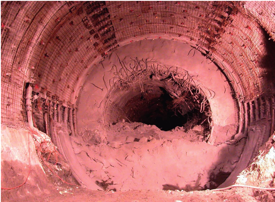
Figure 7.12 Squeezing conditions at TMZ Gotthard Base Rail Tunnel.
