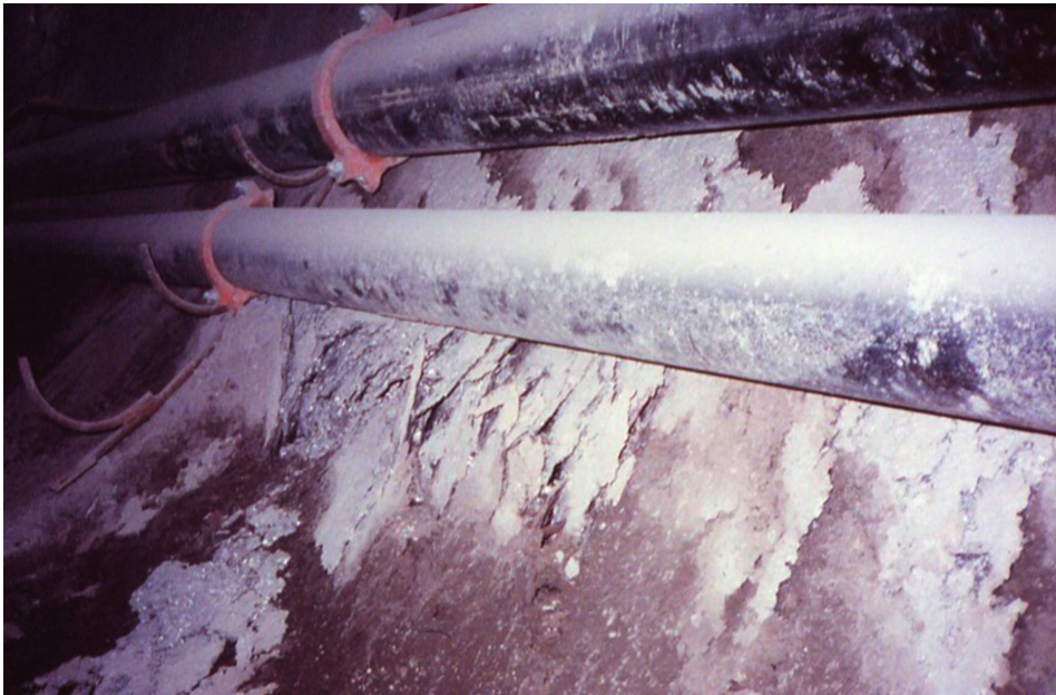
Figure 5.5 Deterioration of basalt during construction.
