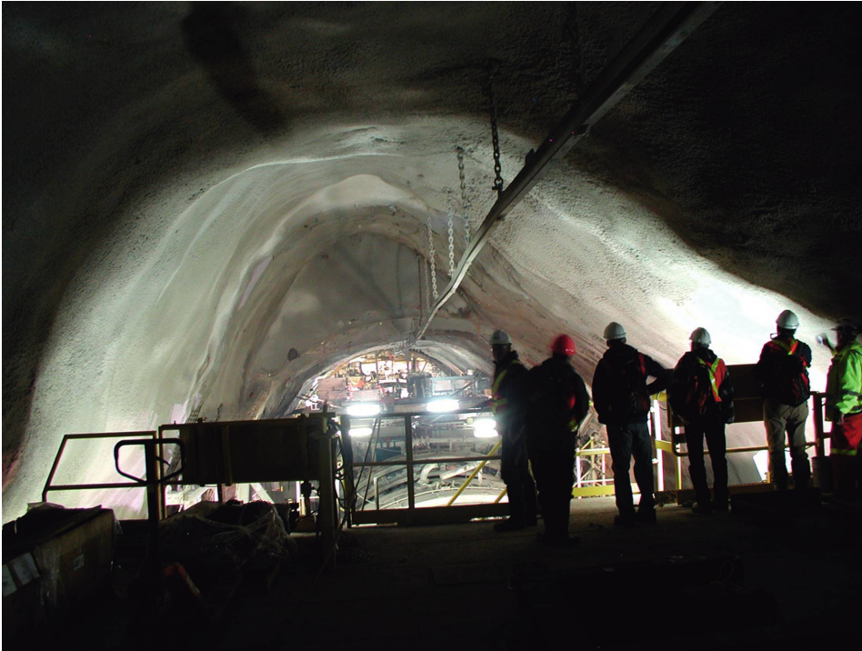
Figure 19.7 Significant oversteering of rock at 150 m depth.
