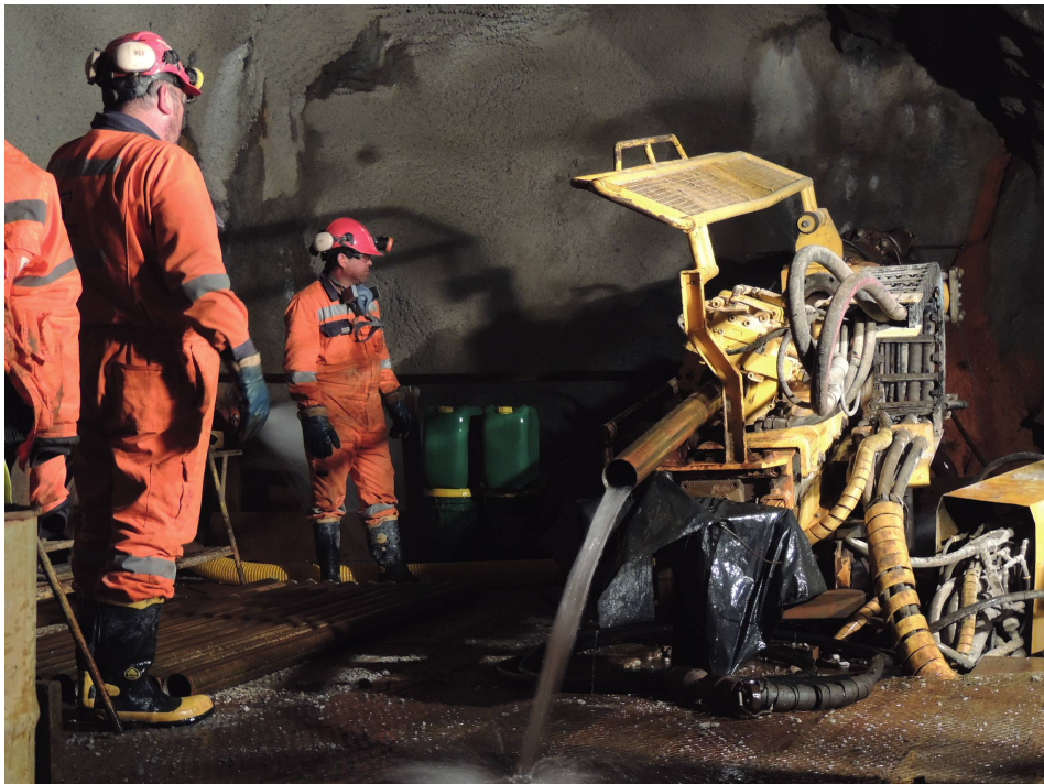
Figure 12.5 Groundwater drain holes at El Teniente.
