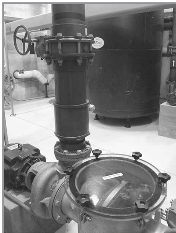
Figure 8.6 The filter room at an aquatic facility.
