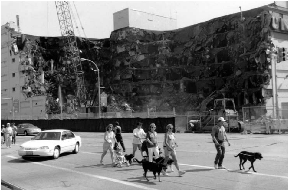
Pittsburgh: part of a parade of dogwalkers passing a demolition site – photo: Malcolm Miles
