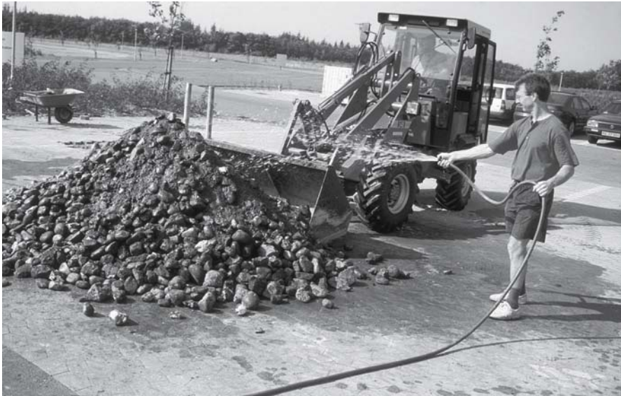
Fig. 11.7. Primixing of the soil and stone mixture before installation (photo: P. Kristoffersen)
