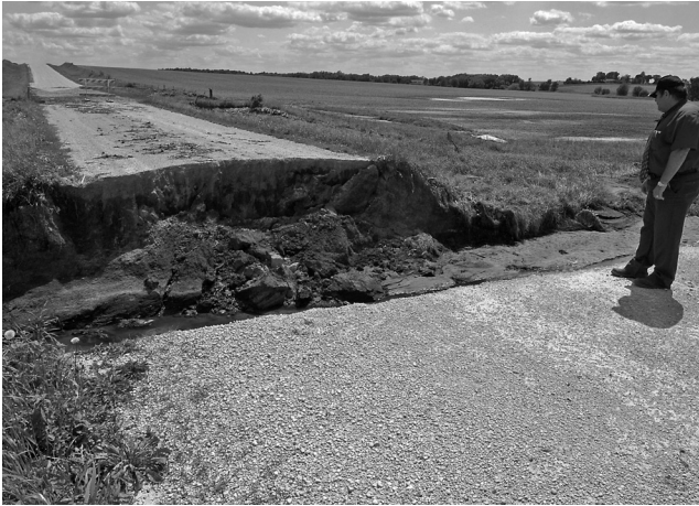
Figure 8.8 Localized infrastructure damage such as this washed out road can be reported and addressed far more quickly when crowdsourcing tools like Ushahidi are used to support and supplement traditional damage assessment teams. (From FEMA/Marvin Nauman. With permission.)
