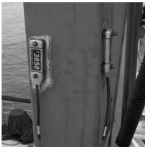
Figure 5. Pasted sensors of derrick's leg.
