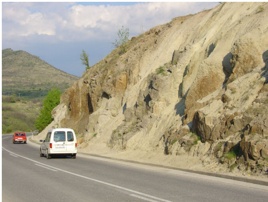
Fig. 15.13 Debris transported downslope of the road to Sv. Petka dam
