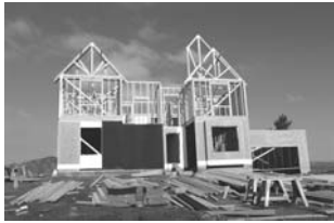
House Under Construction. Polymers are used extensively in the construction of modern houses
