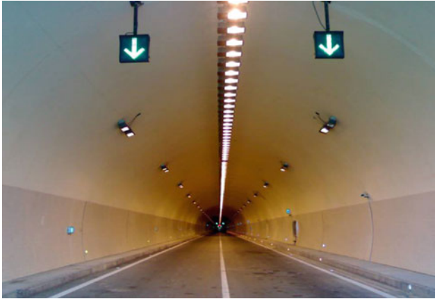
Fig. 1 The lighting environment of the experiment tunnel
