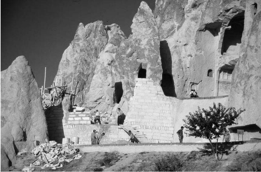
Plate 8.2 Erosion of the fairy chimneys: 'Disneyland tells us that technology can give us more reality than nature can' (Eco 1986: 44). Funding from the Turkish Ministry of Culture and UNESCO pays towards these efforts to strengthen and rebuild the fairy chimneys that house the best examples of Byzantine frescoes in the Göreme Open-Air Museum.
