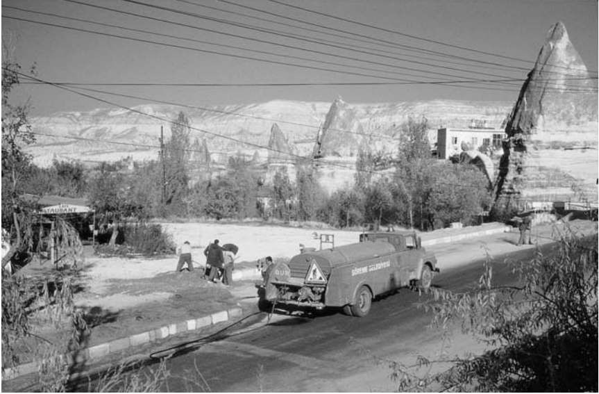
Plate 8.1 The National Park plan in action: municipality workers placing telephone and electric cables underground so that, in accordance with the Göreme National Park plan, wires and pylons do not obscure the 'natural' landscape.
