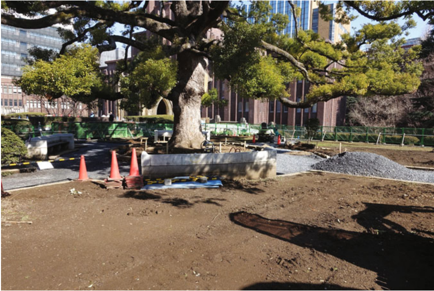
Fig. 13.4 The site condition of this old but robust Cinnamomum camphora is being rehabilitated by expanding the soil and root protection zone well beyond the drip line and improving the soil quality within the entire area. It can be appreciated in the Tokyo University campus (Photo credit C.Y. Jim)
