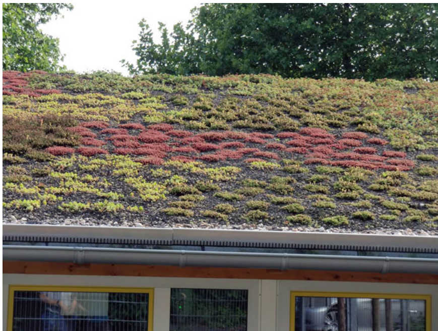
Fig. 11.3 A Sedum greenroof planted on the top of a one-storey kindergarten building in Bonn. This is an extensive type which requires a shallow substrate with limited water holding capacity to suit the drought-tolerant physiology of the succulent plant. It is light-weight, durable and does not demand frequent maintenance ( Photo credit Gwendolyn Wong )
