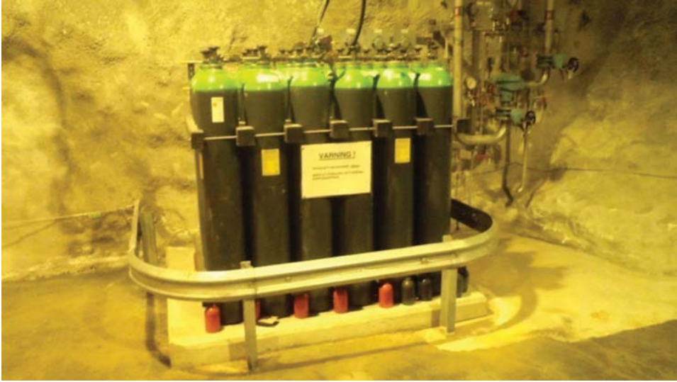
Plate 8.22 Chlorine stored at wastewater treatment plant site.
