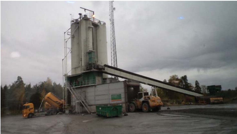
Figure 6.22 Ash stabilization and solidification unit.
