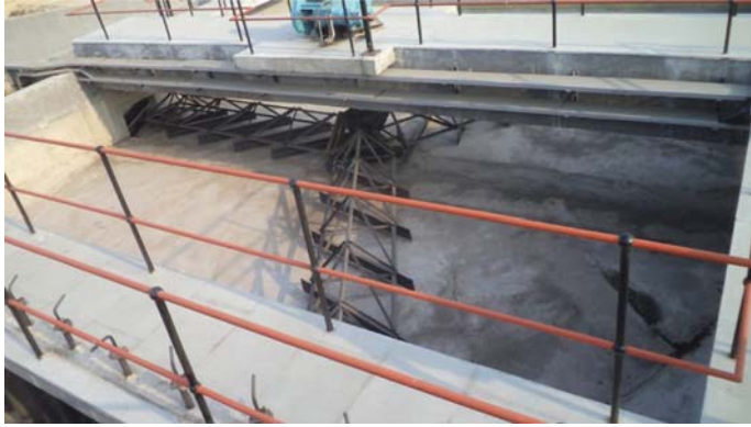
Figure 4.12 A grit-removal chamber with scrapper.
