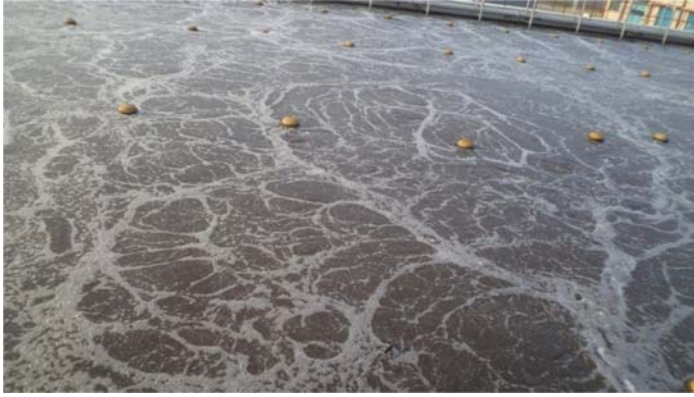
Figure 4.22 Aeration process with submerged aerators.
