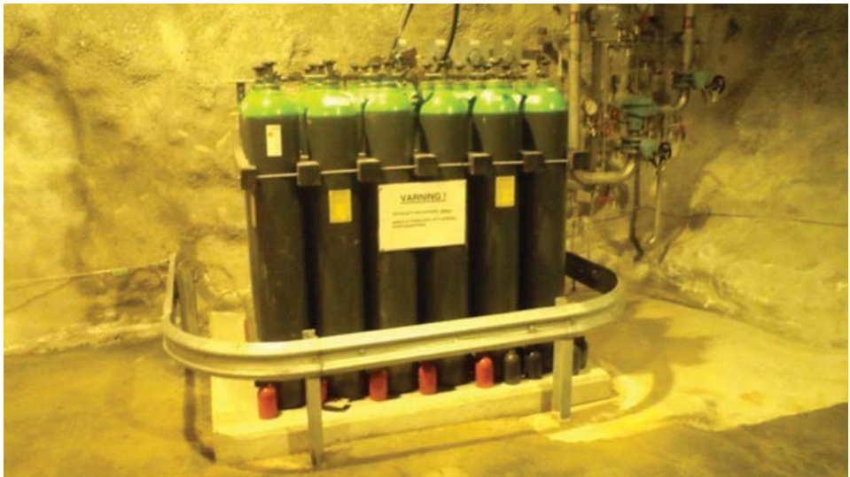
Figure 8.22 Chlorine stored at wastewater treatment plant site. (For a colour version of this figure, see the colour plate section.)
