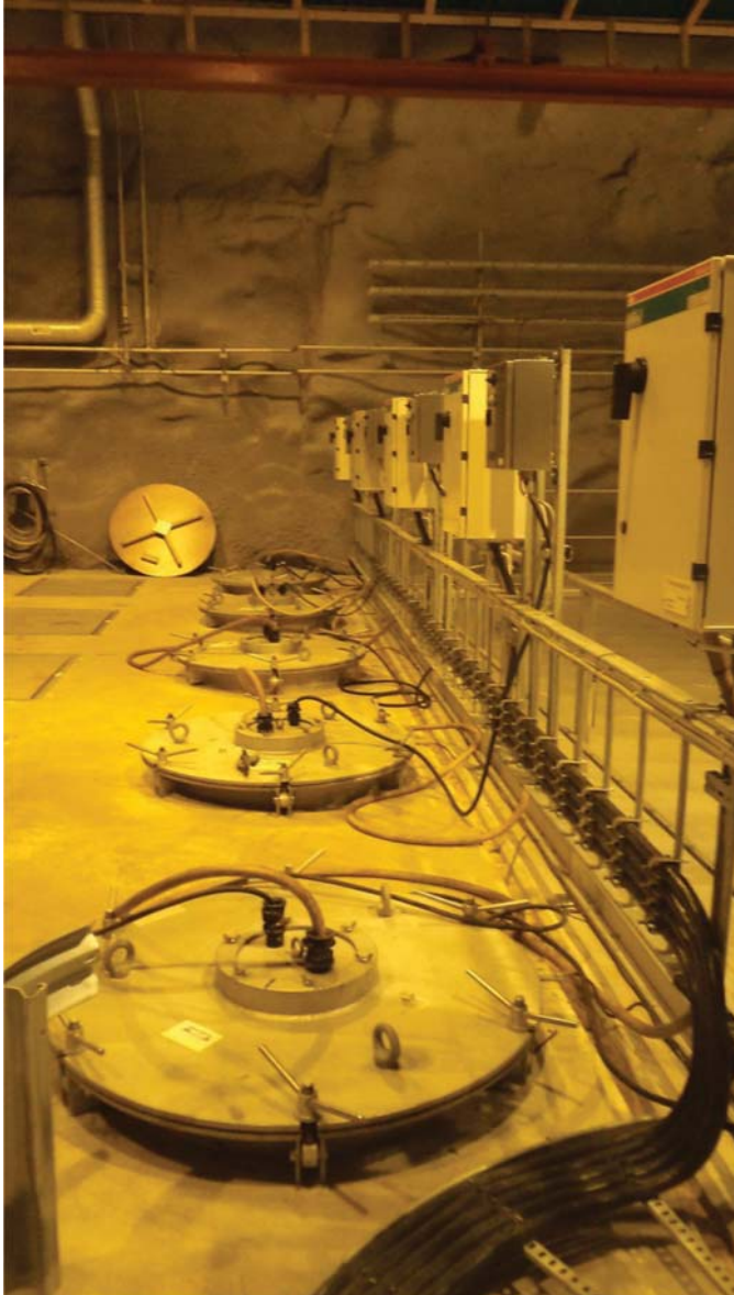
Figure 2.39 View of new-generation pumps in wastewater treatment plants.
