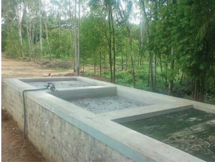
Figure 4.48 Sludge drying beds.
