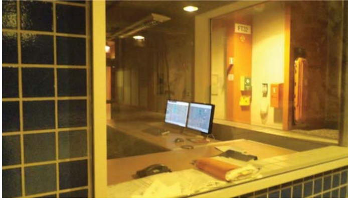
Figure 4.2 Control room of a large sewage treatment plant without process control engineers.
