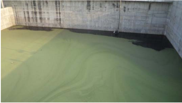
Figure 4.26 Treated effluent from ASP being further treated in anoxic tank to achieve denitrification.
