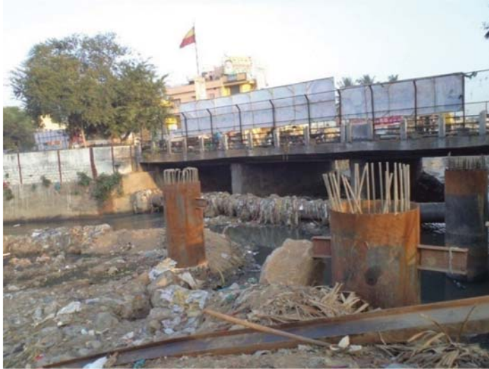
Figure 2.41 Poorly maintained open drainage.
