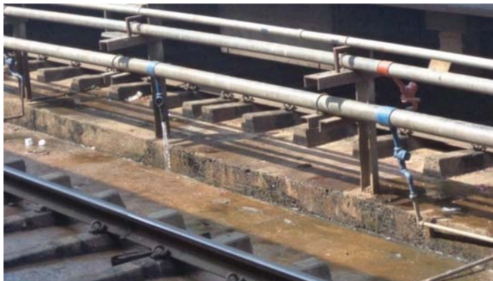
Figure 2.26 Water being wasted in one of the railway stations in India.
