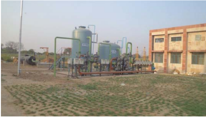
Figure 4.42 View of pressure sand filter and softener.
